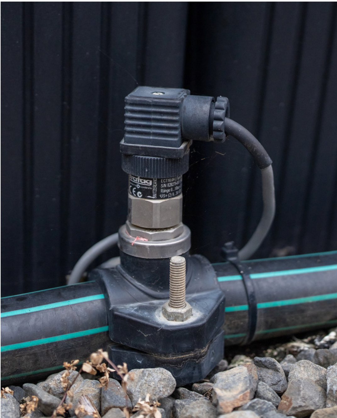
Figure 20. Irrigation pressure transducer installed on 40mm Polyethylene tube irrigation line at a production nursery.
