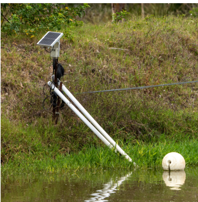
Figure 27. Dam monitoring system with buoy to keep sensors at a constant depth.
