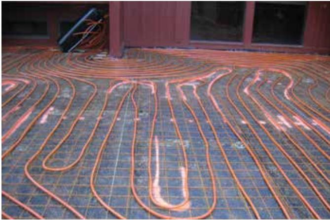
Figure 6. Radiant heating can be installed under the paver surface to melt snow and ice in the winter.
