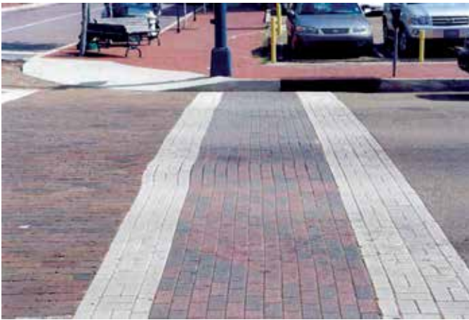
Figure 23. Horizontal Creep is easily spotted in ICP areas that were constructed straight, but over time develop a wave in the pattern.
