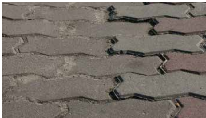
Figure 21. Faulting can be seen as a line of pavers being lifted above the neighboring units.
