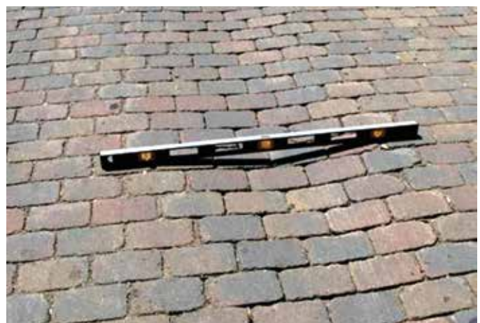
Figure 27. Rutting occurs when the underlying layers settle. The extent of rutting is easily measured by laying a straight edge across the rut.
