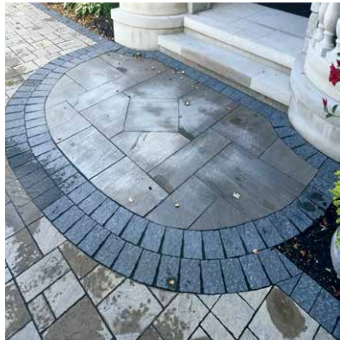
Figure 9. Efflorescence is only an aesthetic concern and can be removed with cleaners specifically formulated for this task.
