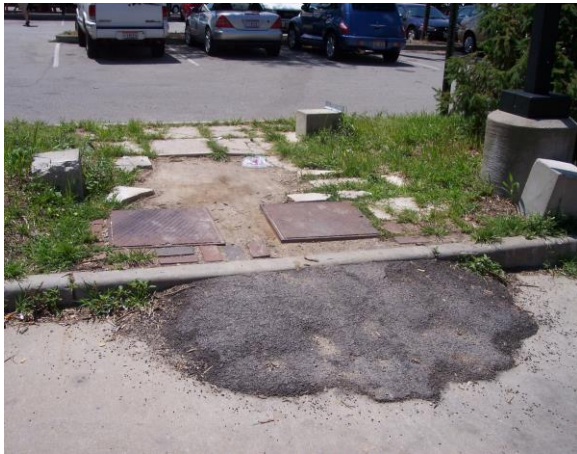
Is this safe for your customer walk-way into the market? Who will be responsible for repairs? Who will be responsible should some be hurt?
