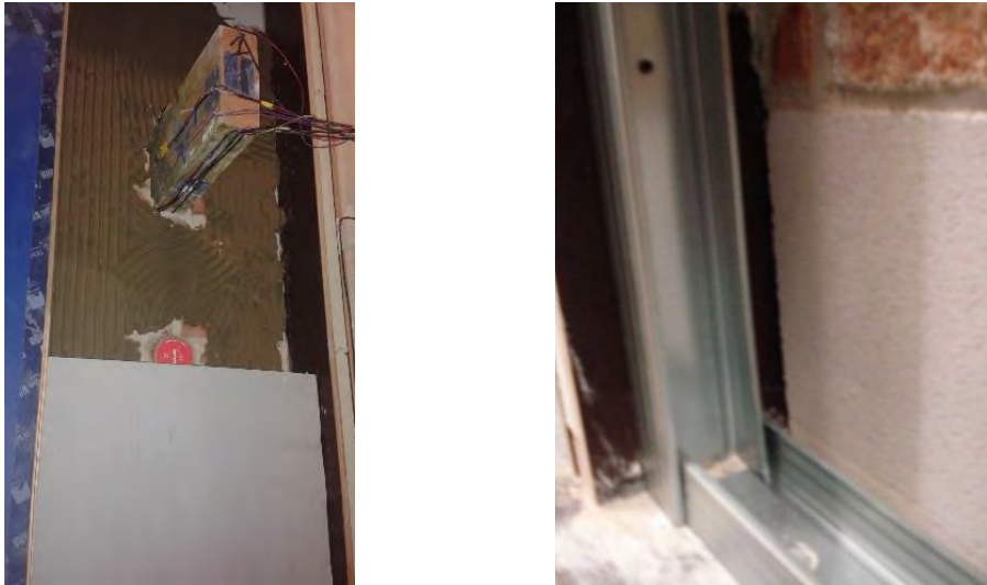
Fig. 86.: Left: calcium silicate boards fully adhered to the wall. Right: The metal studs in the mineral wool system were positioned 4 cm in front of the masonry wall to avoid thermal bridges.
