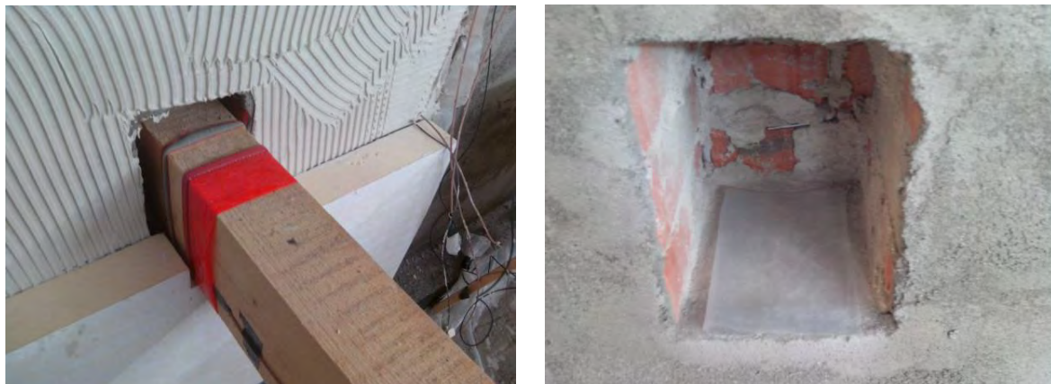
Fig. 8.: Double layer of pre-compressed sealing tape around the joist end prior mounting of the insulation boards (left) and PE-foil in the masonry block-out for the joist end (right), both in the first test strip of the test wall (iQ-Therm).
