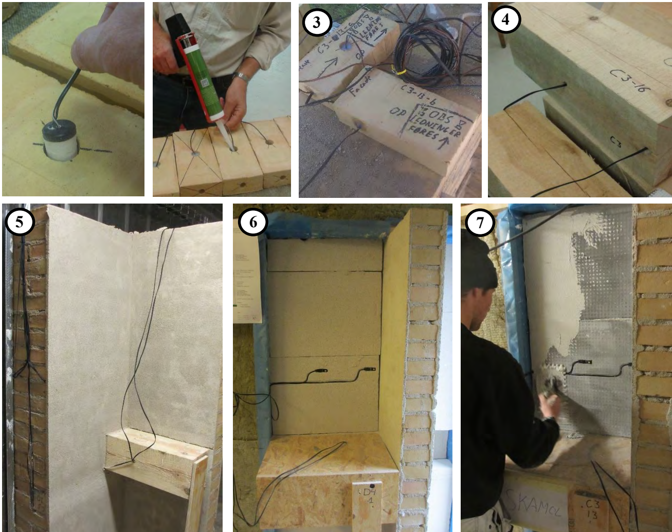
Fig. 59.: Sensor installation. 1) Sensors installation in masonry brick. 2) Filling cavity around the sensors with silicone. 3) Sensors at location 1 and 2 being installed in the masonry assembly. 4) Sensors at location 6 and 7 in the wooden beam. 5) Reference wall with all the sensors installed. 6) Installation of sensors 4 and 9 in recesses in the Xella Multipor boards. 7) Covering up sensors 4 and 9 in Skamoplus boards with the interior finishing.
