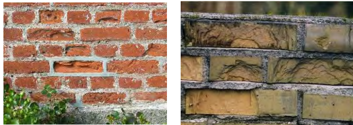
Figure 4-14: Example of scaling due to frost in masonry
