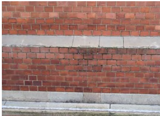
Figure 4–35: Brick façade with a distinct frieze which has collected water leading to joint and frost damage.
