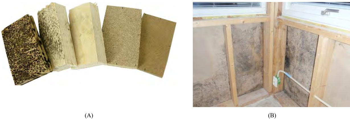
Figure 4–11: (A) Illustration of how the visible impression of mould growth varies. All samples shown have the same extent of mould growth, although the growth is not visible to the naked eye in all cases. (B) Example on how mould growth may be hidden within the building structure. In this example, interior surface materials and insulation was removed before mould growth was detected.
