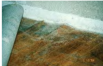
Figure 4–9: Examples of visually apparent induced damage of internal façades
