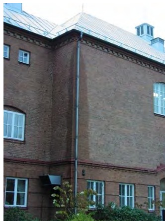
Figure 4–37: A clear sign on a blocked water collection system. Water that cannot be transported through the vertical pipe is absorbed to the bricks (the darker areas around the vertical pipe).
