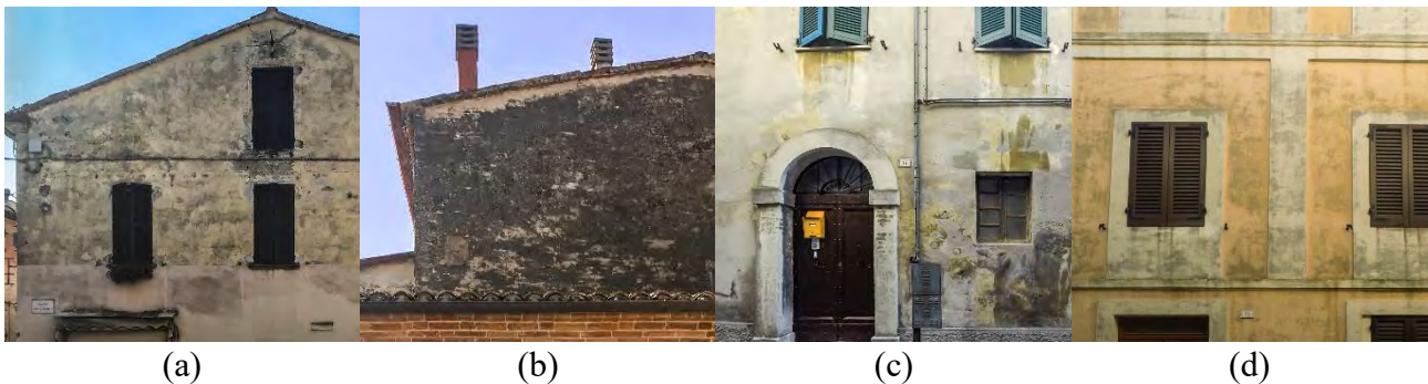
Figure 4–15: Examples of algae growth on external walls: a) and b) façades exposed to wind driven rain; c) and d) fed by drain water from windows overhangs.
