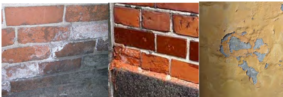
Figure 4–19: Examples of rising damp and damages caused by moisture in the walls; left: darkening of masonry and salt efflorescence, middle: frost damage in masonry, right: peeling of paint due to moisture accumulation and too diffusion tight paint (Source: Morten Hjørlev Hansen).
