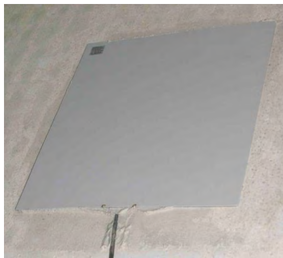
Figure 4–50: Example of a heat flow meter sensor applied to the wall surface
