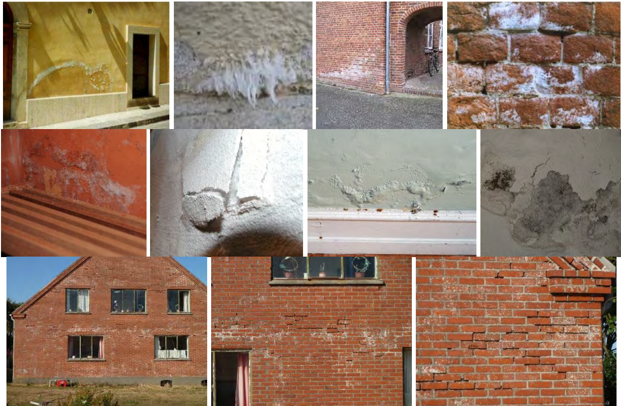
Figure 4–17: Examples of salt efflorescence in masonry walls; top row: externally, middle row: internally, bottom row: façade with salt attack.
