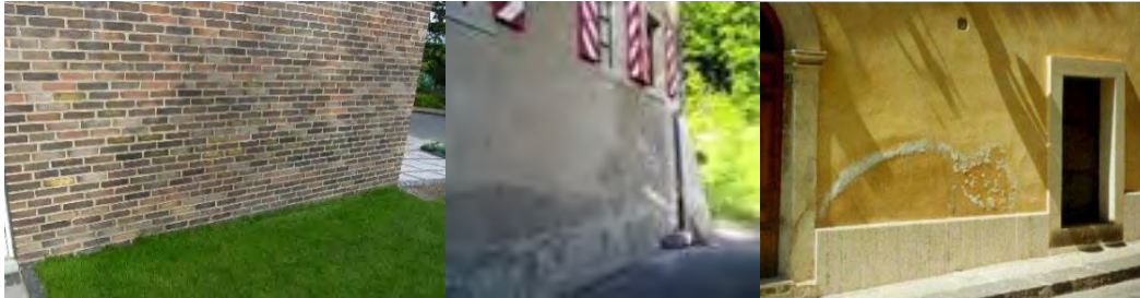
Figure 4–18: Examples of rising damp in external masonry, appears as darkened/moist areas (Left and center), and an example also showing salt efflorescence (right). Source (center): CSC Sárl https://conservation-science.ch/
