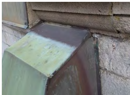
Figure 4–36: Frieze with steel cladding. Water can be transported behind the steel plate, be absorbed and lead to frost damage.
