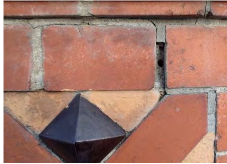
Figure 4–34: Example of frieze on a brick façade with extensive damaged joints.
