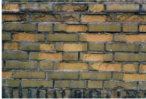
Figure 4–32: Frost damage in outer layers of historic masonry
