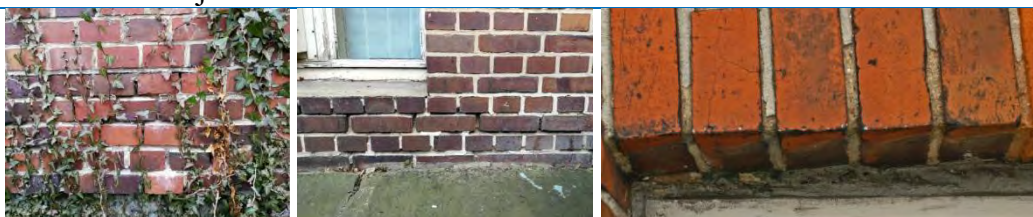
Figure 4-7: Examples of visually apparent moisture induced damage of external façades
