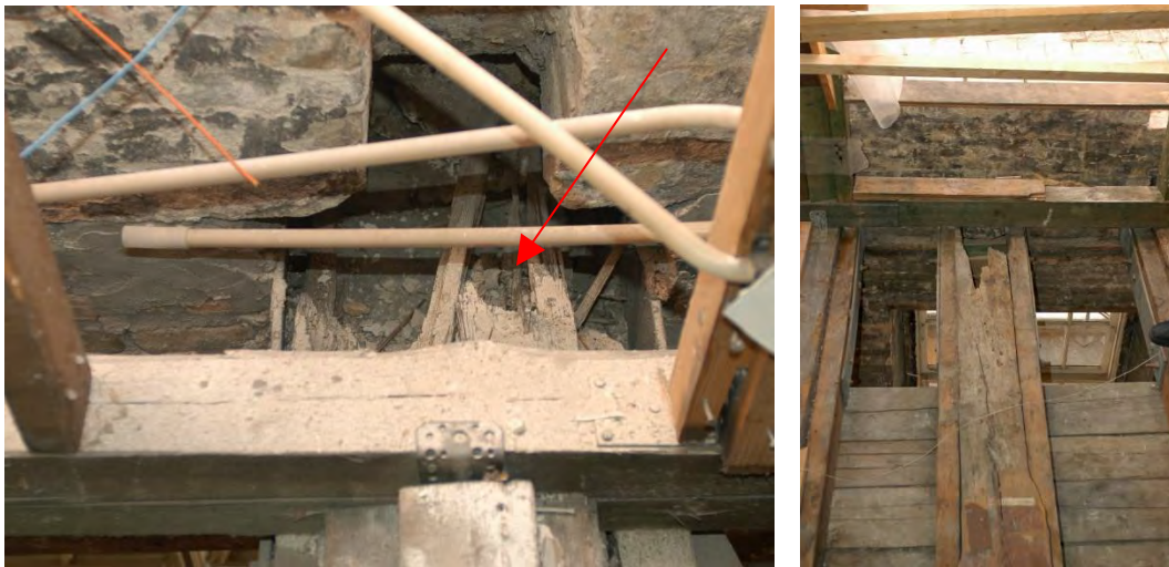
Figure 4–12: Example of wood decay in a storey partitioning beam (L), and rot fungi attack on beam near the roof (R).
