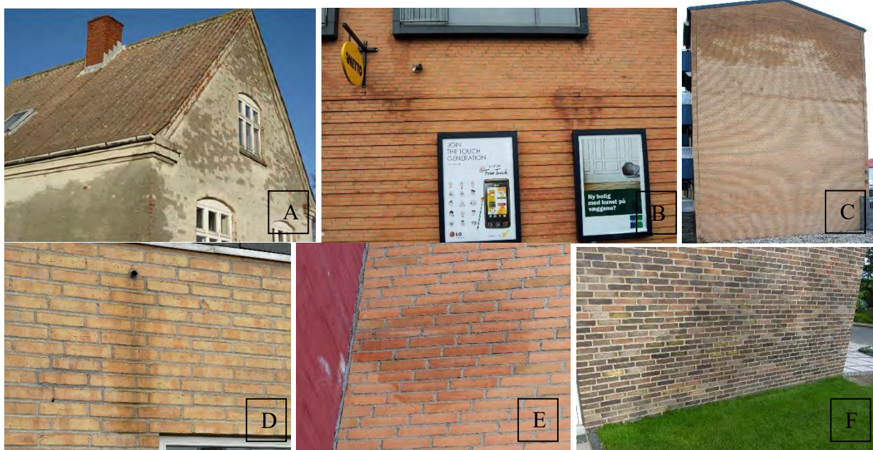
Figure 4–6: Examples of stains and wet spots. A: moist areas on rendered masonry façade, B: wet spots on masonry façade, C: moisture accumulation at top of façade gable, likely due to precipitation, D+E: local defects causing concentrated moisture accumulation, F: moisture accumulation near the plinth, likely due to rising damp
