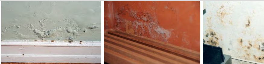
Figure 4–8: Examples of visually apparent moisture and moisture induced damage of internal façades.
