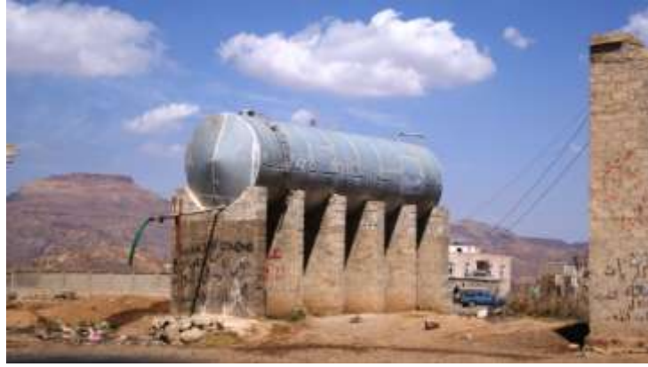
Photo 1.1: A storage tank located near by the well
