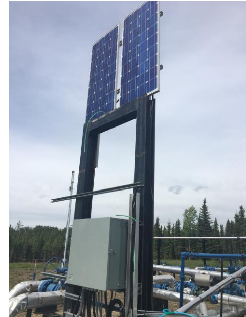
Spartan Delta wellsite solar power generation
