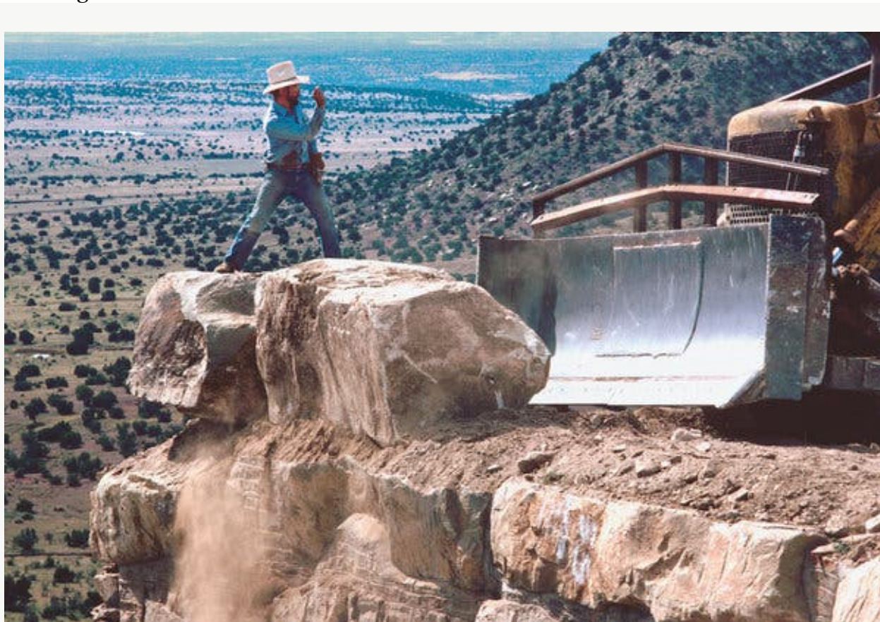
Ross on a boulder during the construction of "Star Axis" in 1982. Credit...Elizabeth Ginsberg
