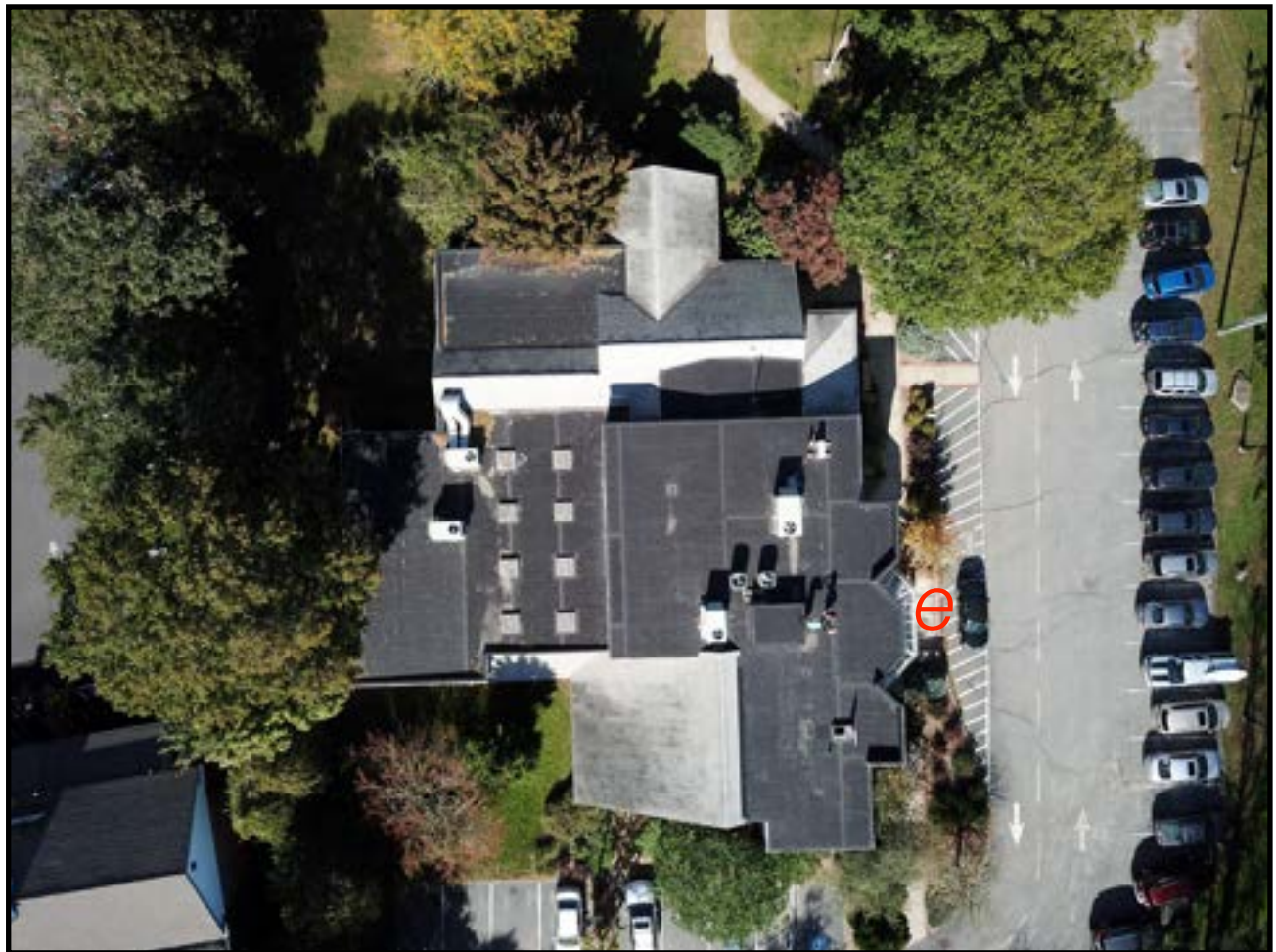
Rooftop view. Black areas are flat membrane roofing. Gray areas are sloping asphalt shingle.
