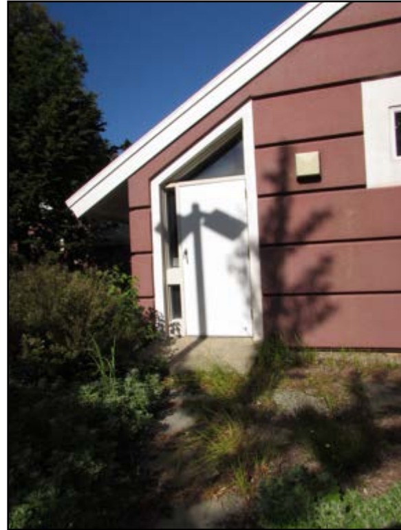
Meeting Room emergency egress door. Note sloping landing.
