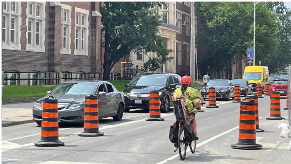
Image 3: Cyclist heading west toward Spadina Road. There appeared to be a makeshift sidewalk, though not indicated by signage, between these construction cones and a fence that delineated the construction zone. The narrow passage was taken by many westbound cyclists as a way to avoid motor traffic, but this put those cyclists in potential conflict with pedestrians walking east or west. The actual sidewalk was closed. (Photo: Albert Koehl)
