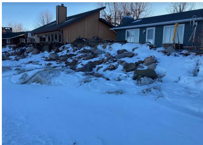
Photo 6: Ice heaves causing uplift of bank
