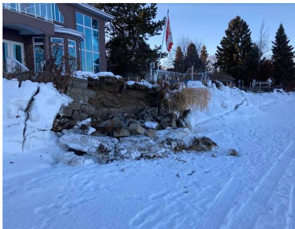
Photo 2: Damage to shoreline retaining wall
