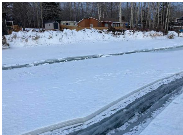
Photo 5: Ice jacking caused by expansion/contraction of ice. Contraction fractures are shown.
