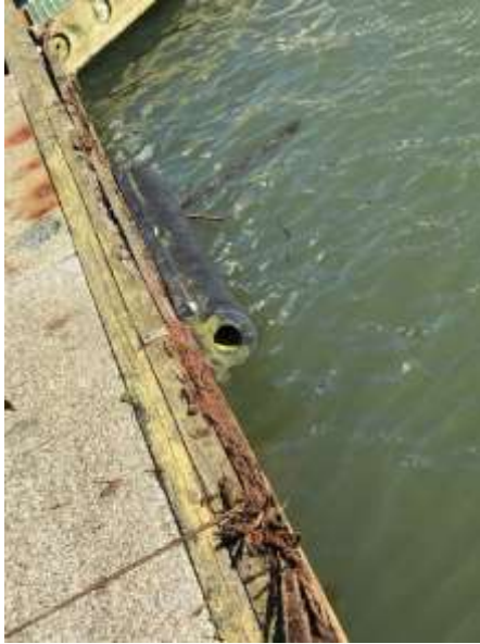
Figure 4-6: Deteriorated Fender Systems
