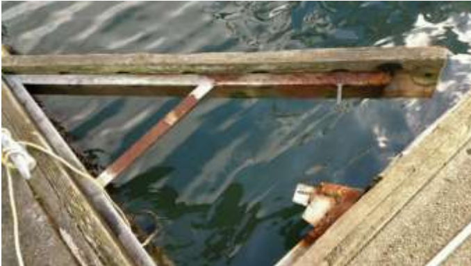
Figure 4-4: Broken Mooring Braces
