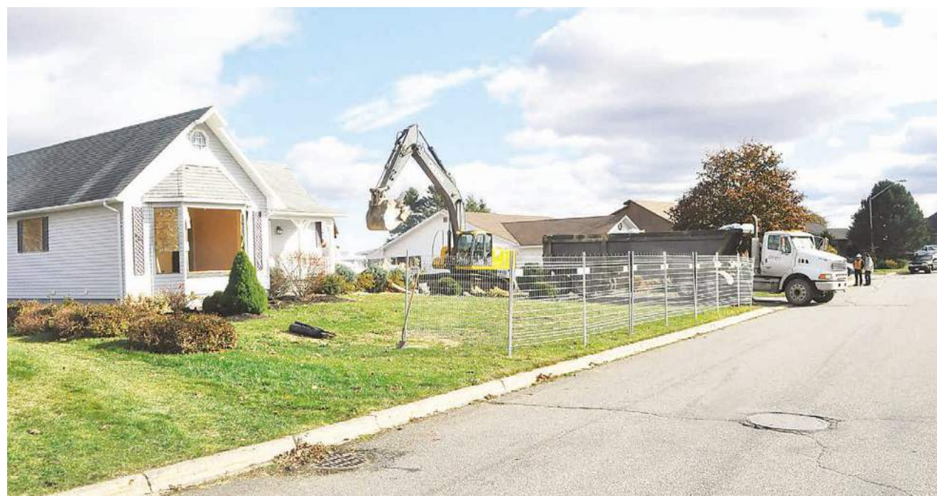
Work began on Thursday to demolish 13 homes on Ocean Ridge Drive in Bathurst. PHOTO: JAMES MALLORY/THE NORTHERN LIGHT
