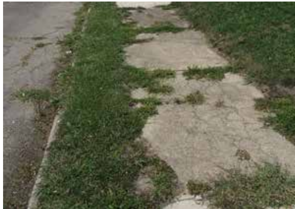
Figure 3 – Poor sidewalk conditions. Photo: Martin.
