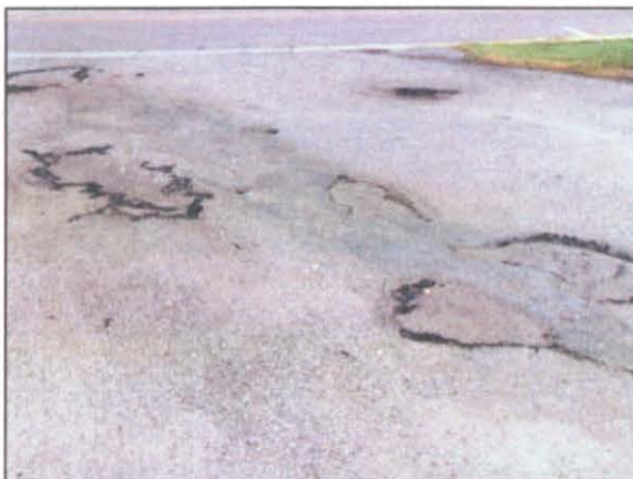
On-site street surfaces in need of repair are the most common site problems in the Survey Area.
