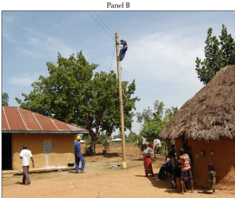
Fig. 5.4 Example of a REA design drawing and the electrification of a treatment household Notes: After receiving payment, REA designers visited each treatment community to design the local low-voltage network. The designs were then used to estimate the required materials and determine a budgeted estimates of the total construction cost. Materials (e.g., poles, electricity line, service cables) represented 65.9% of total installation costs. Reprinted from Lee et al. (2020a)
