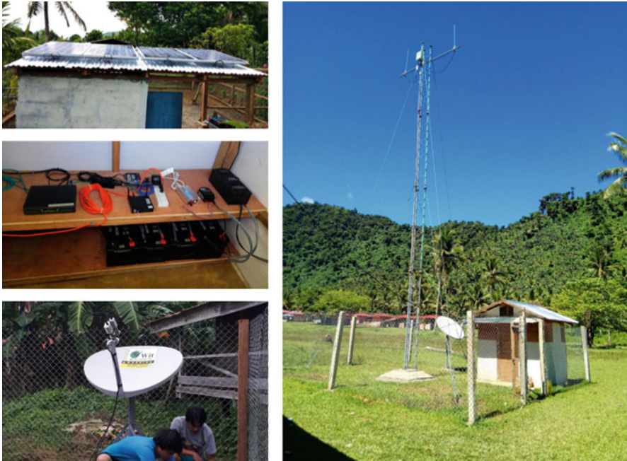
Fig. 21.1 A typical installation of a community cellular network cell site piloted in the Philippines
