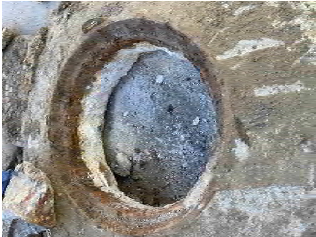
Photo 3-12 Manhole Ring and Cover Debris
