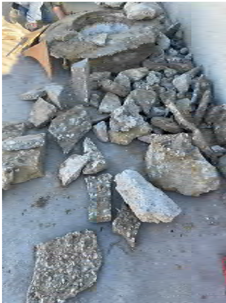
Photo 3-8 Pile of Debris from Collapse Site
