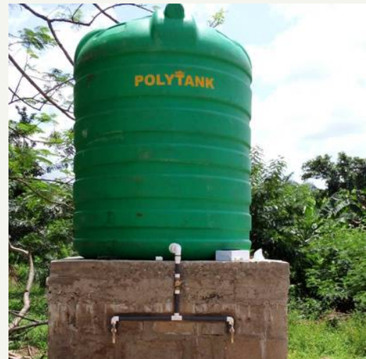
Borehole and water tank built by the Asunafo cooperative. Credit: Adom Cocoa
