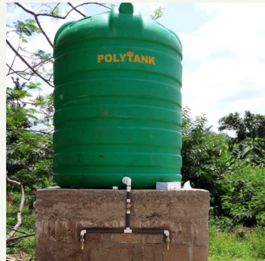
Borehole and water tank built by the Asunafo cooperative. Credit: Adom Cocoa
