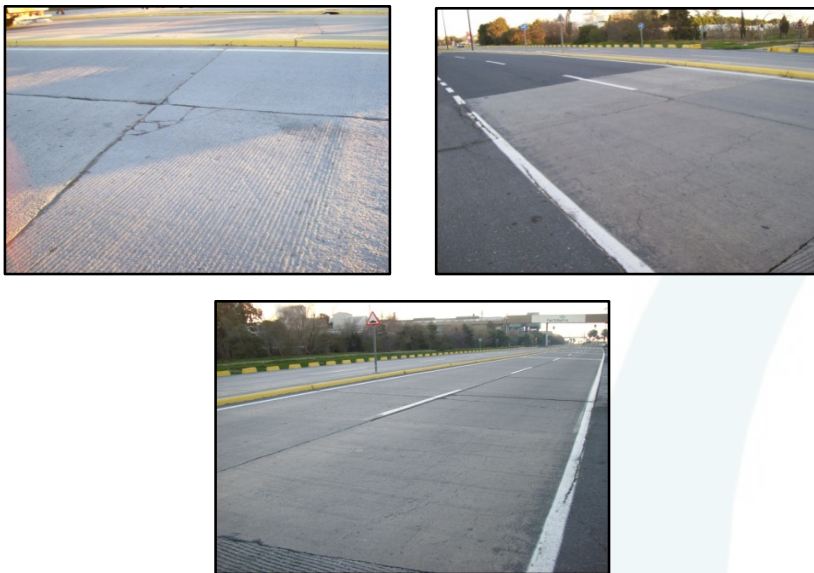
Deteriorated pavement in Huelva
