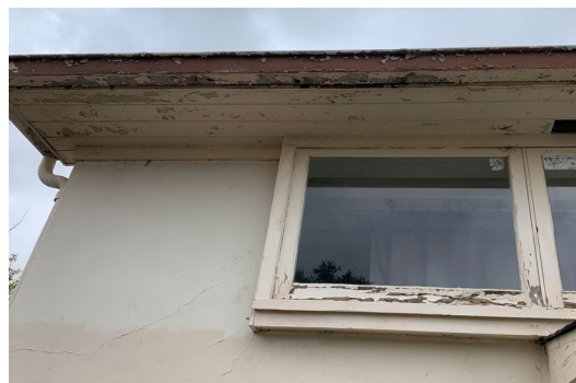
Deteriorating Building Exterior
