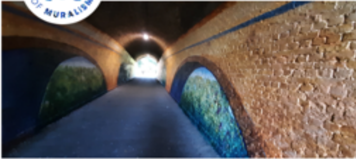
The arches also helped provide some rhythm as pedestrians walk along the tunnel, dividing the long length of it to make it more entertaining.
