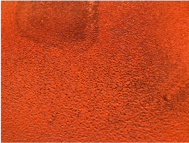
Image 3: Surface appearance of a flame coated HDPE pipe.
