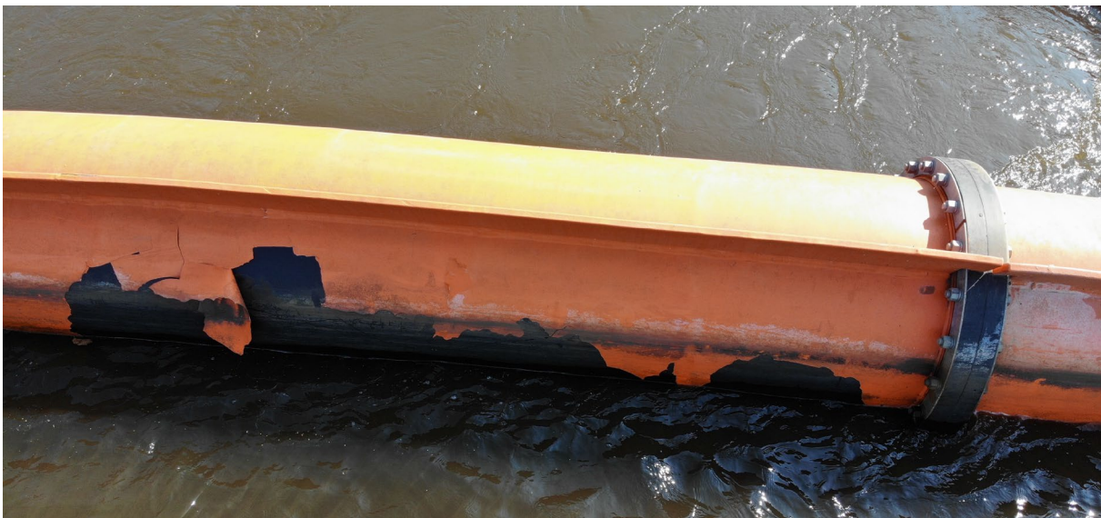
Image 1: Painted HDPE pipe shown 14-months after installation at a hydroelectric plant on the Mississippi river near Lower Saint Anthony Falls, MN (USA).
