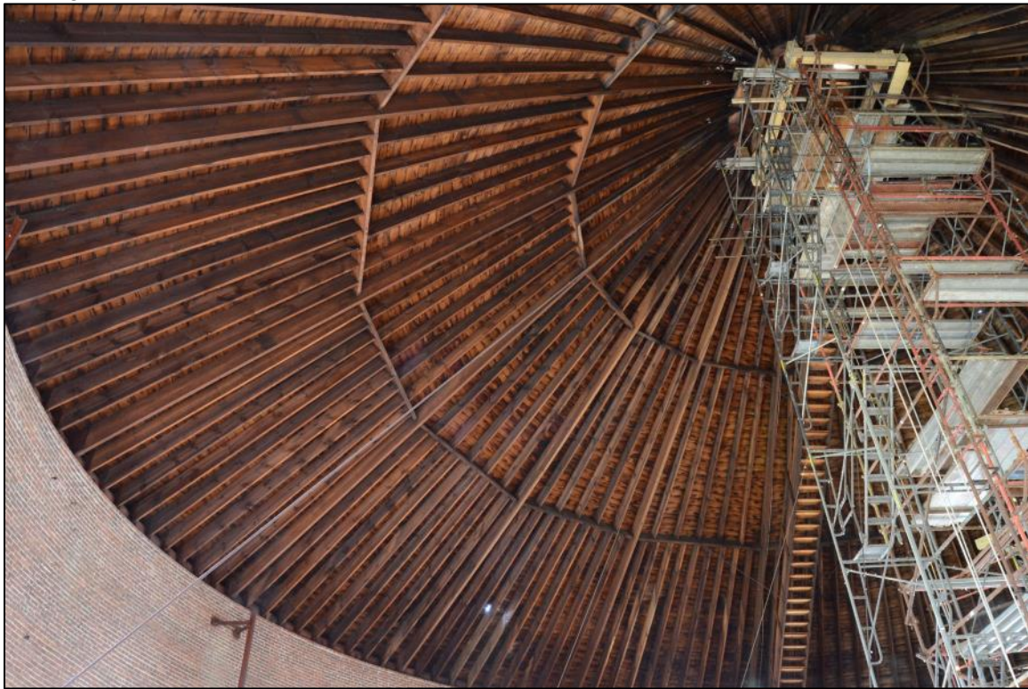
Photo 11. Ceiling framing of Gasholder House with cupola opening (obscured by scaffolding) at top right.
