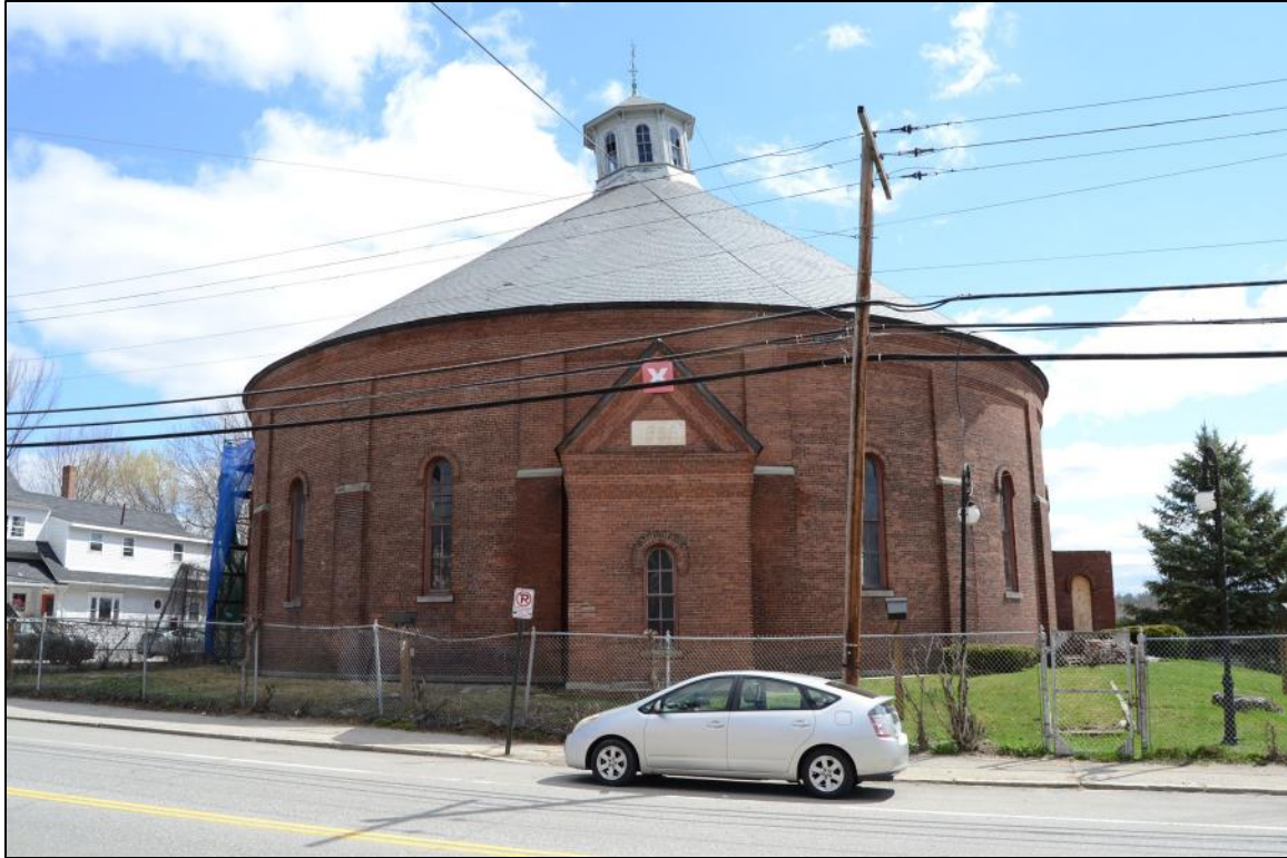
Photo 5. West side of Gasholder House and west valve house, looking east from South Main Street.
