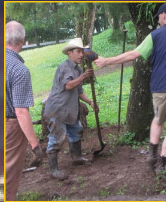
The yard crew pulling poles out of mountain clay by hand. The man with the shovel is 70 and outworked everyone.
