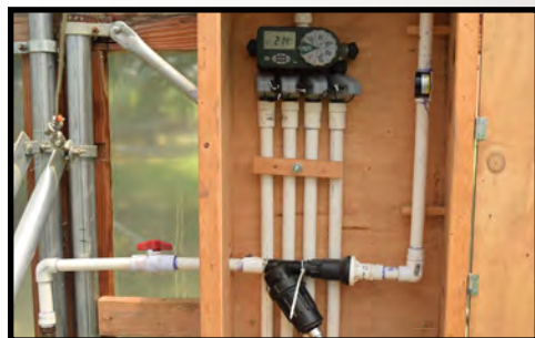
Irrigation manifold with timer at Griggs Bros. Farms.
