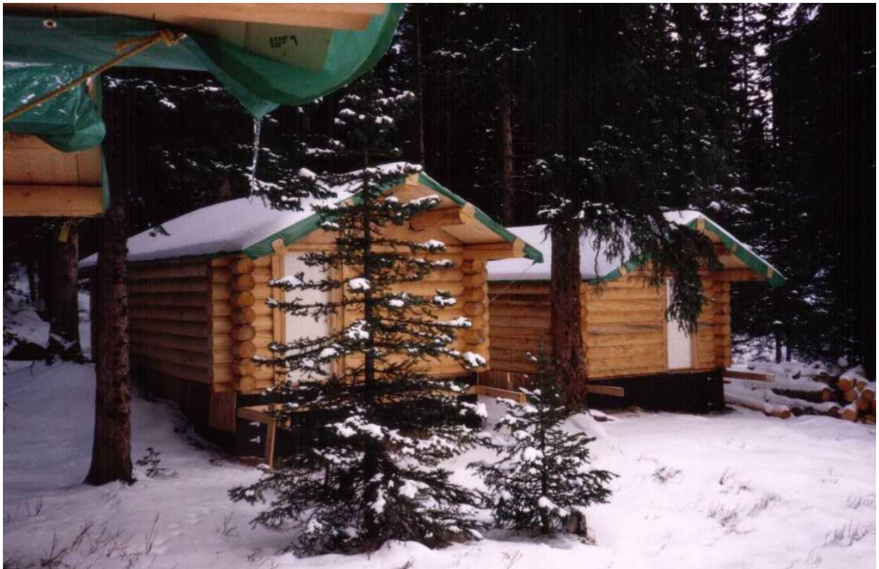
The partly completed cabins were covered in tarps for the winter of 1990/91.
