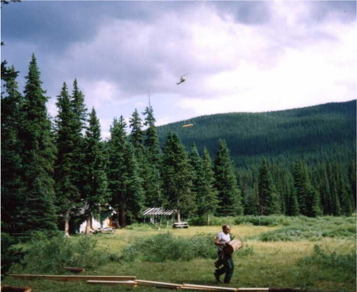
A helicopter slings in a log during the summer of 1990, when the new cabins were built.
