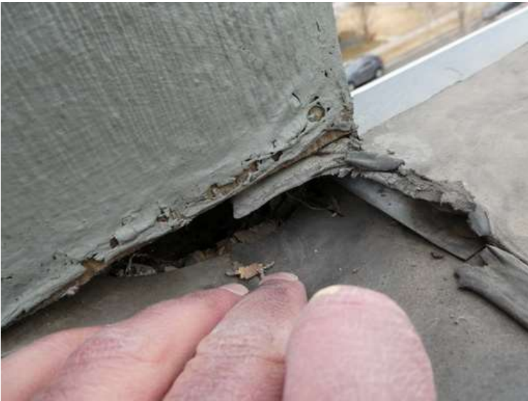
91. Building 03. Opening where water could leak past the roof.
