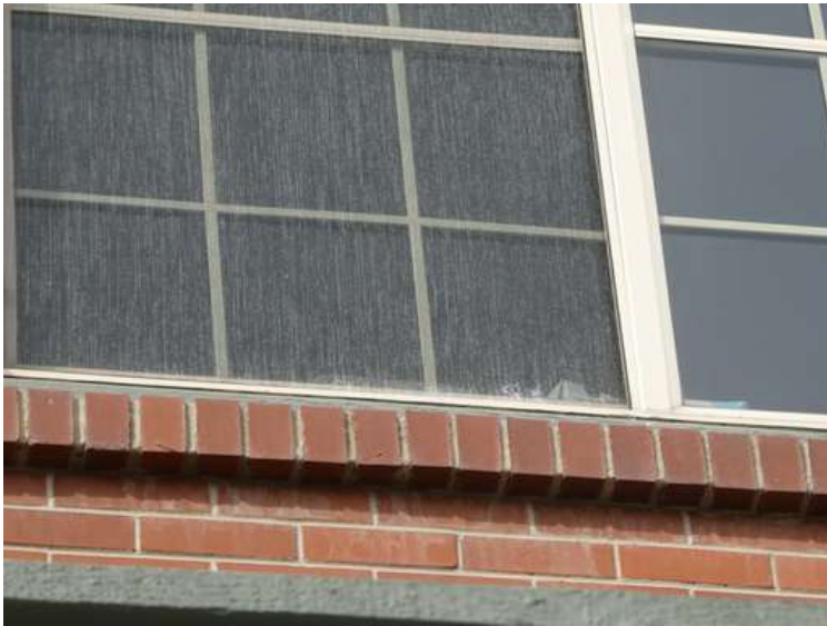
313. Building 14. Tears in a screen from hail.
