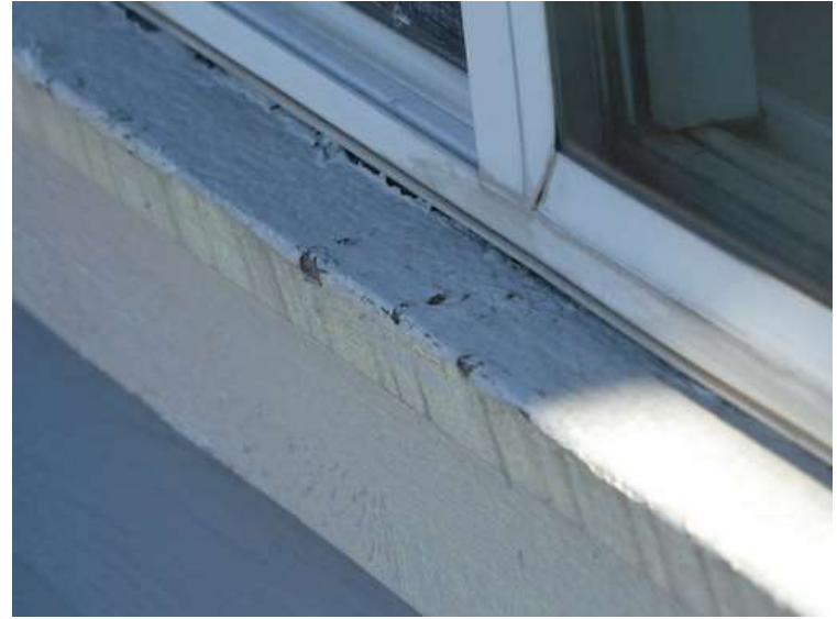
586. Building 24. Chips in paint from hail.
