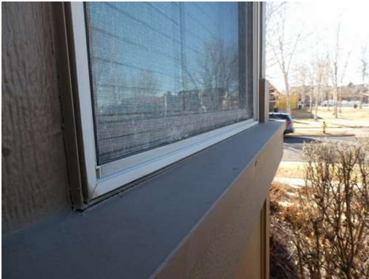
635. Building 26. Tears in a screen.
