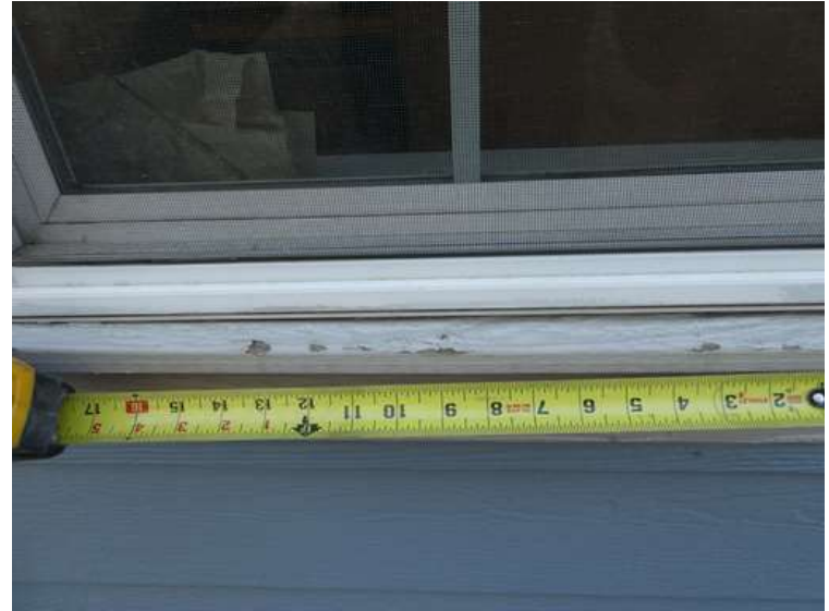
216. Building 09. Chips in paint on a sill.
