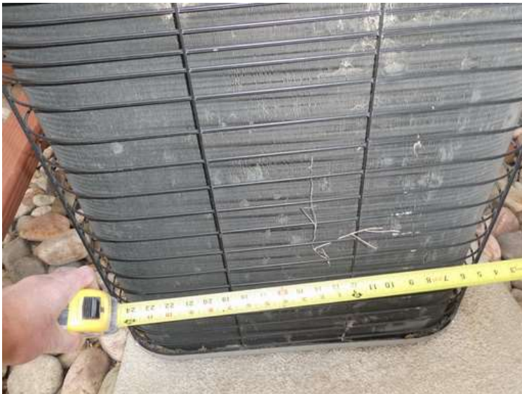
343. Building 15. Condenser fins dented by hail.
