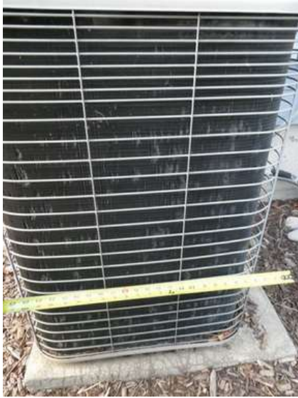
517. Building 22. Dents in condenser fins from hail.
