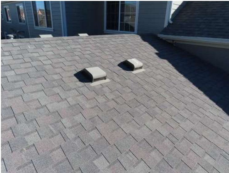
391. Building 17. West test area. No shingles within the test area were bruised by hail.
