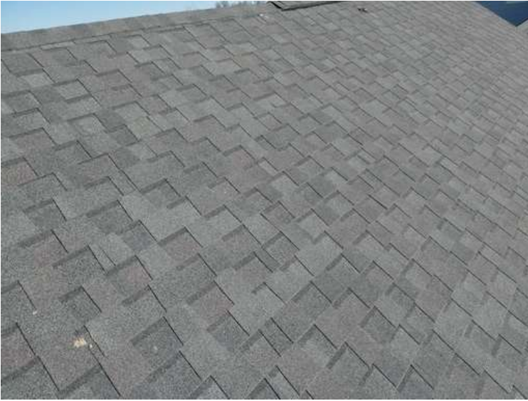
209. Building 08. West test area. No shingles within the test area were bruised by hail.
