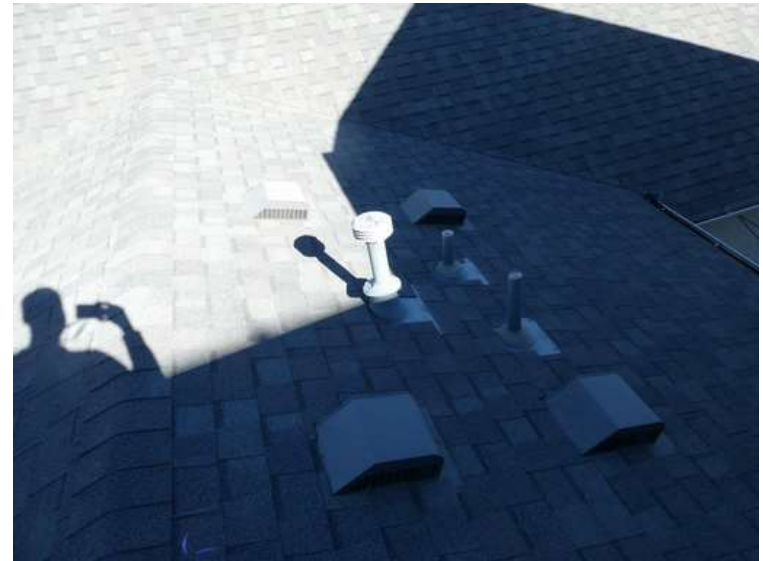
492. Building 21. East test area. No shingles within the test area were bruised by hail.
