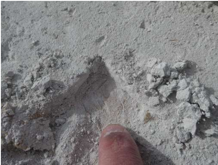
333. Building 14. The roof consisted of an OSB or plywood deck, gypsum board, and the adhered membrane.
