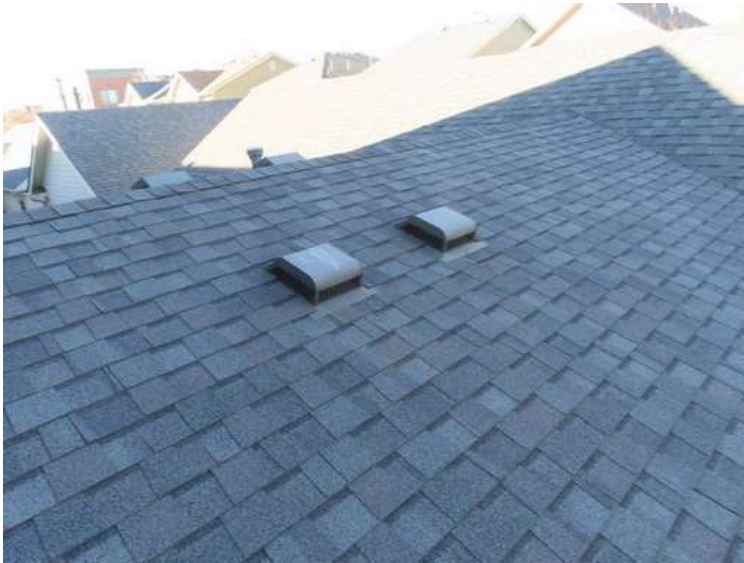
415. Building 18. East test area. No shingles within the test area were bruised by hail.
