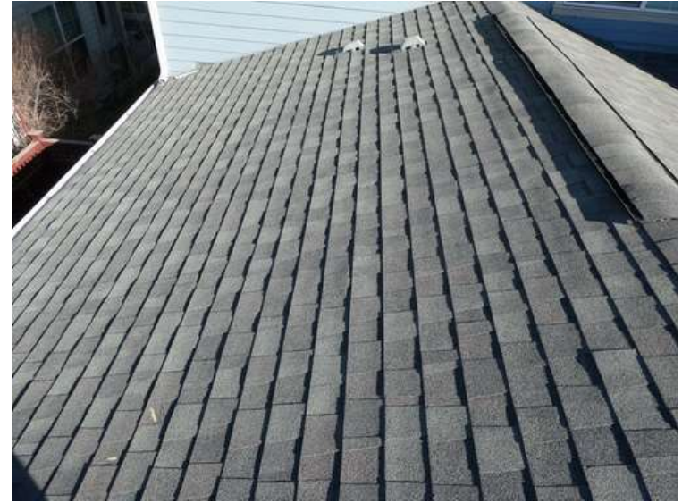
226. Building 09. North test area. No shingles within the test area were bruised by hail.
