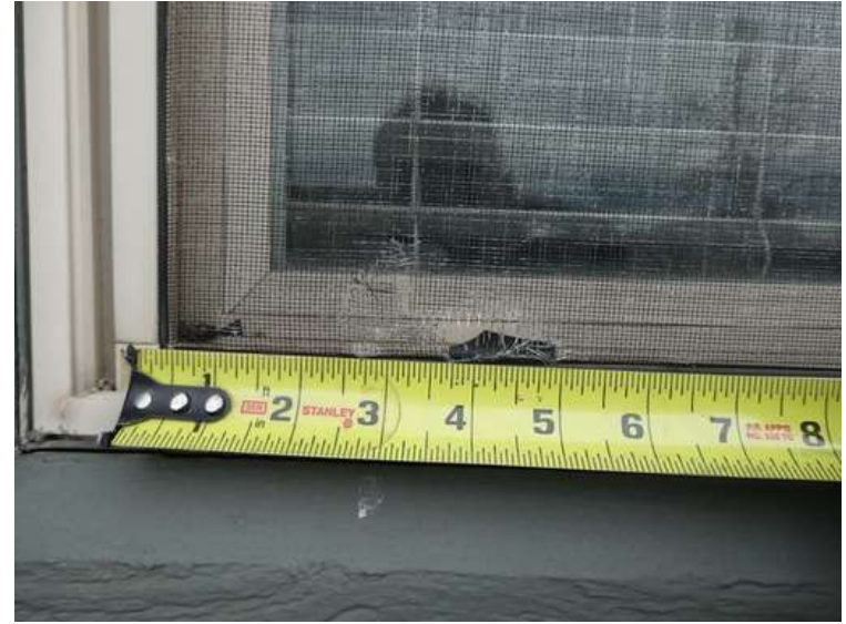
362. Building 16. Tears in a screen from hail.
