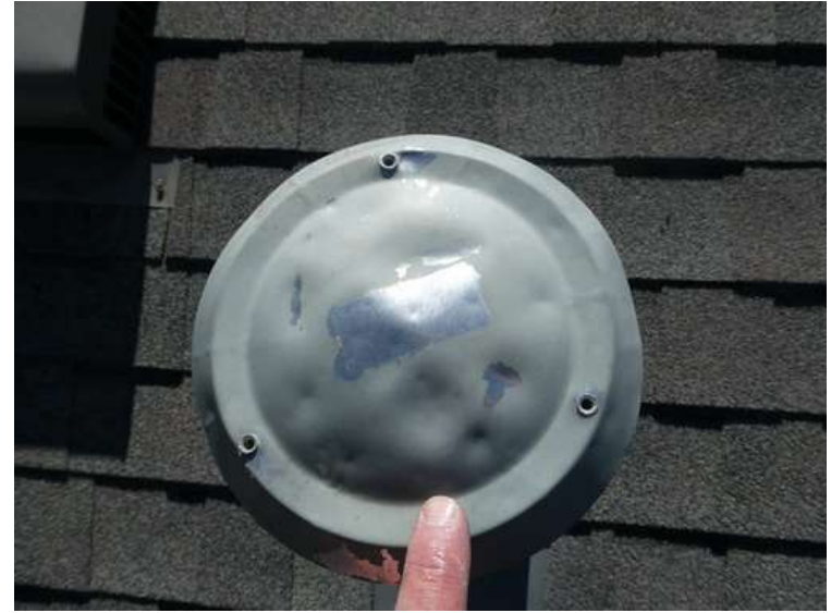
590. Building 24. Dents from hail.
