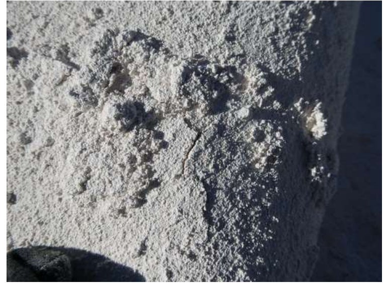
658. Building 26. Tear in the facer sheet from hail.
