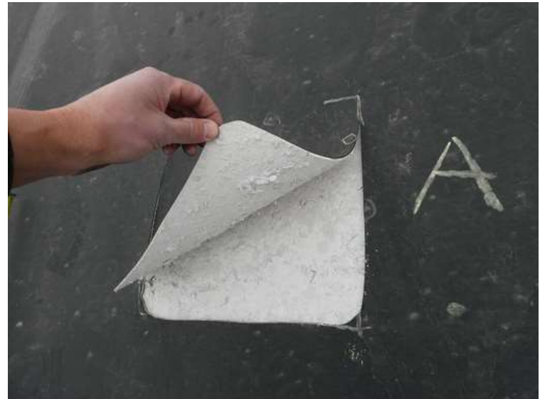
24. Building 01. Sample after cutting. The substrate provided little resistance to uplift.
