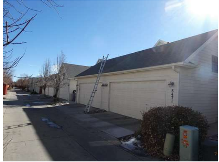
486. Building 21. North elevation. Garage doors were not dented by hail.
