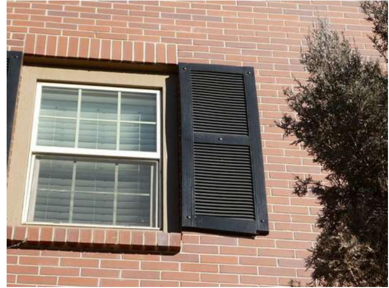
630. Building 26. Fractured shutter.
