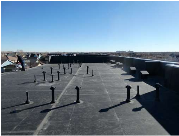
641. Building 26. View looking east. The roof was covered with an adhered EPDM membrane.
