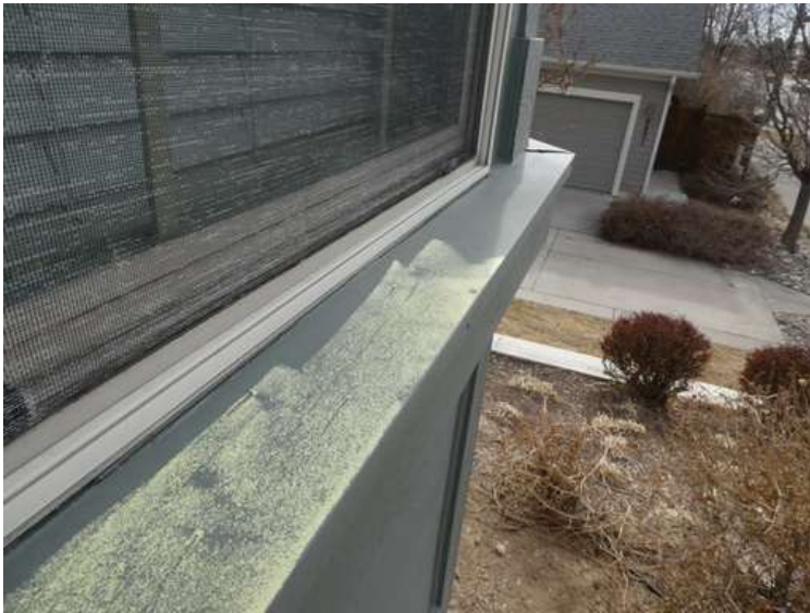
363. Building 16. Dents in steel flashing from hail.
