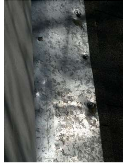
534. Building 22. Dent in headwall flashing.
