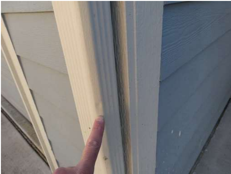
511. Building 22. Mechanical dent in a downspout.
