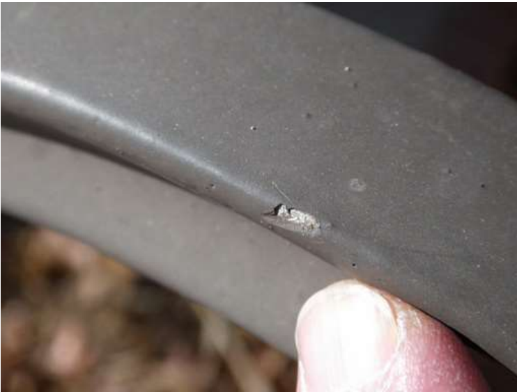
539. Building 23. Mechanical chip in paint on an iron fence.
