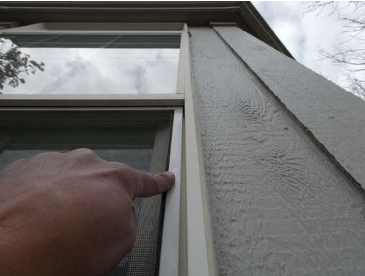
123. Building 05. Dent in a screen frame.
