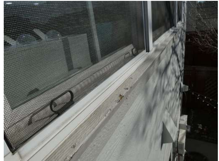
198. Building 08. Chips in paint.
