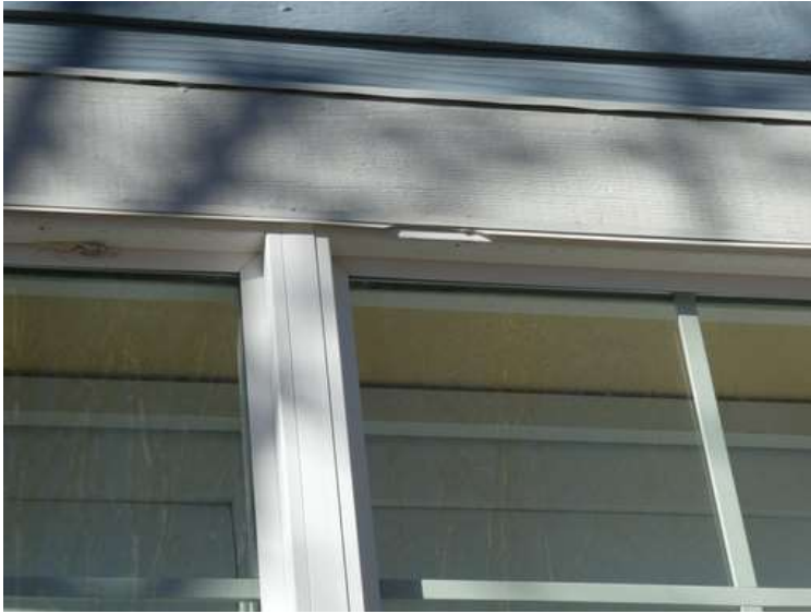
509. Building 22. Fracture in a plastic window frame from hail.
