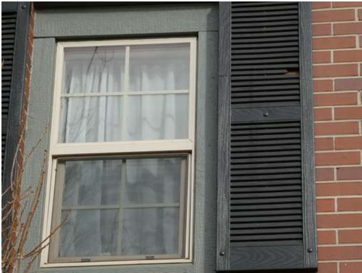
315. Building 14. Fractures in a shutter from hail.
