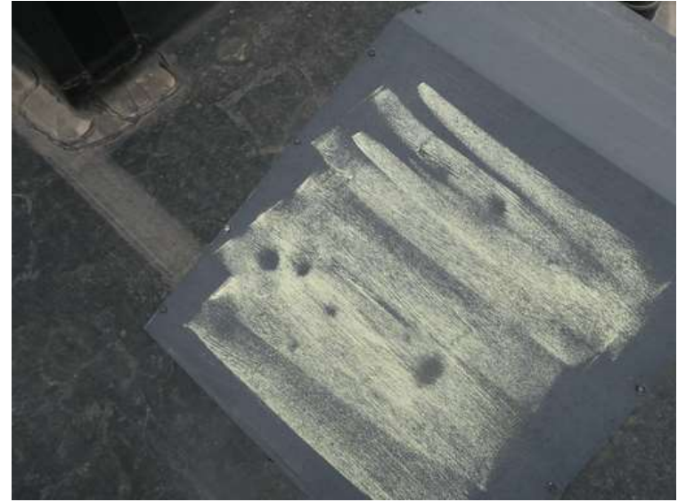
54. Building 02. Dents in an exhaust hood from hail.
