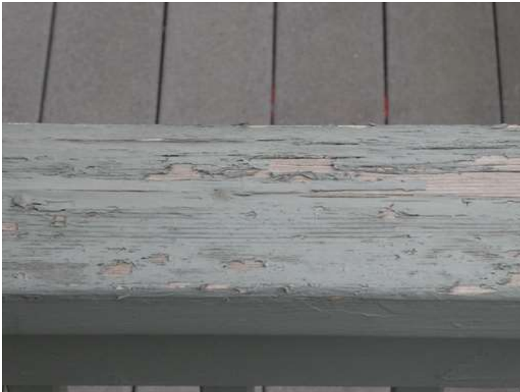
71. Building 03. Chips in worn paint on a hand railing from hail.
