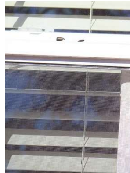
292. Building 13. Fractured glazing bead.
