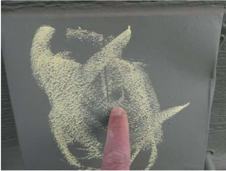
365. Building 16. Dent in a vent terminal from hail.
