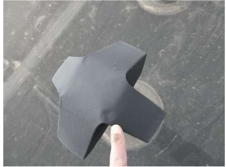
378. Building 16. Dent in a flue cap from hail.
