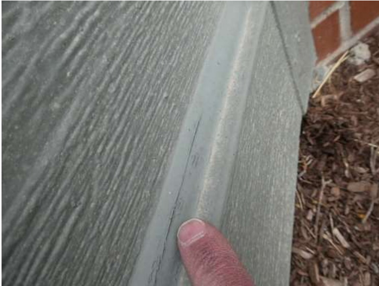
93. Building 04. Chips in paint from hail.
