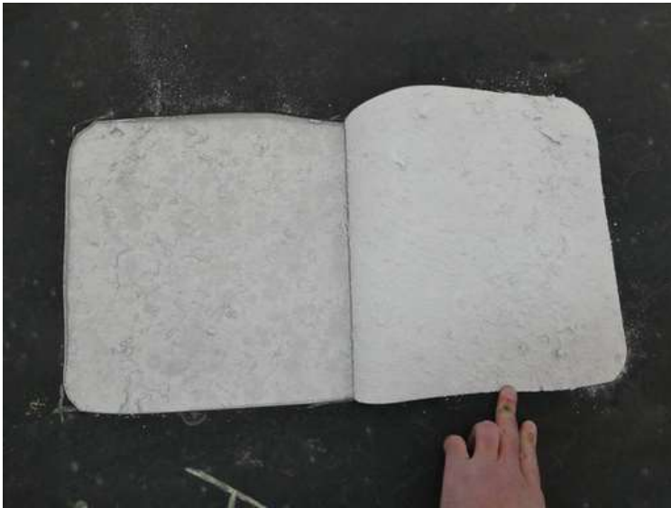
25. Building 01. Membrane folded back. The gypsum was powdery.
