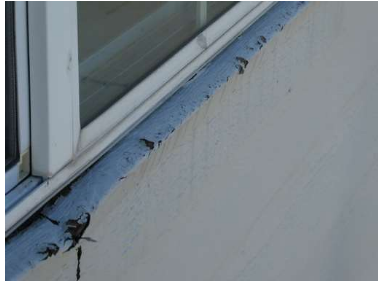
550. Building 23. Chips in paint on a fiberboard windowsill.
