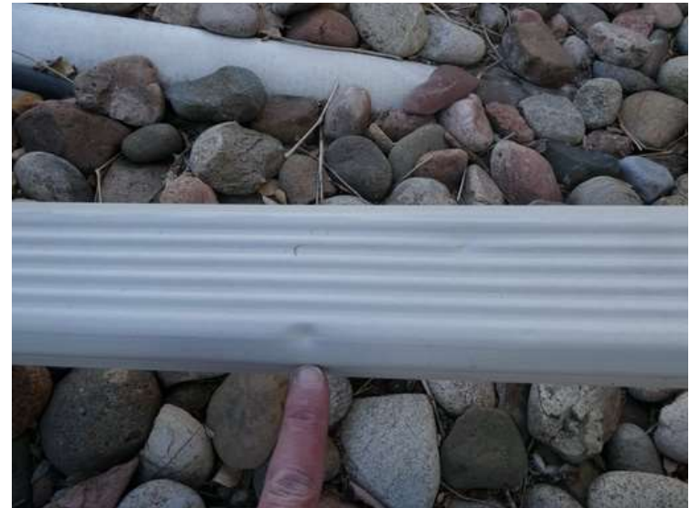
544. Building 23. Dent in a downspout extension from hail.
