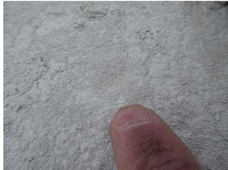
26. Building 01. Powdery gypsum.
