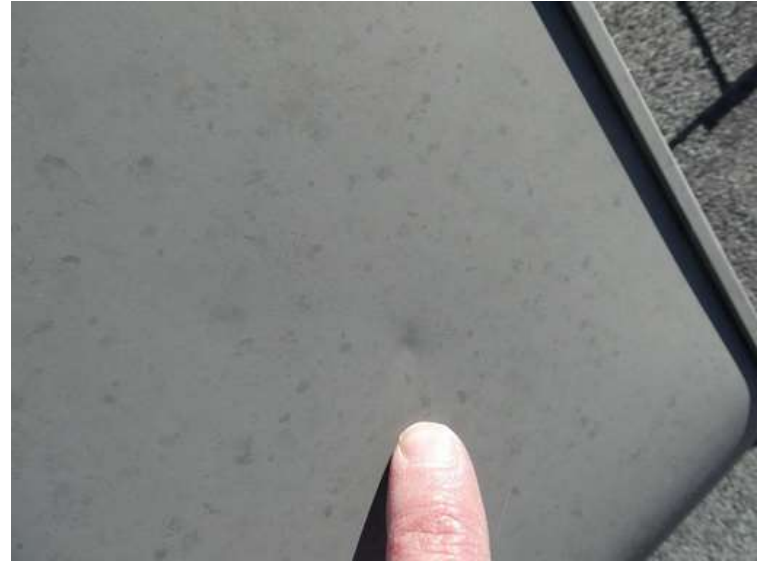
554. Building 23. Dent in a steel attic vent from hail.
