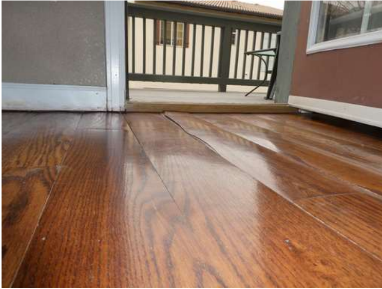
81. Building 03. Warped flooring in the dining area on the second floor.
