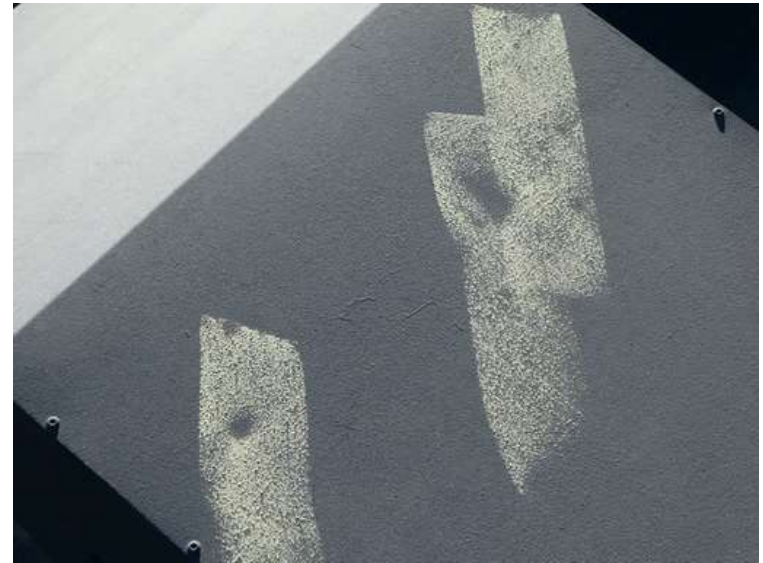
620. Building 25. Dents in an exhaust hood from hail.
