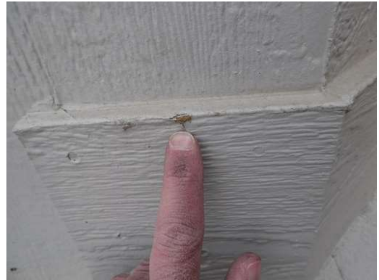
144. Building 06. Chip in paint from hail.
