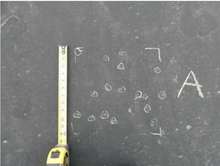
23. Building 01. Test area. Circular chalk marks denote dents in the substrate.
