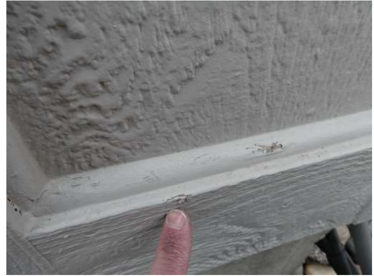
118. Building 05. Chips in paint from hail.
