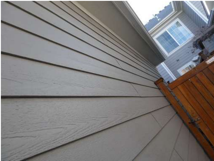
455. Building 20. Paint finishes on fiber cement siding were not fractured by hail.
