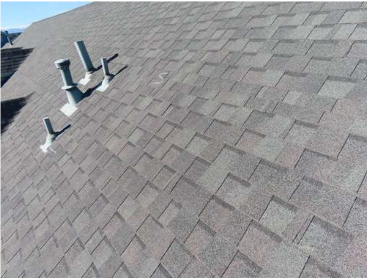
399. Building 17. South test area. No shingles within the test area were bruised by hail.
