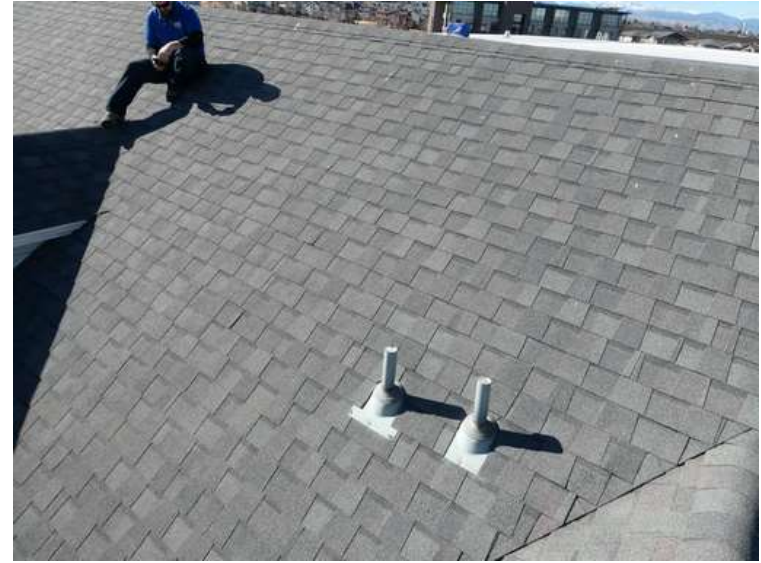
566. Building 23. East test area. No shingles within the test area were bruised by hail.
