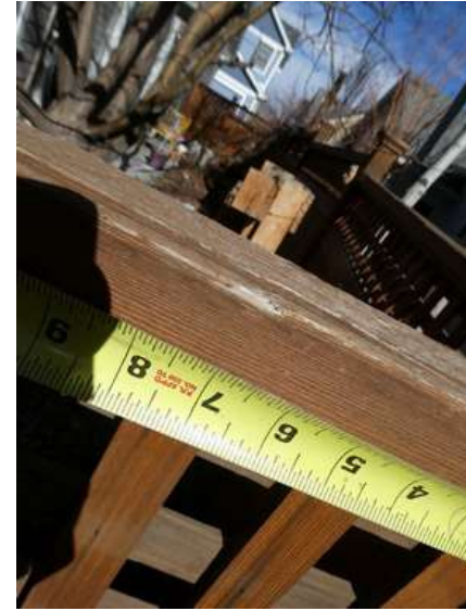
450. Building 20. Chip in a wood fence.
