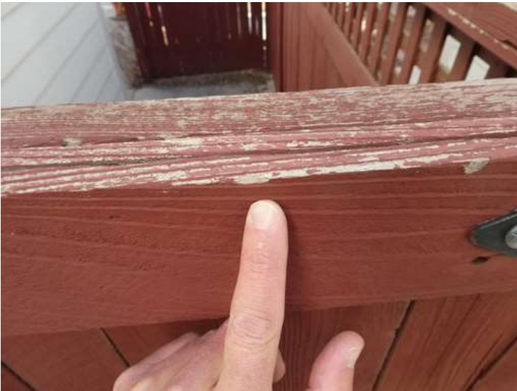
243. Building 10. Stain scuffed by hail.
