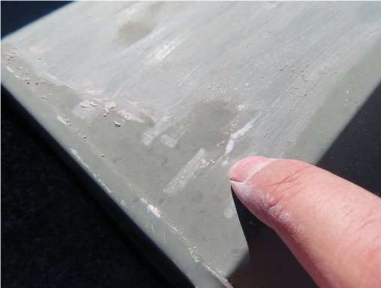
393. Building 17. Dent in an attic vent with a corresponding spatter mark.
