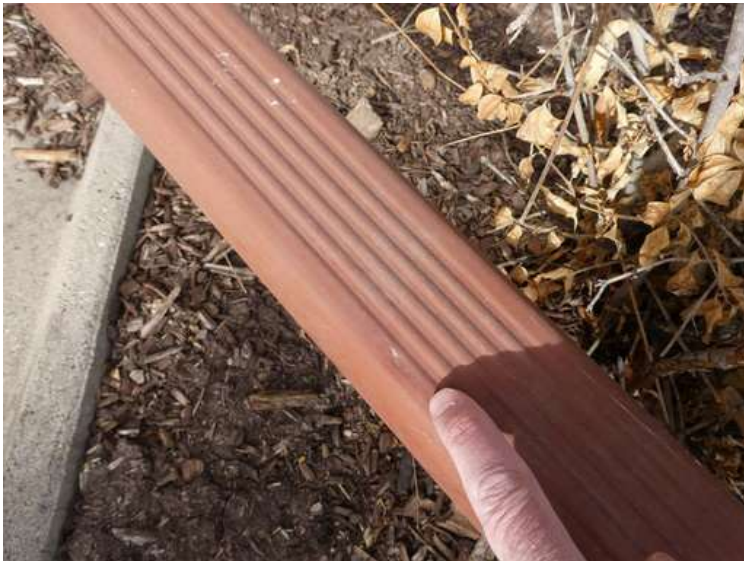
335. Building 15. Dent in a downspout extension from hail.
