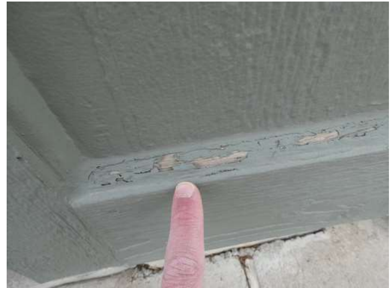
342. Building 15. Chips in weathered paint from hail.
