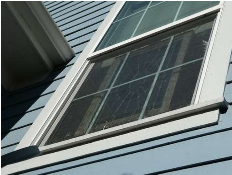
583. Building 24. Tears in a screen from hail.
