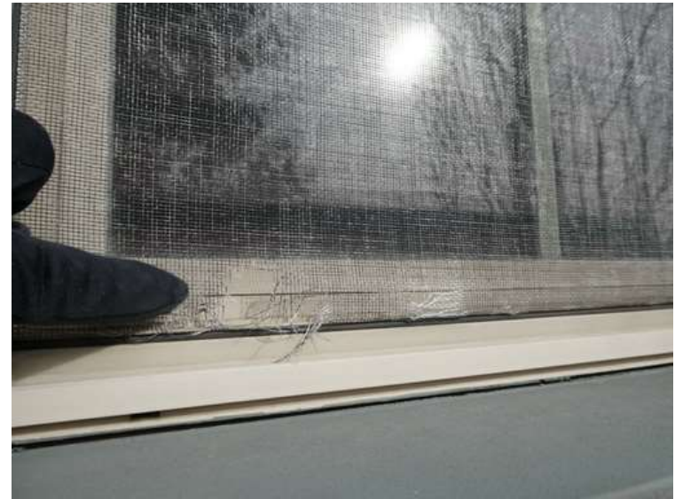
316. Building 14. Tears in a screen.
