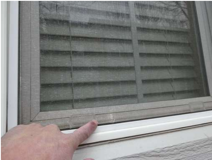
139. Building 06. Tears in a screen from hail.
