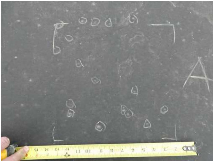
133. Building 05. Test area. Circular chalk marks denote dents in the substrate.
