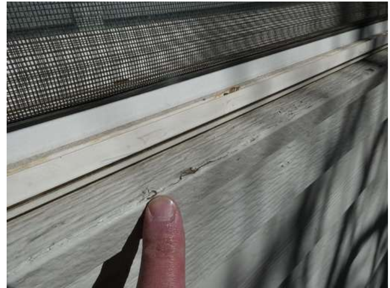
472. Building 21. Chips in paint on a sill from hail.
