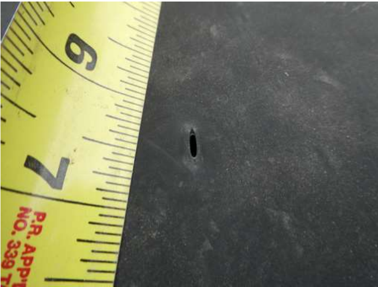
75. Building 03. Mechanical cut in the membrane.
