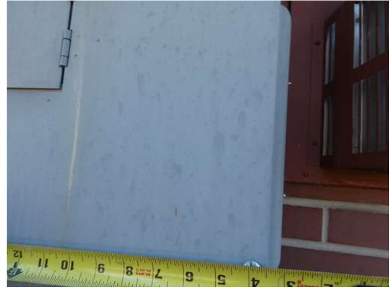
638. Building 26. Spatter marks on an electrical box.
