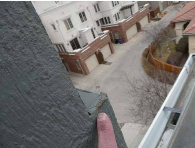
113. Building 04. Paint chipped by hail.
