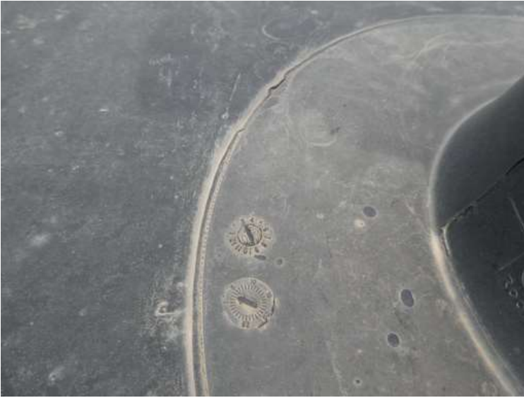
377. Building 16. Flashing boot dated, '05'.
