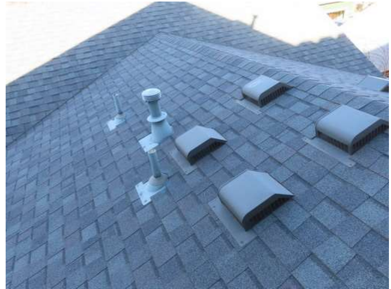
416. Building 18. West test area. No shingles within the test area were bruised by hail.
