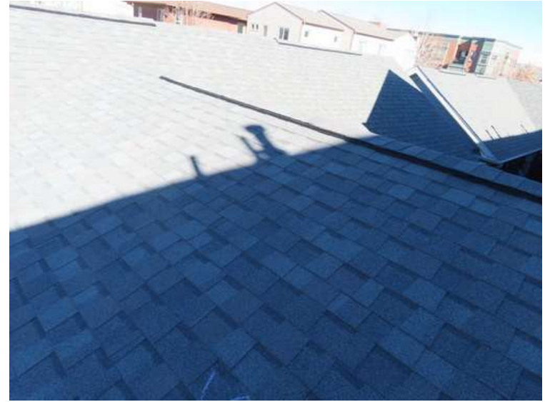
302. Building 13. West test area. No shingles within the test area were bruised by hail.
