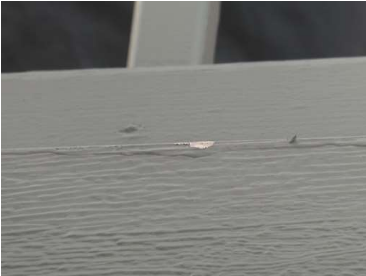
371. Building 16. Chip in paint on wood trim around a balcony from hail.
