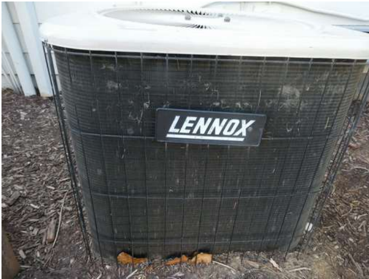
541. Building 23. Small dents in condenser fins from hail.
