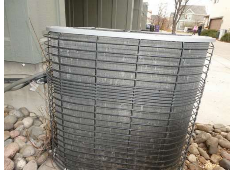
66. Building 03. Dents in condenser fins from hail.
