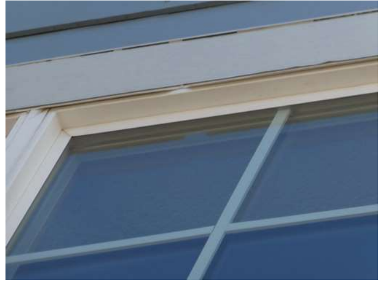
426. Building 19. Fractures in a vinyl window frame.
