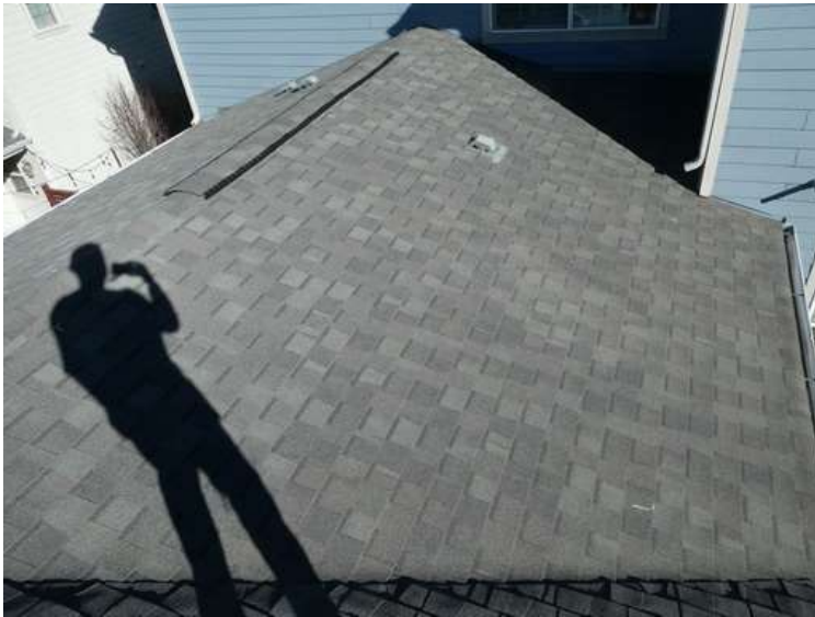
227. Building 09. South test area. No shingles within the test area were bruised by hail.
