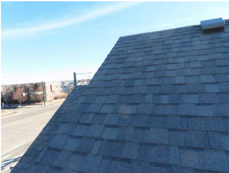
439. Building 19. North test area. No shingles within the test area were bruised by hail.
