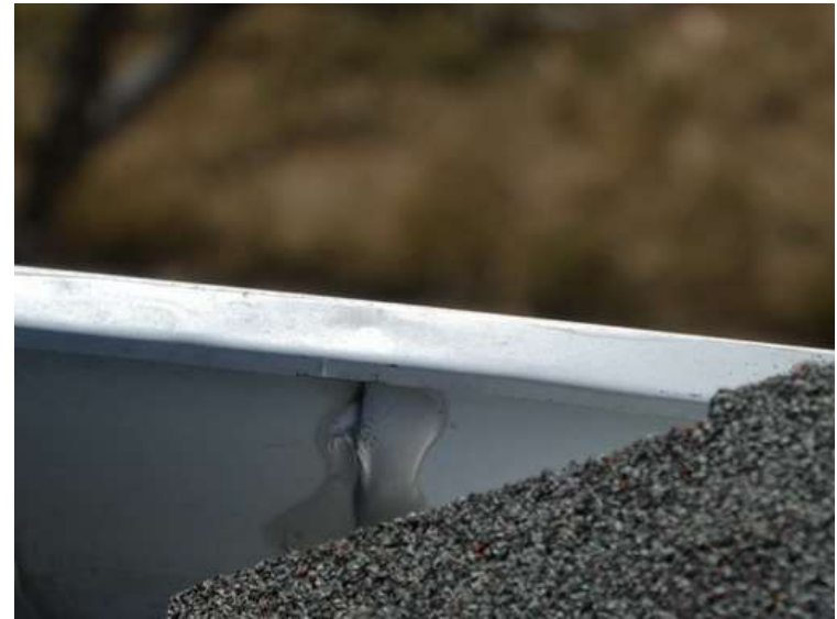
464. Building 20. Dent in a gutter.
