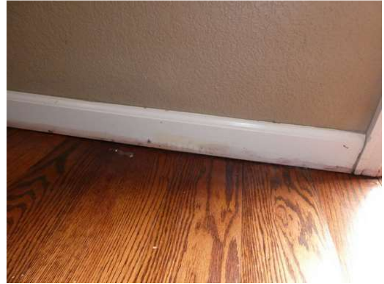
82. Building 03. Stained base board.
