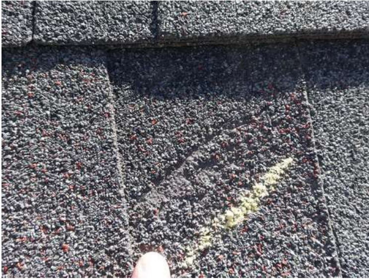
225. Building 09. Mechanical scuff.
