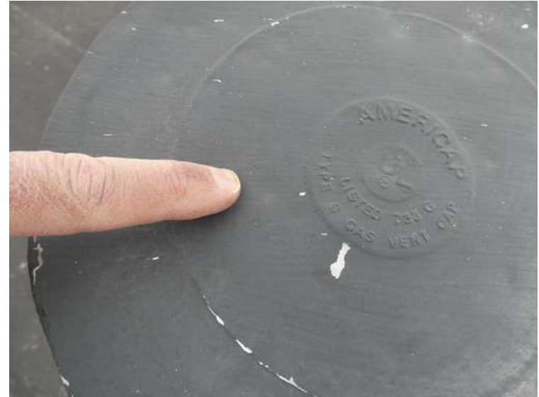
78. Building 03. Dents in a flue cap from hail.
