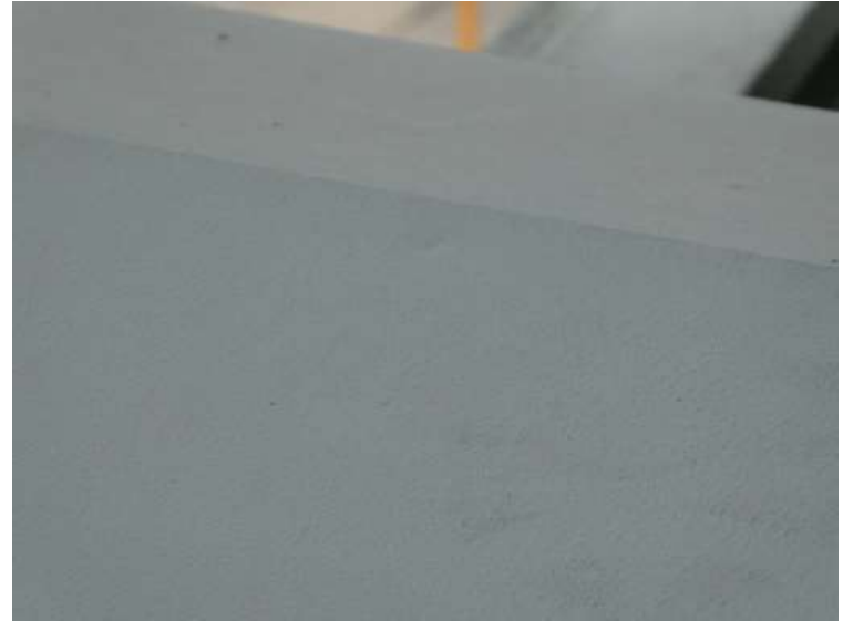
346. Building 15. Dents from hail.
