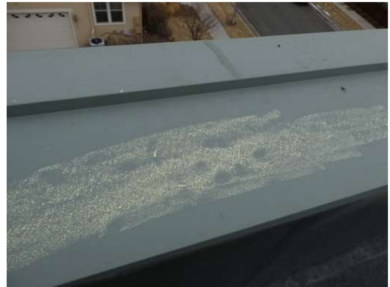
108. Building 04. Dents in coping from hail.
