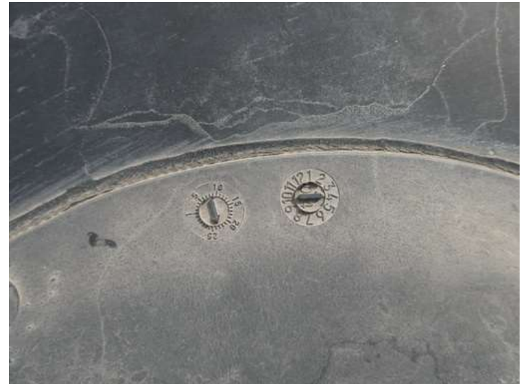
320. Building 14. Flashing boot dated, '04'.
