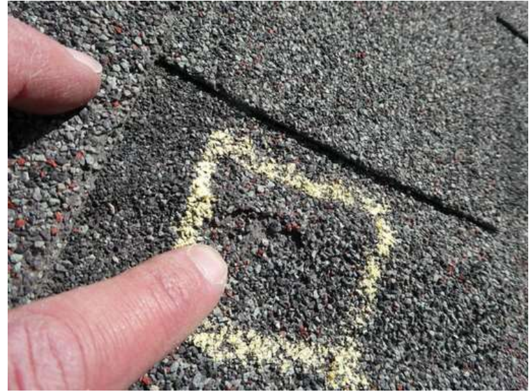
210. Building 08. Bruise in a wrinkle outside the test area.
