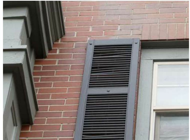
4. Building 01. Fractures in a plastic shutter.
