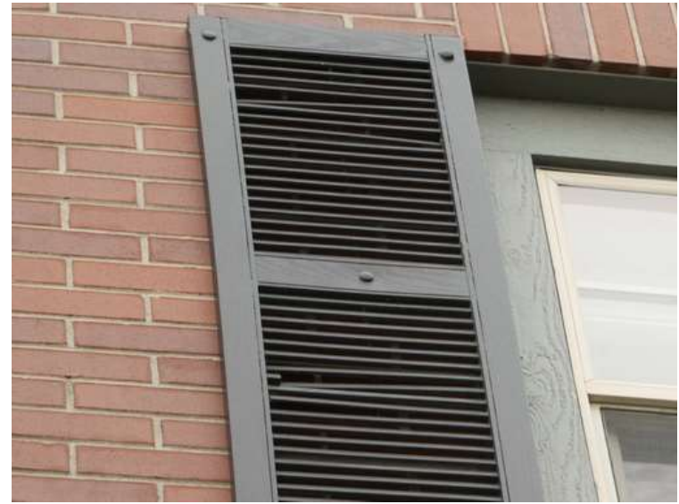
46. Building 02. Fractures in a shutter.
