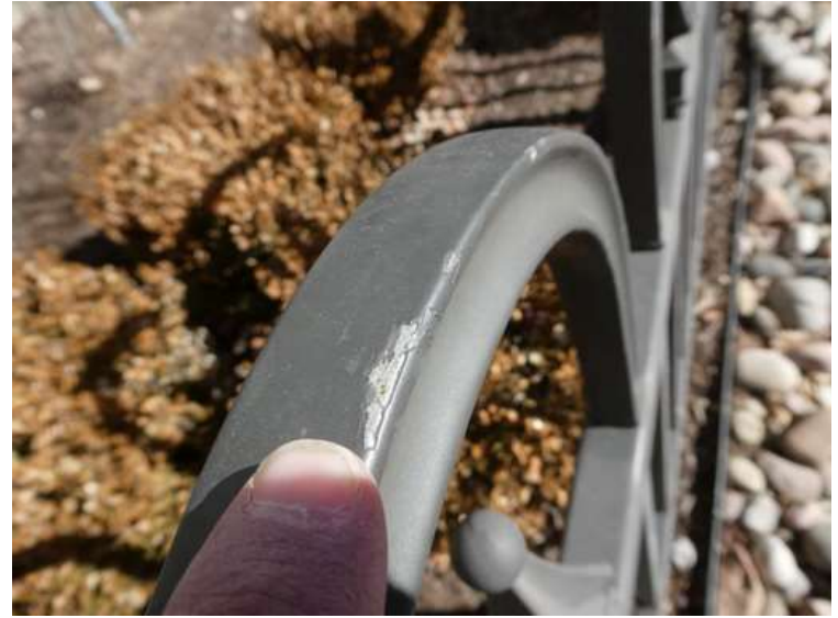
446. Building 20. Scrape in paint.
