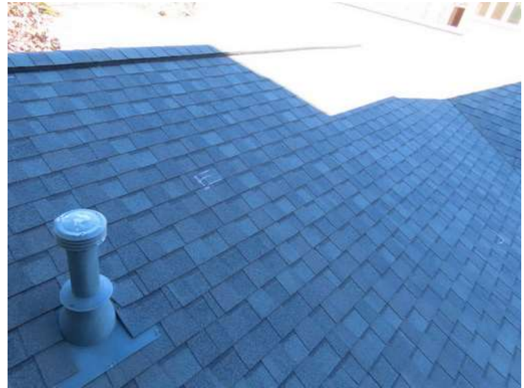
276. Building 11. East test area. No shingles within the test area were bruised by hail.
