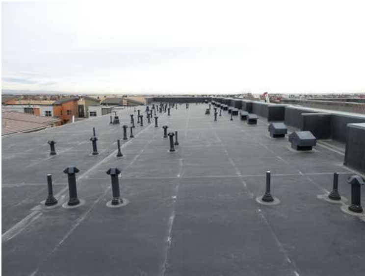
15. Building 01. View looking north. The roof was covered with an adhered EPDM membrane.
