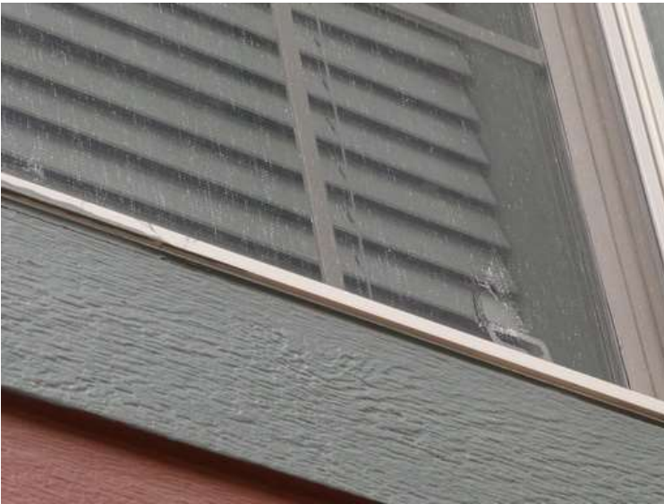
11. Building 01. Tears in a screen from hail.
