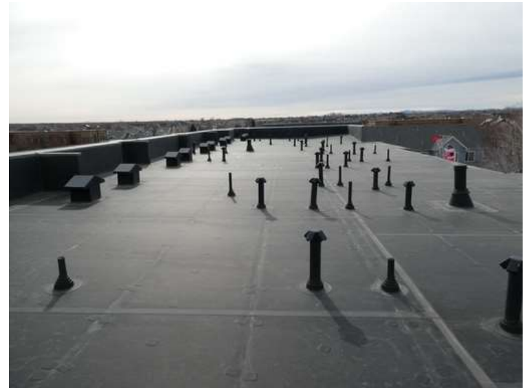
350. Building 15. View looking south. The roof was covered with an adhered EPDM membrane.
