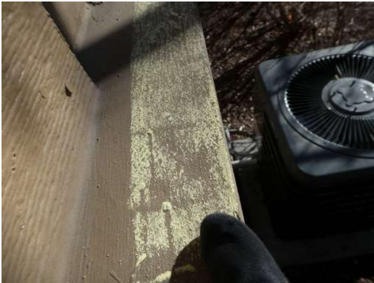
627. Building 26. Dent in steel flashing.
