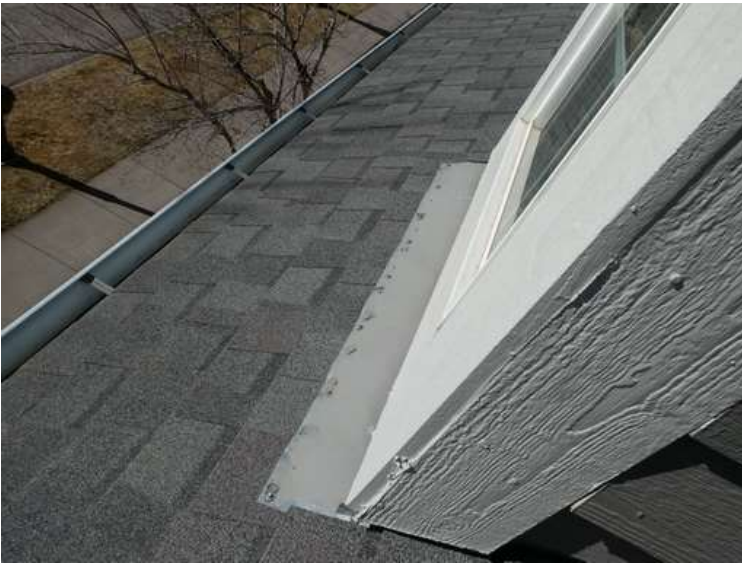
467. Building 20. Re-used headwall flashing.
