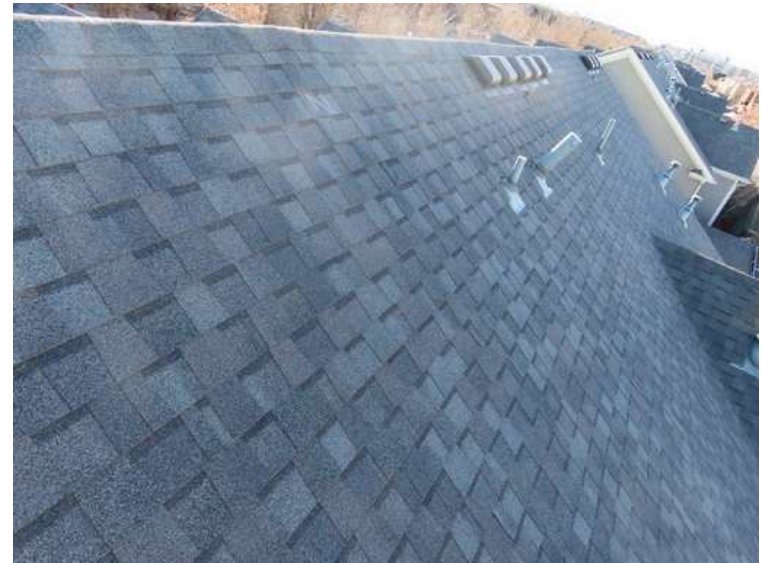
410. Building 18. North test area. No shingles within the test area were bruised by hail.
