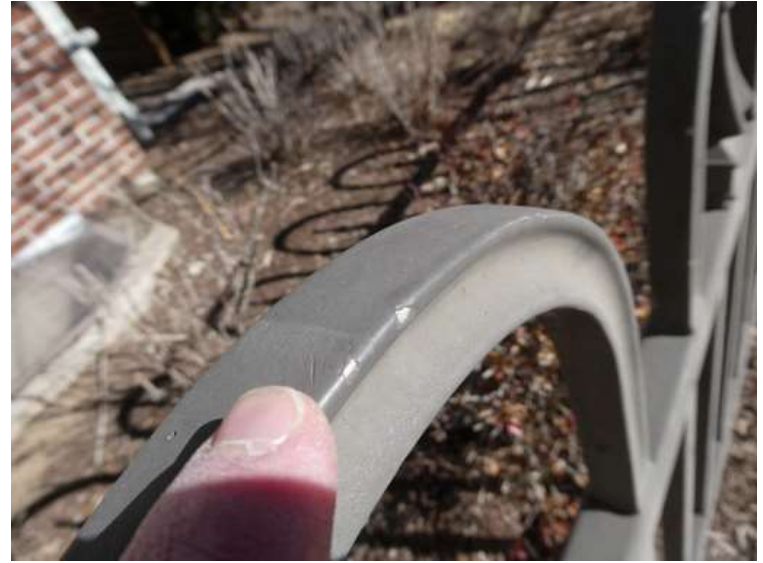
474. Building 21. Scuffs in paint.
