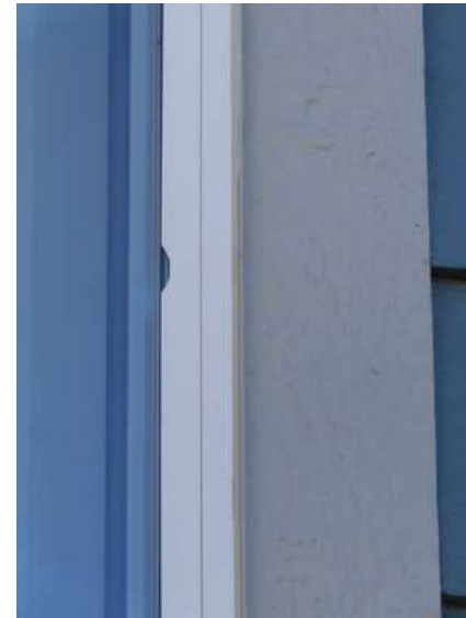
264. Building 11. Fracture in glazing bead from hail.
