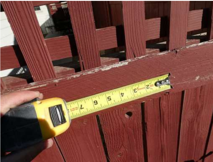
195. Building 08. Chips in a stained fence from hail.
