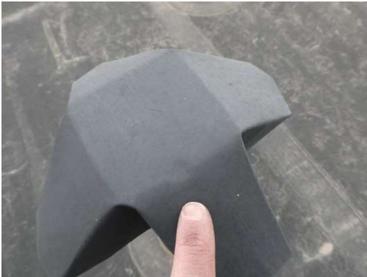
151. Building 06. Dent in a flue cap from hail.
