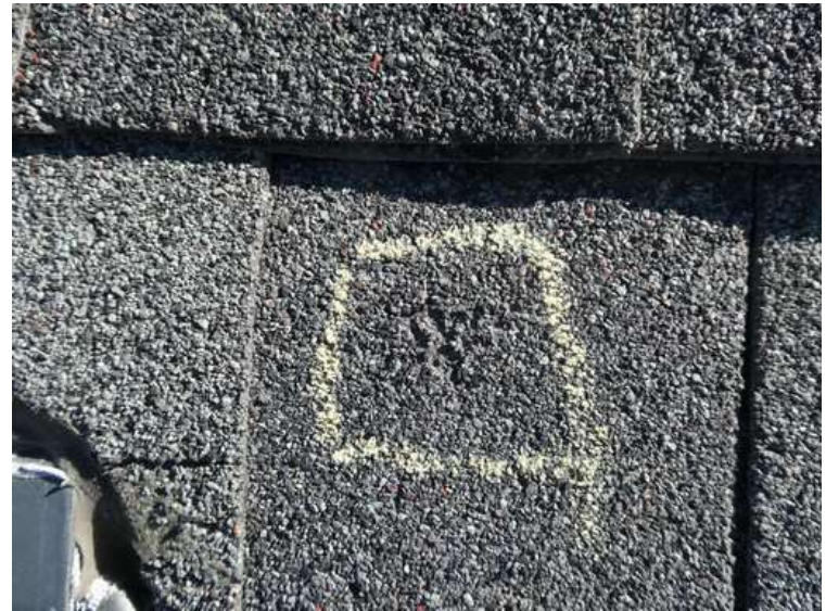
556. Building 23. Bruise in a shingle draped over flashing from hail.
