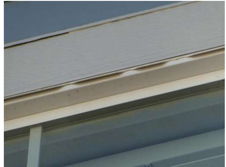
516. Building 22. Fractures in another window frame from hail.
