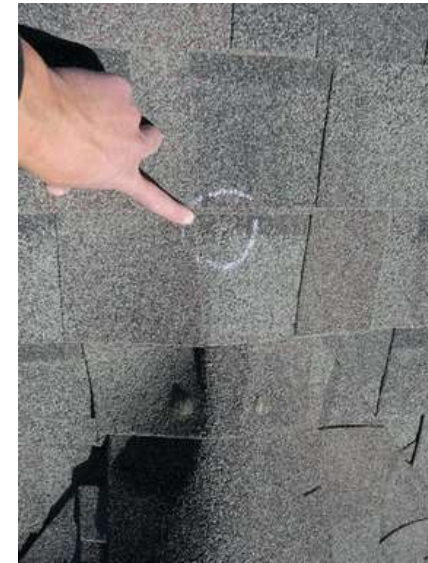
528. Building 22. Bruise in a ridge shingle.
