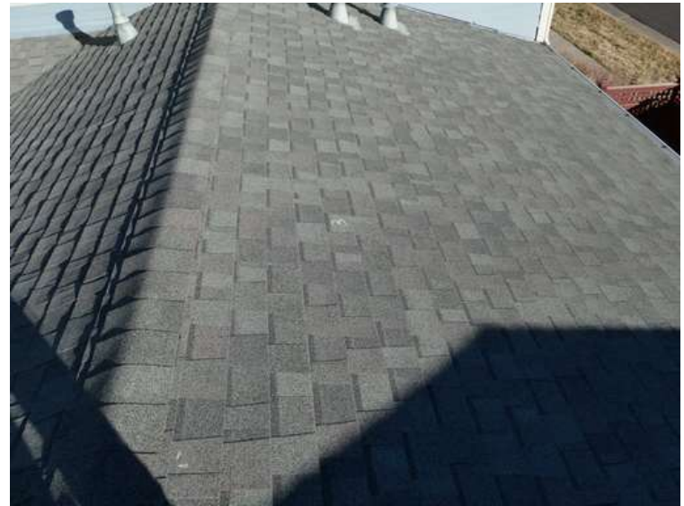
186. Building 07. South test area. No shingles within the test area were bruised by hail.
