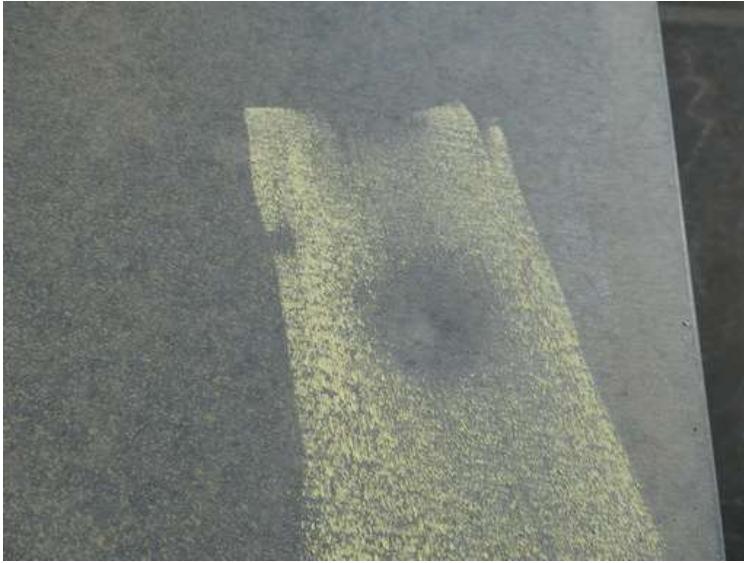
645. Building 26. Dent in coping from hail.
