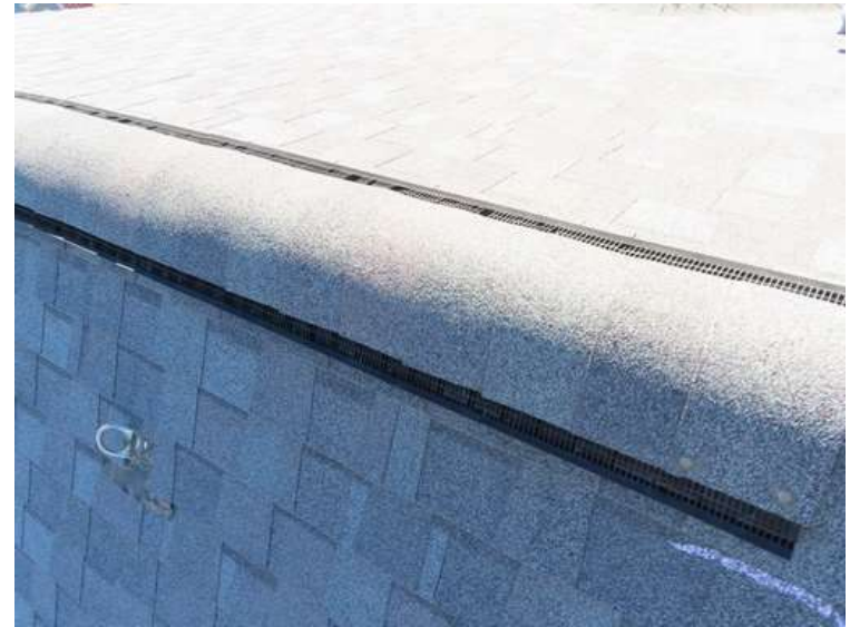
288. Building 12. Shingles draped over the ridge were not bruised by hail.
