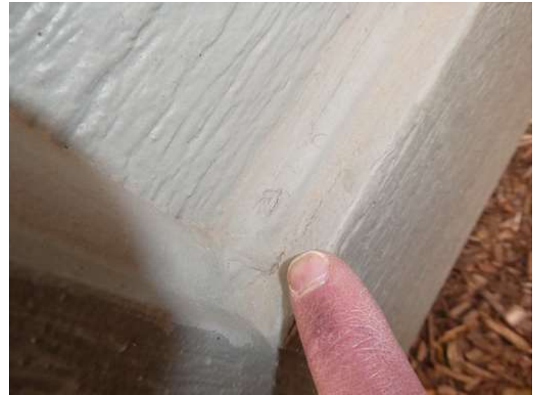
36. Building 02. Chips in paint from hail.
