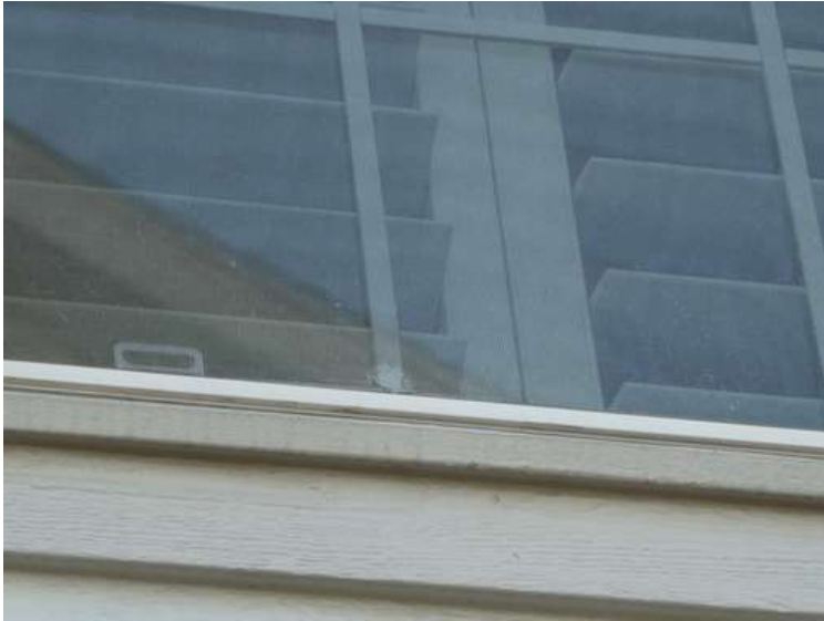
245. Building 10. Tear in a screen from hail.
