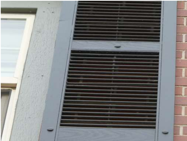
367. Building 16. Fracture in a shutter.
