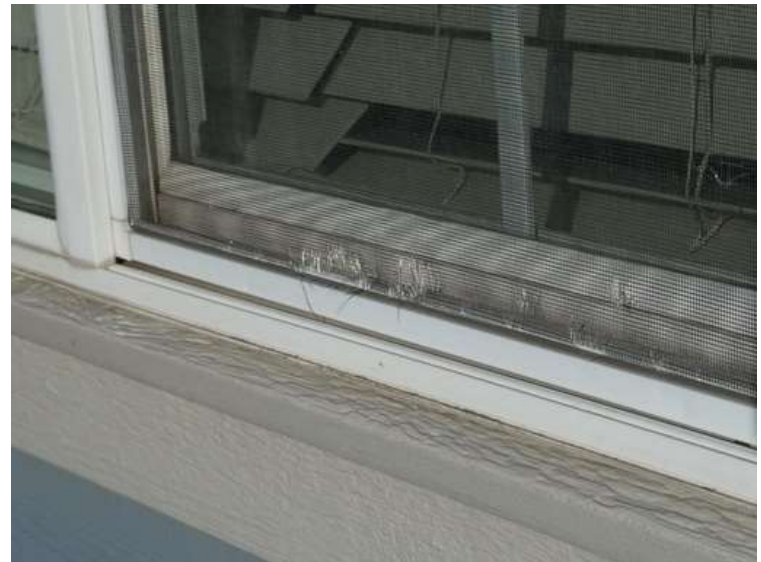
188. Building 07. Tears in a screen from hail.
