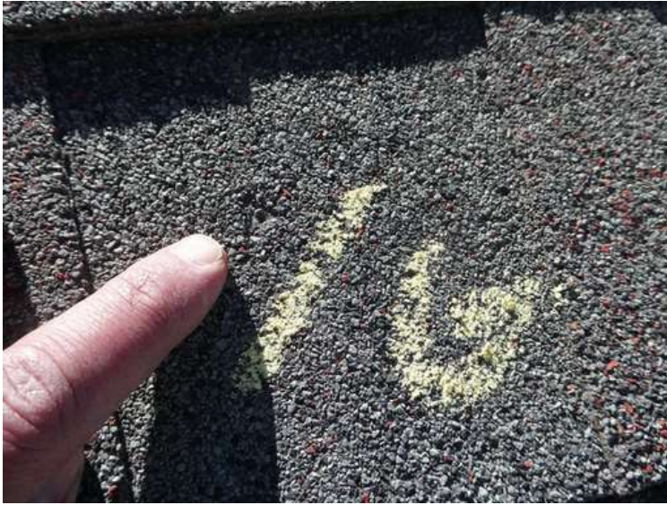
569. Building 23. Mechanical gouge.
