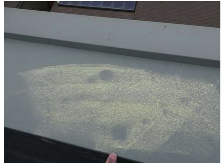
52. Building 02. Dents in coping.
