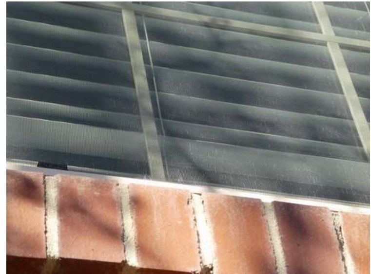
632. Building 26. Tears in a screen.
