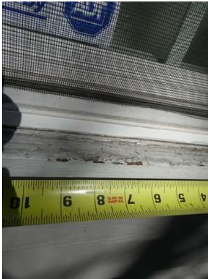
443. Building 20. Chips in paint on a fiberboard sill.
