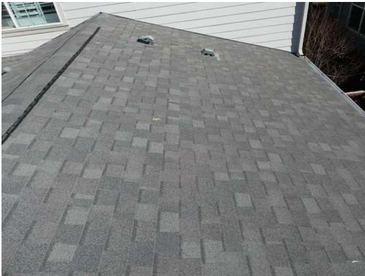
259. Building 10. South test area. No shingles within the test area were bruised by hail.
