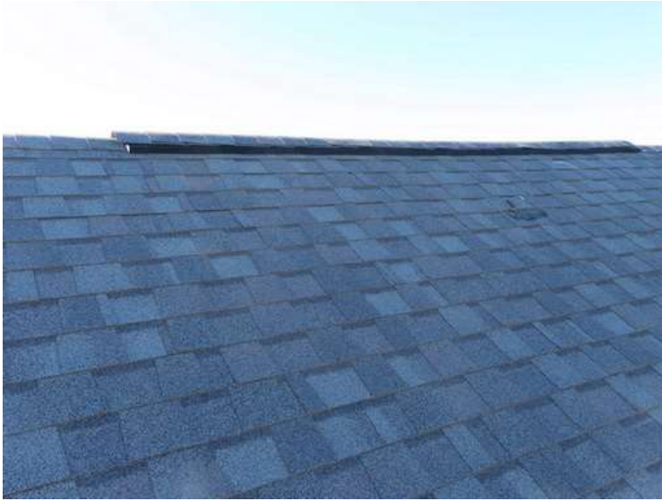
273. Building 11. North test area. No shingles within the test area were bruised by hail.
