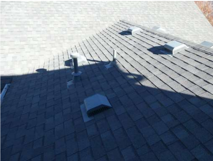
523. Building 22. West test area. No shingles within the test area were bruised by hail.
