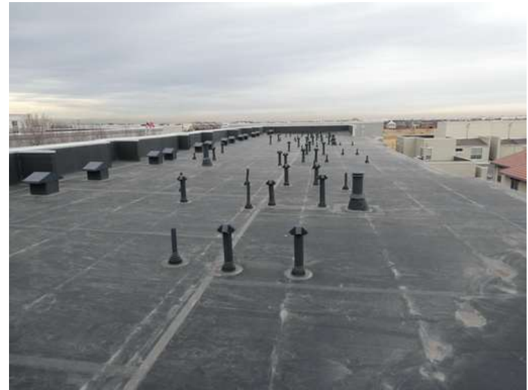
146. Building 06. View looking north. The roof was covered with an adhered EPDM membrane.
