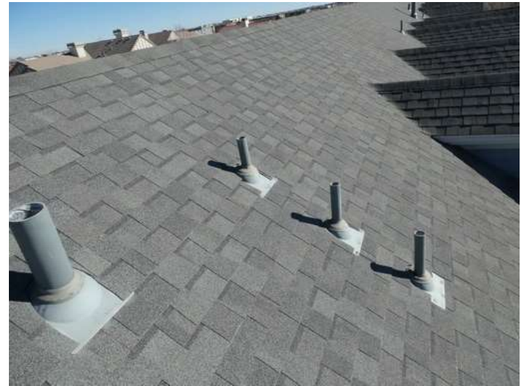
526. Building 22. South test area. No shingles within the test area were bruised by hail.
