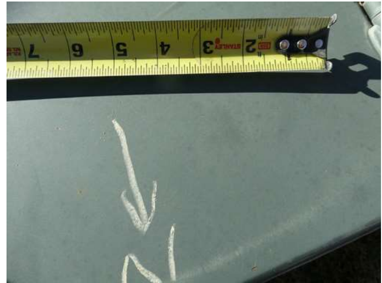
606. Building 25. Spatter marks on the top of a transformer cabinet.
