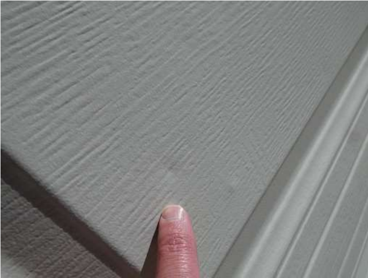
241. Building 10. Dent in a garage door from hail.
