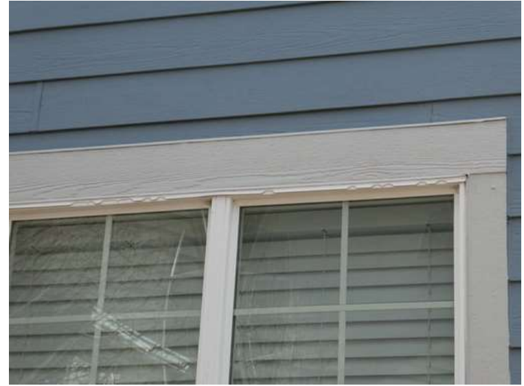
422. Building 19. Fractures in vinyl above the window.
