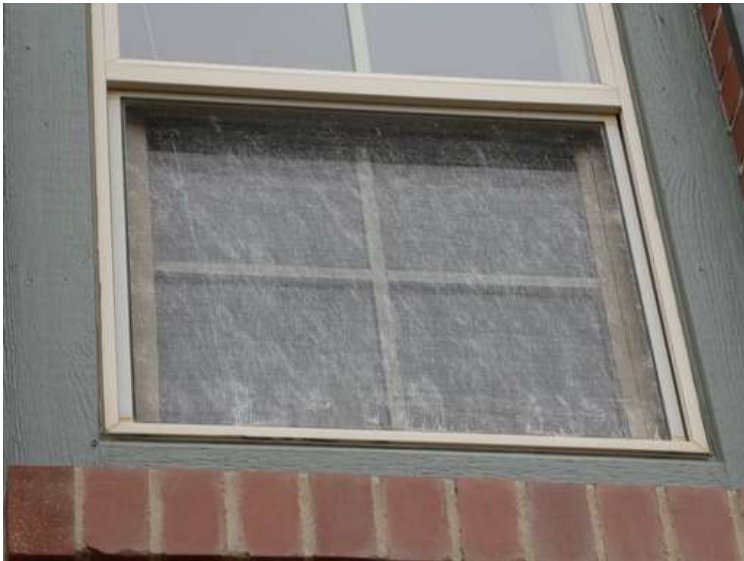
39. Building 02. Tears in a screen from hail.
