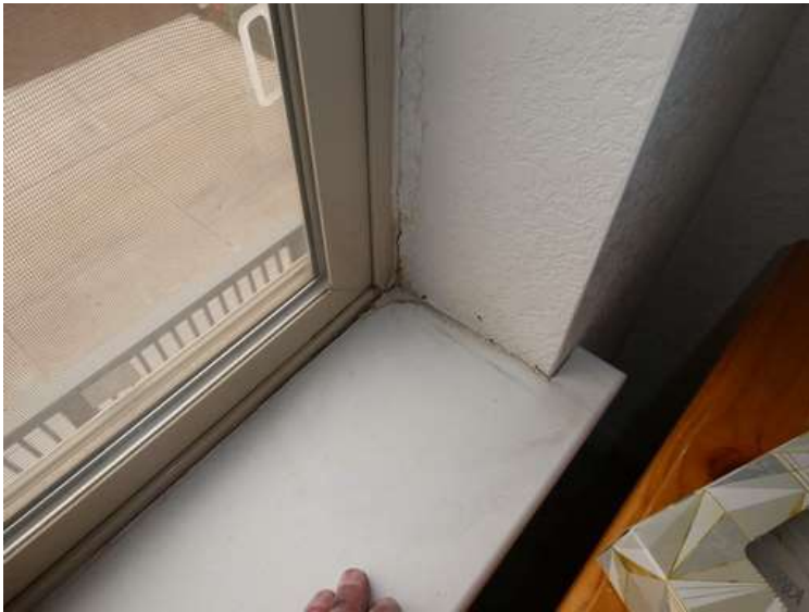
85. Building 03. Water stains.
