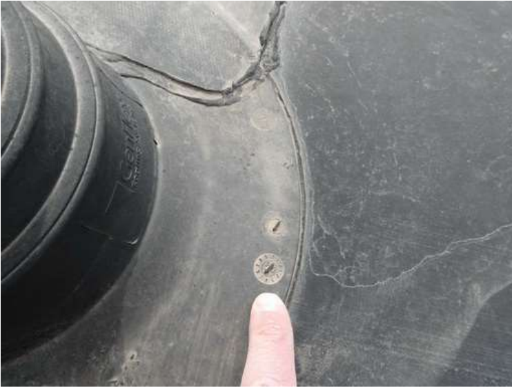
353. Building 15. Flashing boot dated, '04'.
