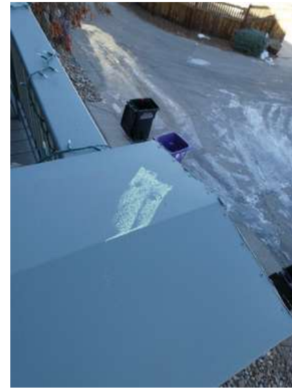
614. Building 25. Dents in a steel cap from hail.
