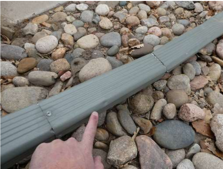
43. Building 02. Dent in a downspout extension from hail.
