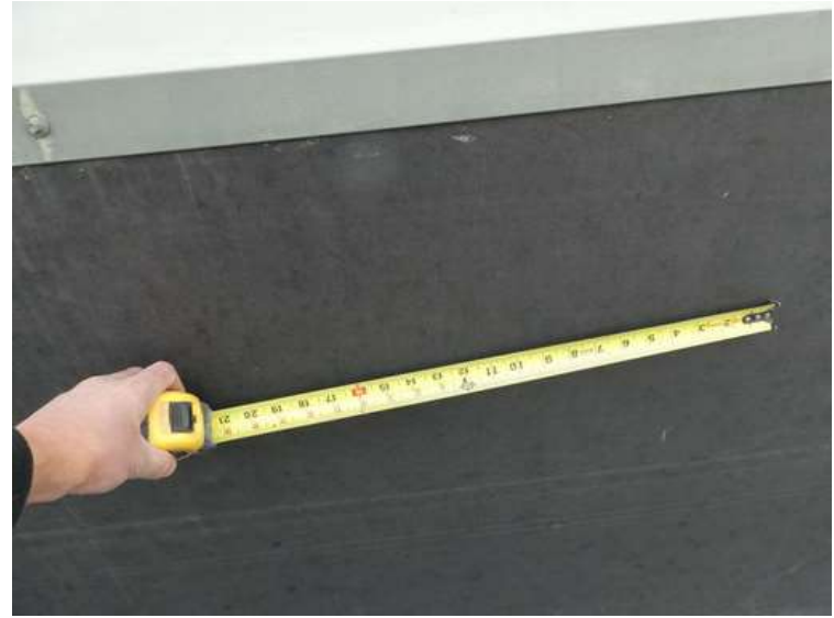
22. Building 01. Spatter marks on membrane extending up a parapet.
