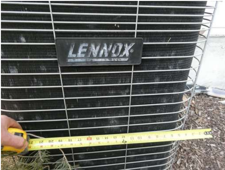
483. Building 21. Dents in condenser fins from hail.
