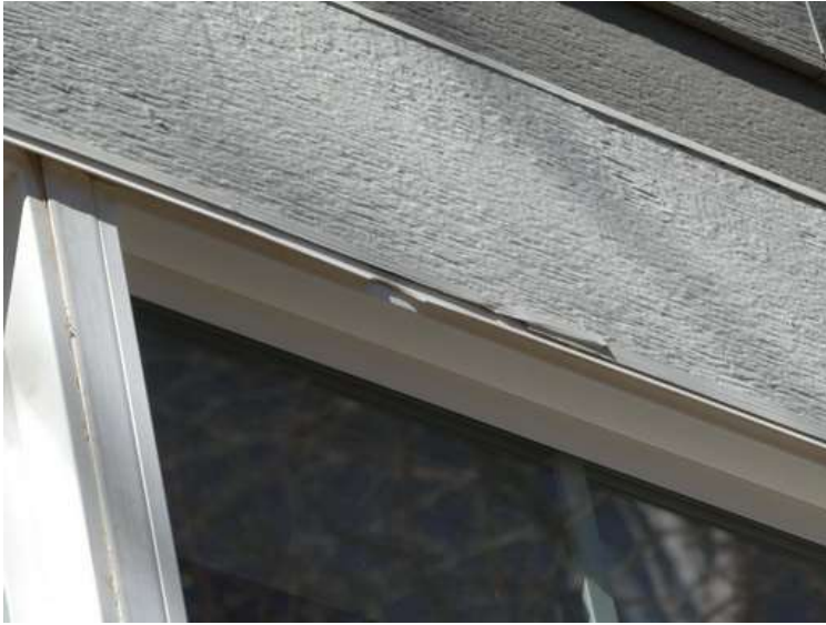
449. Building 20. Fracture in a vinyl window frame.
