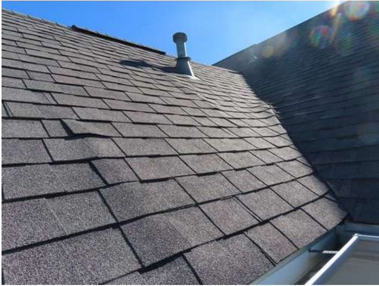
285. Building 12. Wrinkled roofing from decking movement.
