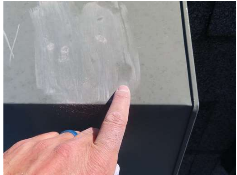
428. Building 19. Dents from hail.
