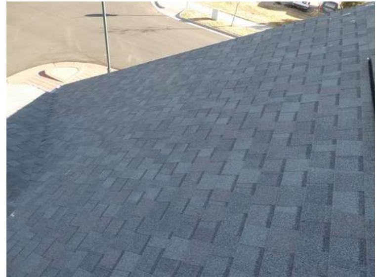
180. Building 07. East test area. No shingles within the test area were bruised by hail.
