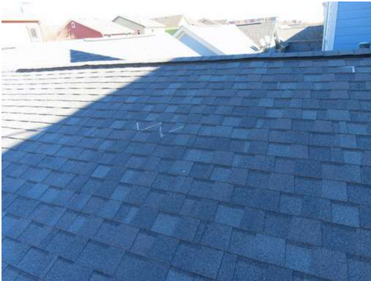
275. Building 11. West test area. No shingles within the test area were bruised by hail.
