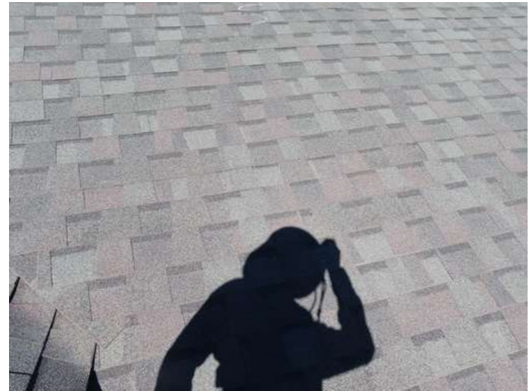
298. Building 13. South test area. No shingles within the test area were bruised by hail.
