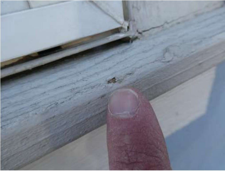
213. Building 09. Chip in paint on a sill.
