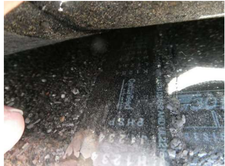
536. Building 22. Cellophane strip indicating impact resistant shingle.
