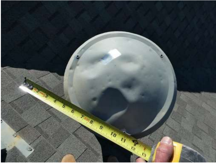
205. Building 08. Dents in a flue cap.
