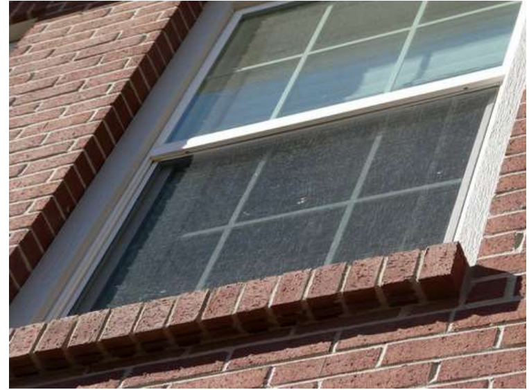
538. Building 23. Tears in a screen.
