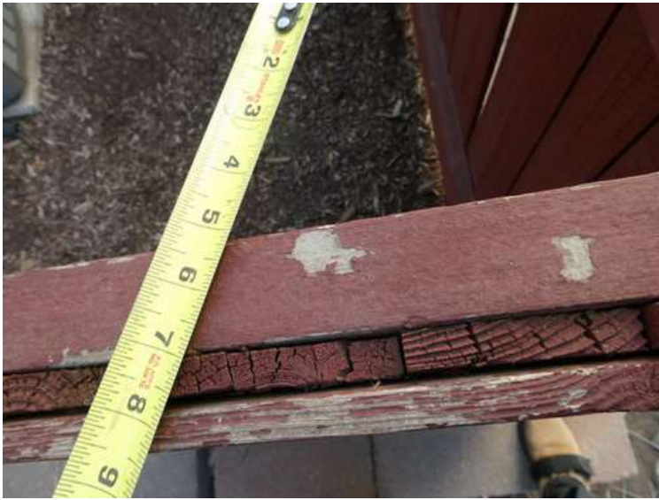
169. Building 07. Chip in stain on a wood fence.
