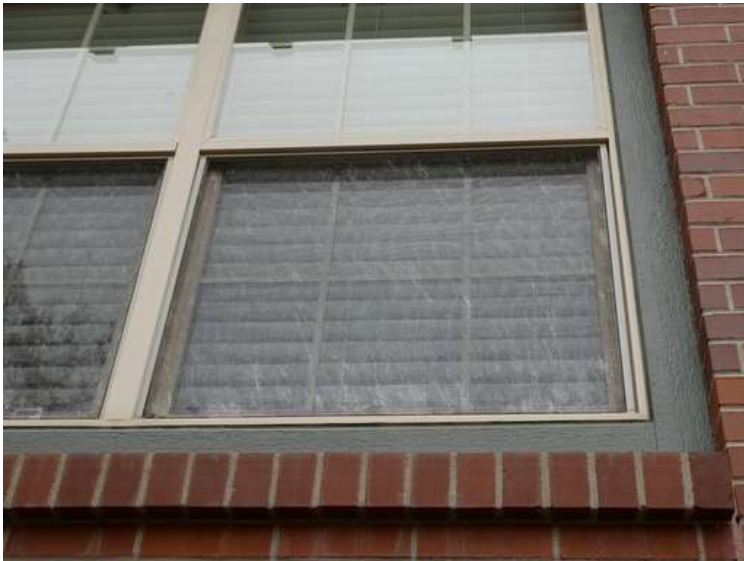
103. Building 04. Tear in a screen from hail.
