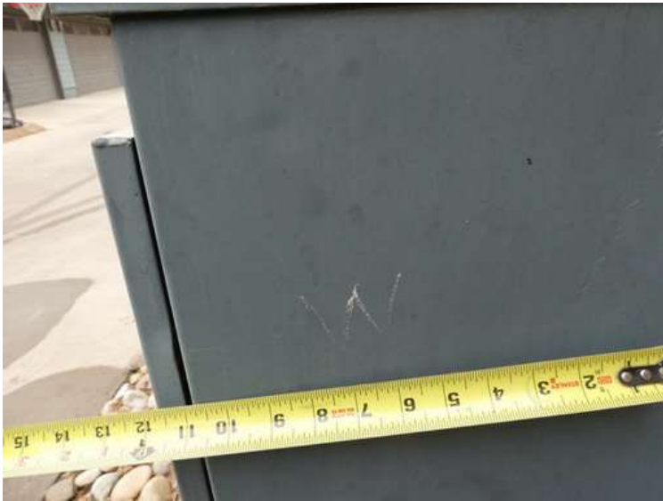
49. Building 02. Spatter marks on the west side of the cabinet.
