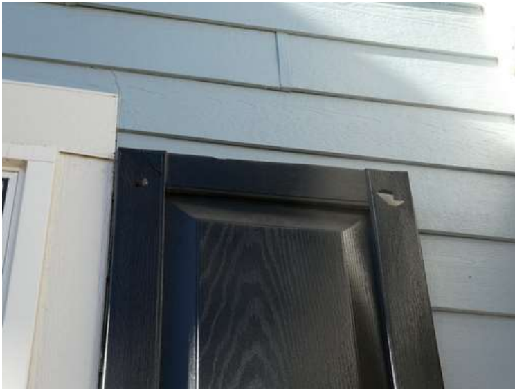
571. Building 24. Fractures in a shutter from wind.
