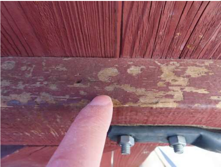
295. Building 13. Scuffs in stain on a wood fence.
