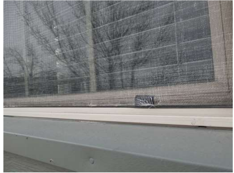
338. Building 15. Tears in a screen.
