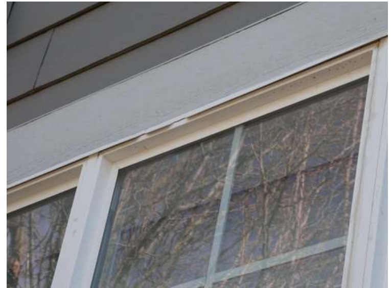
452. Building 20. Fractures in a vinyl window frame.
