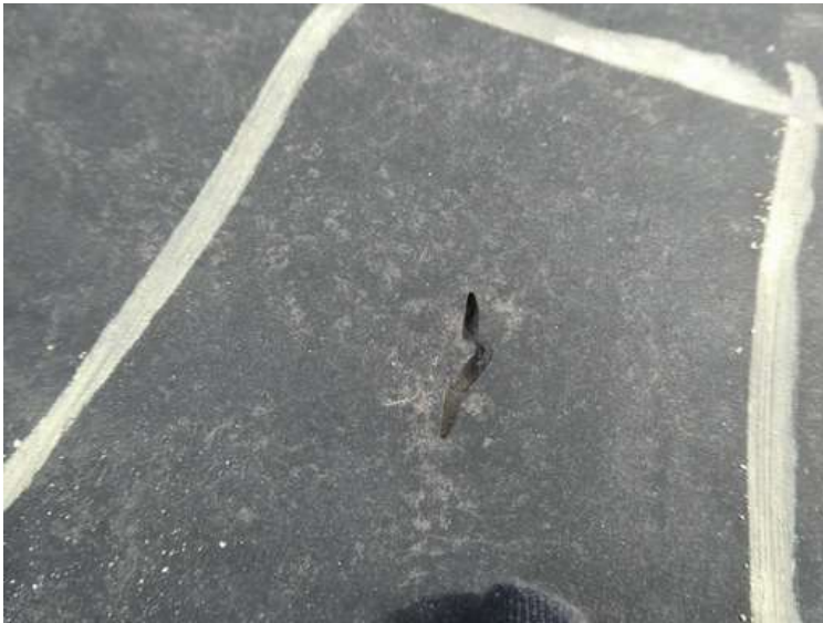
321. Building 14. Mechanical tear in the membrane.
