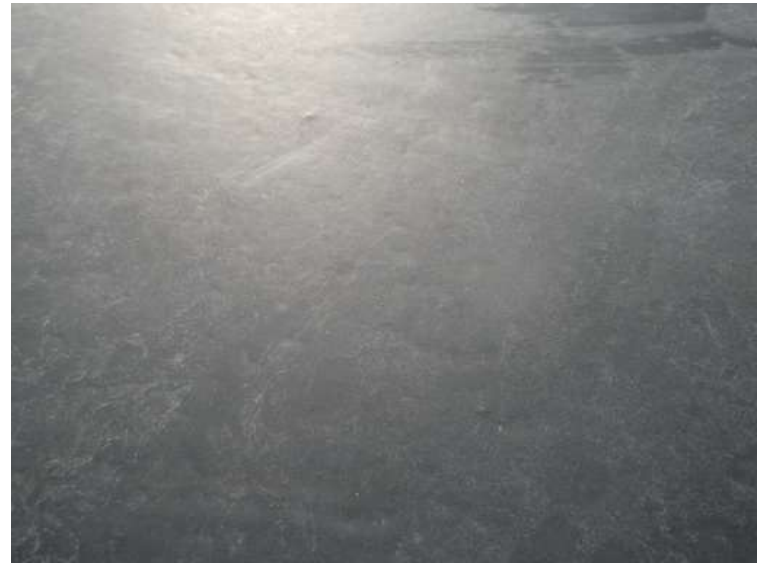
648. Building 26. Dents in the roof surface.
