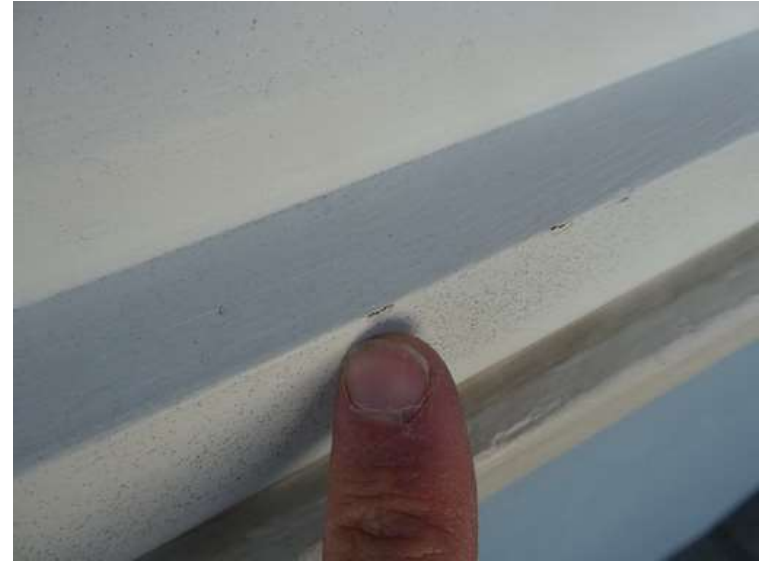
230. Building 09. Chips in paint on a north elevation sill.
