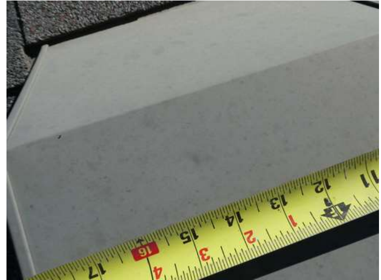
490. Building 21. Dent in an attic vent from hail.
