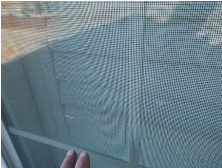
551. Building 23. Tears in a screen.
