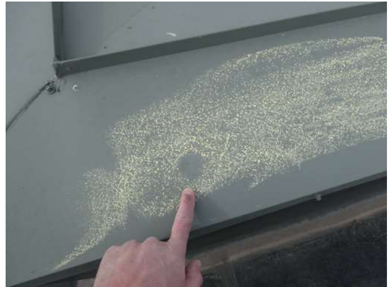
380. Building 16. Dent in coping from hail.
