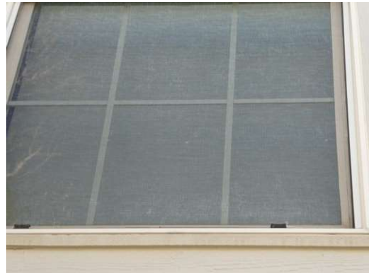
480. Building 21. Tears in a screen.
