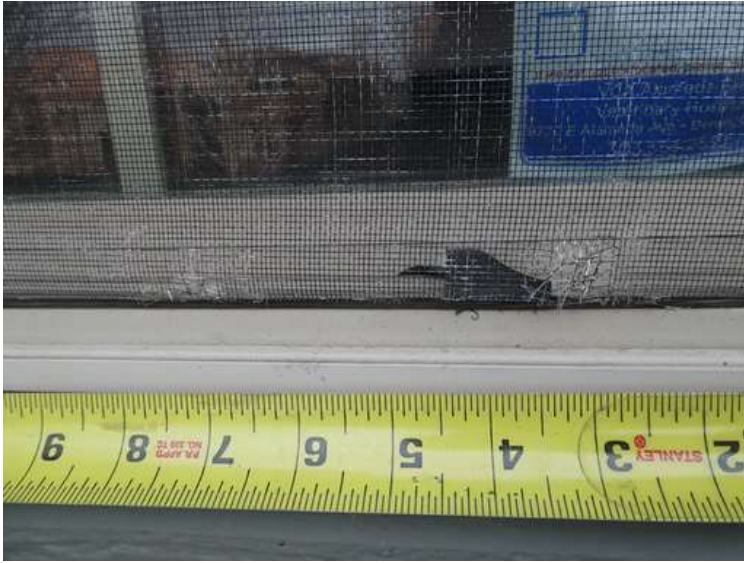
305. Building 14. Tears in a window screen from hail.
