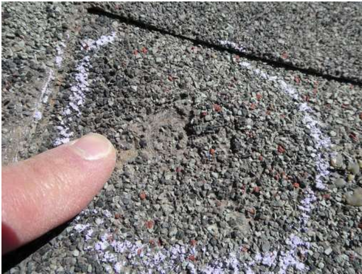
535. Building 22. Bruise in a ridge shingle.
