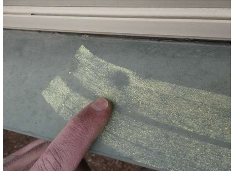
94. Building 04. Dent in steel flashing a ledge.
