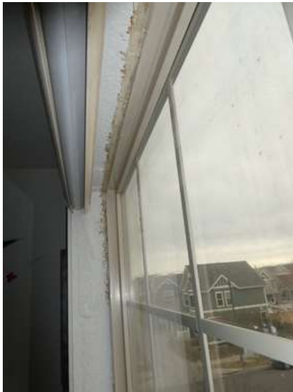
83. Building 03. Water leaked from above this window on the third floor.
