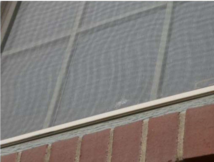
47. Building 02. Tears in a screen.
