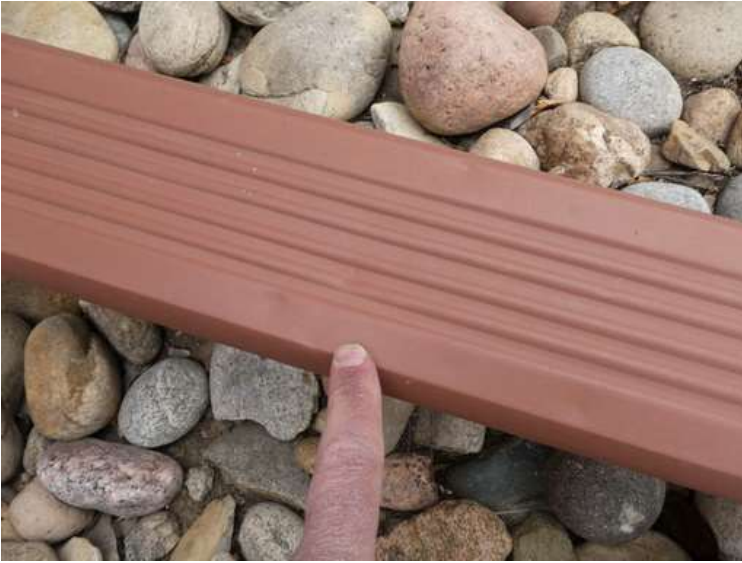
121. Building 05. Dents in a downspout extension from hail.
