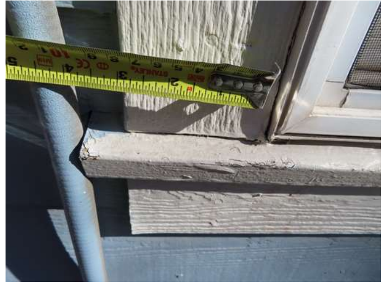
294. Building 13. Paint on a windowsill chipped by hail.
