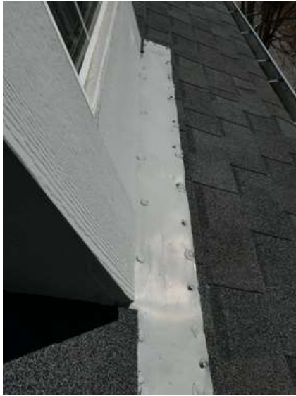
533. Building 22. Re-used flashing.
