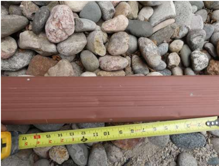
69. Building 03. Dents in a downspout extension from hail.
