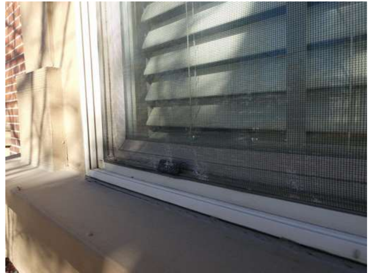
628. Building 26. Tears in a screen.
