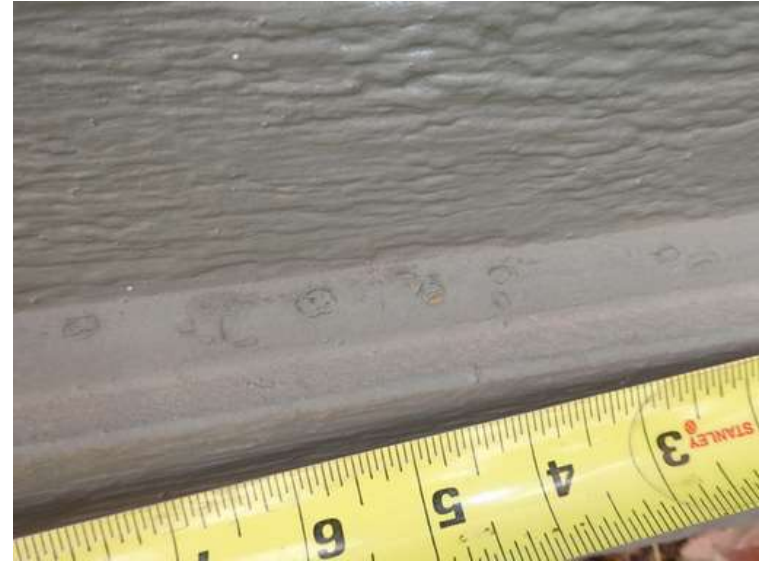
306. Building 14. Chips in paint from hail.
