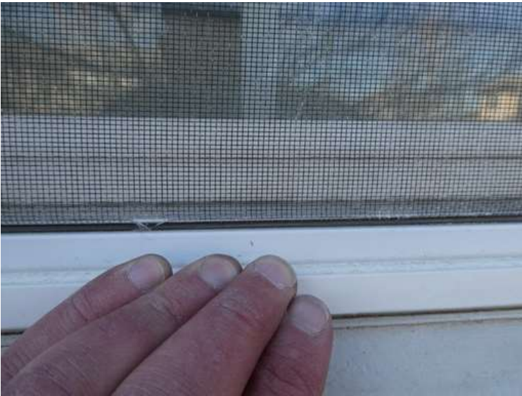
191. Building 08. Tears in a screen.
