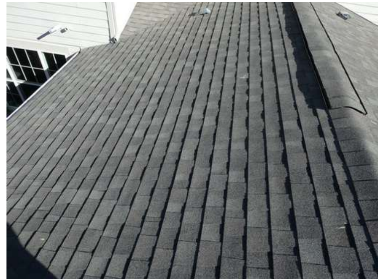
260. Building 10. North test area. No shingles within the test area were bruised by hail.
