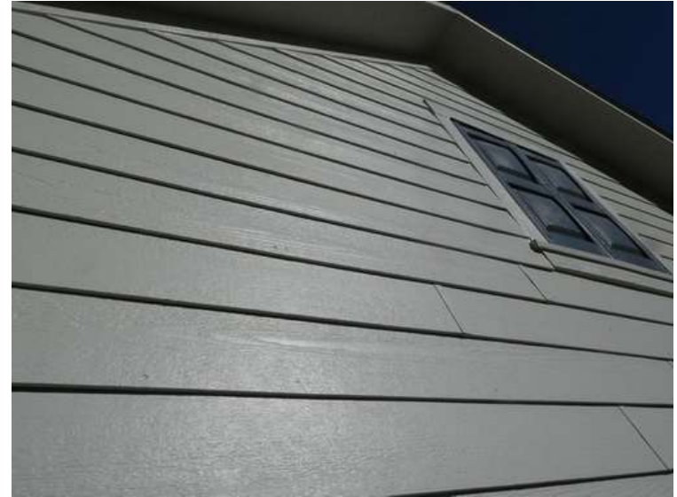
546. Building 23. Paint finishes on fiber cement siding were not chipped by hail.
