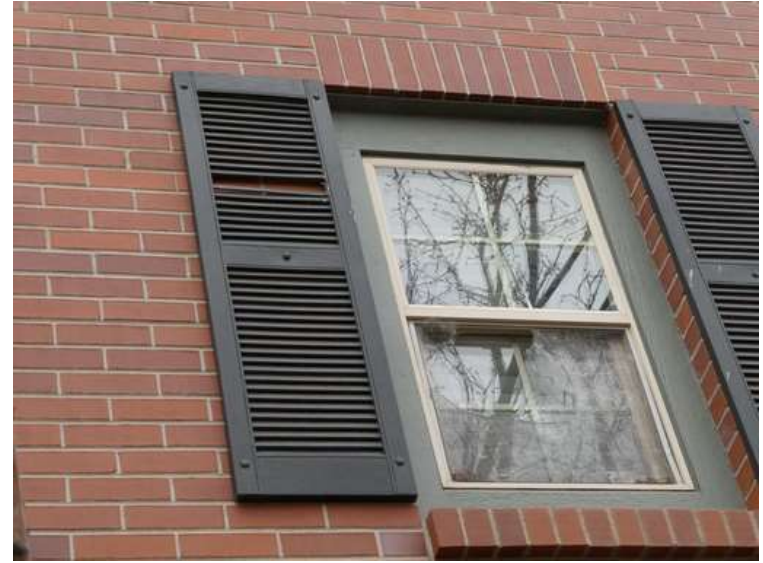
102. Building 04. Shutter fractured by hail.
