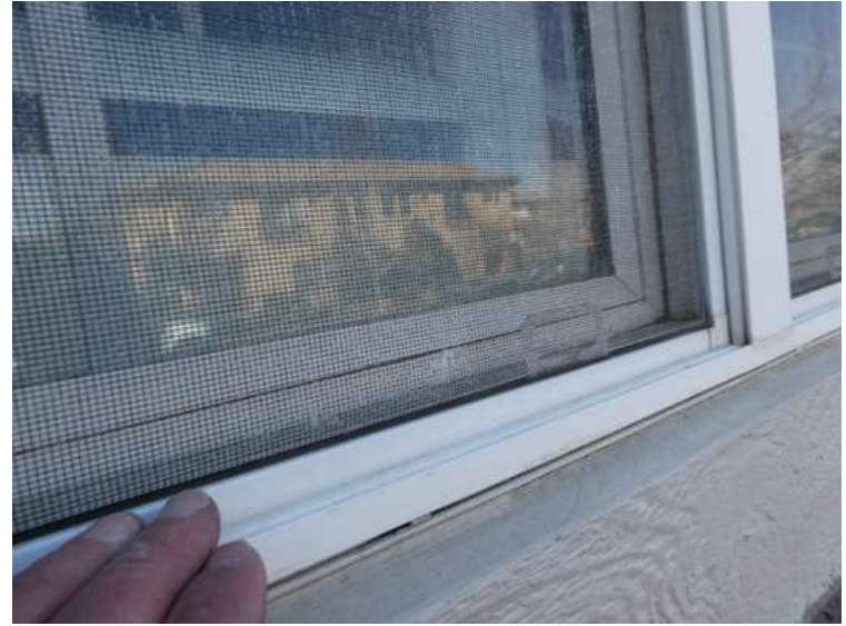
214. Building 09. Tears in a screen.
