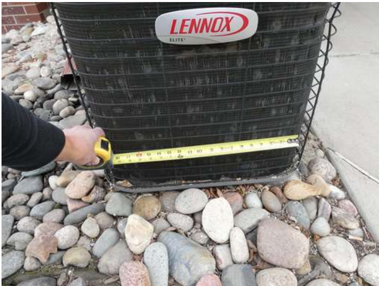
7. Building 01. Dents in condenser fins from hail.
