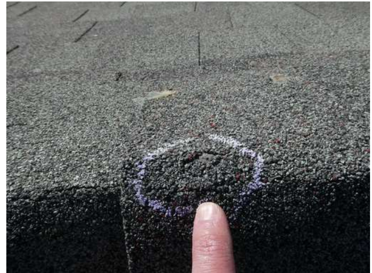
524. Building 22. Bruise in a ridge shingle.
