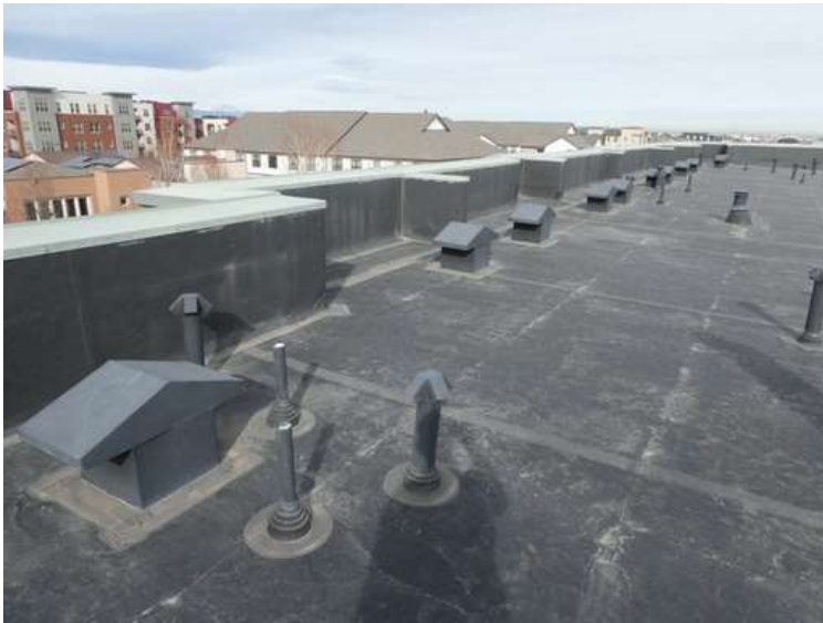
325. Building 14. Vent hoods.
