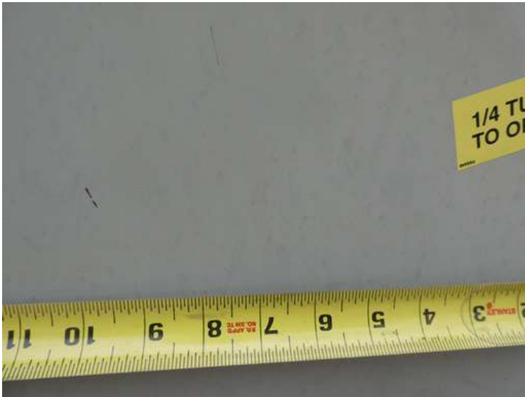
97. Building 04. Spatter marks on an electrical cabinet.
