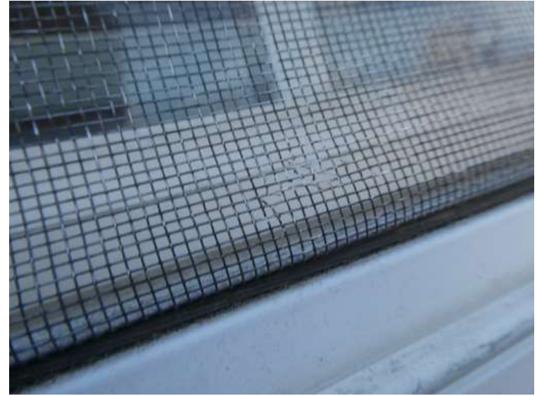
166. Building 07. Tear in a screen.
