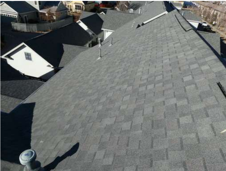
179. Building 07. West test area. No shingles within the test area were bruised by hail.
