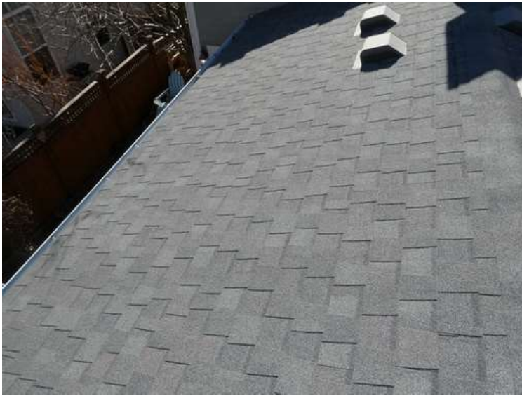
461. Building 20. East test area. No shingles within the test area were bruised by hail.
