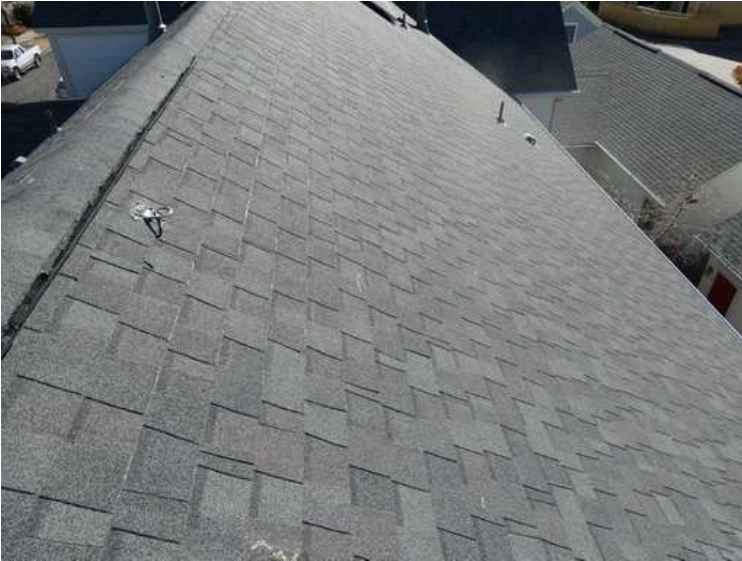
251. Building 10. West test area. No shingles within the test area were bruised by hail.
