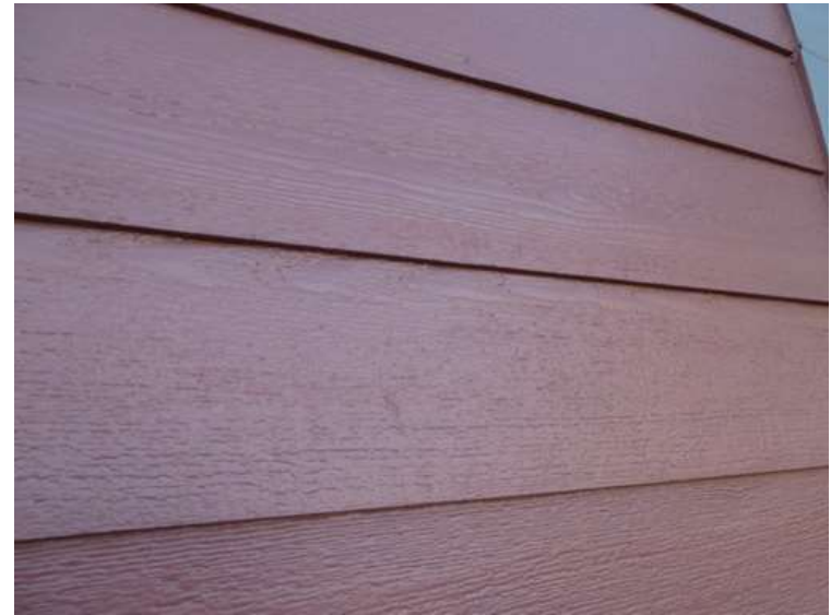
608. Building 25. Paint finishes on fiber cement siding were not chipped by hail.
