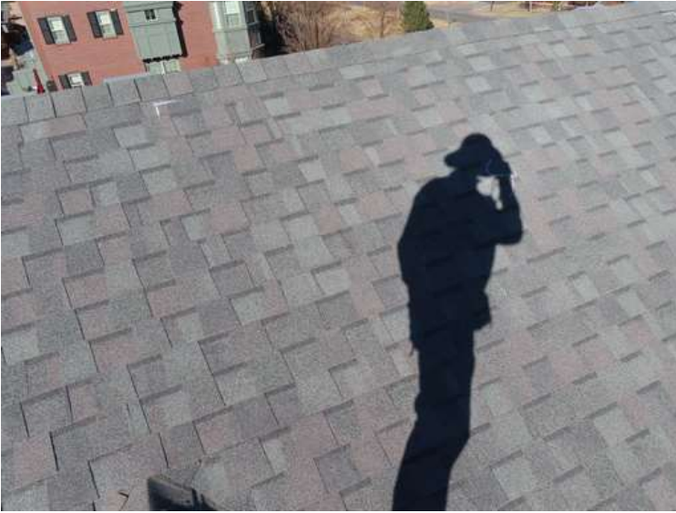
433. Building 19. South test area. No shingles within the test area were bruised by hail.
