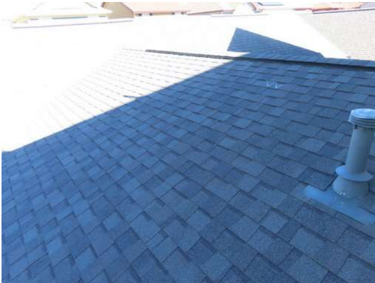
283. Building 12. West test area. No shingles within the test area were bruised by hail.
