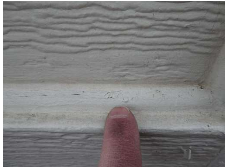
140. Building 06. Chip in paint from hail.
