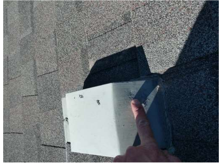
206. Building 08. Dent in an exhaust vent.
