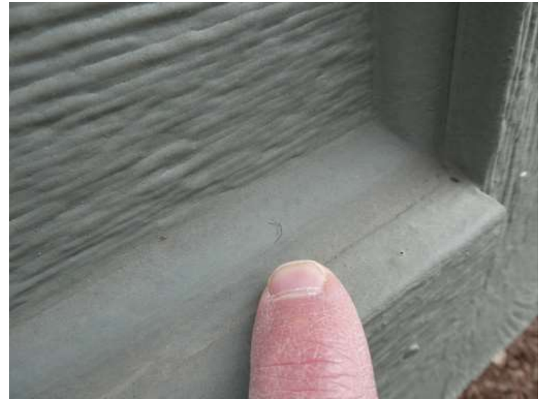
364. Building 16. Chip in paint from hail.
