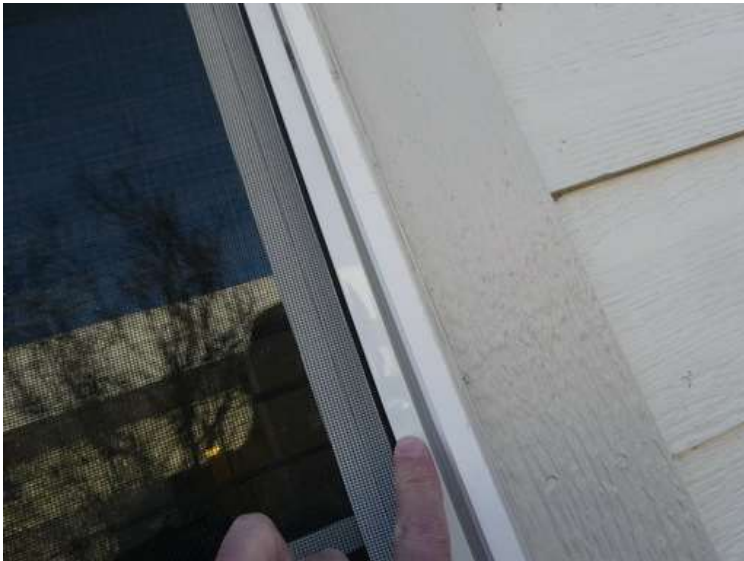
239. Building 10. Dent in a screen frame.
