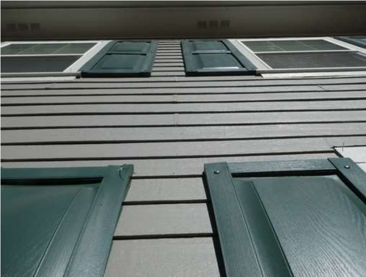
447. Building 20. Fracture in a shutter.
