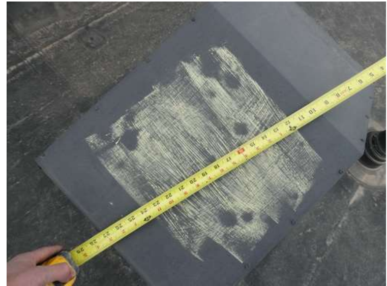
150. Building 06. Dents in an exhaust hood from hail.
