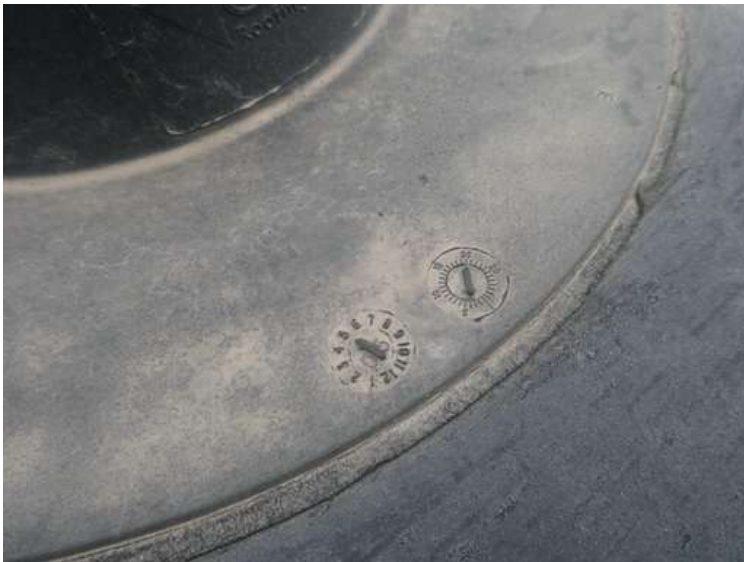
51. Building 02. Flashing boot dated, '05'.
