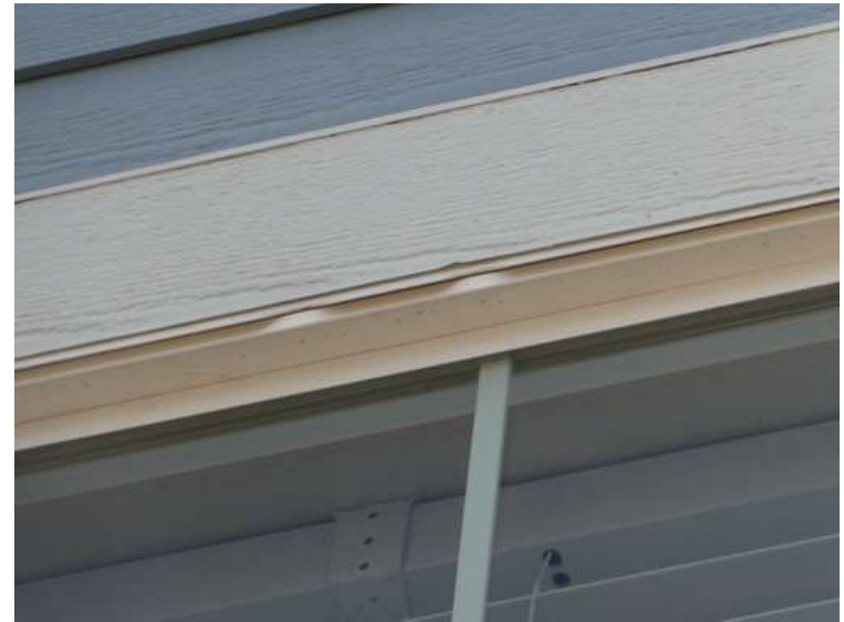
424. Building 19. Fractures in vinyl above the window.
