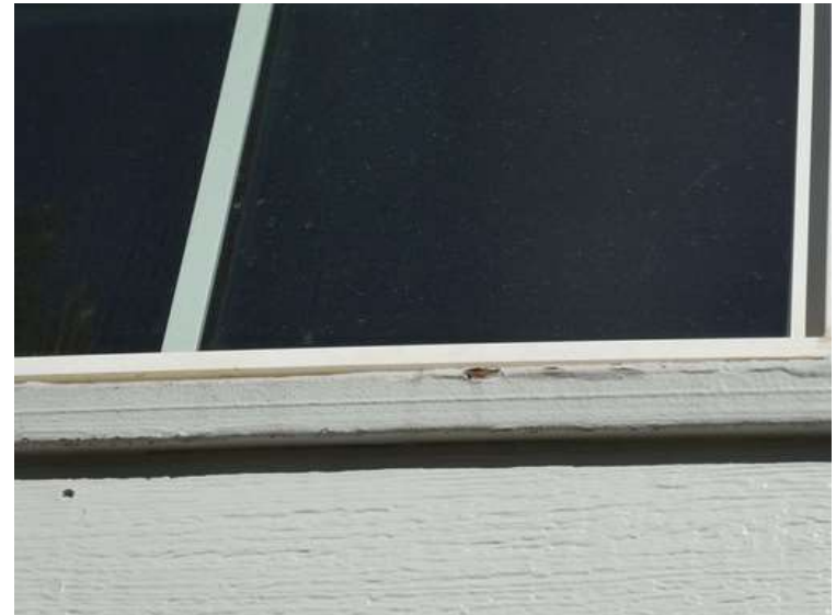
548. Building 23. Chip in paint from hail.
