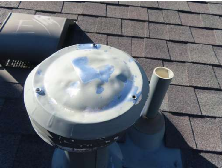
395. Building 17. Dents from hail.
