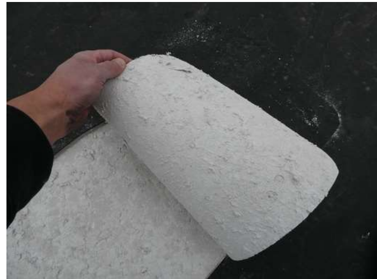
30. Building 01. Facer sheet stuck to the underside of the membrane.
