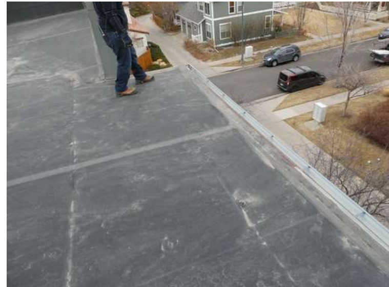
88. Building 03. Roof above the water-stained window opening and warped wood flooring. The deck was soft.
