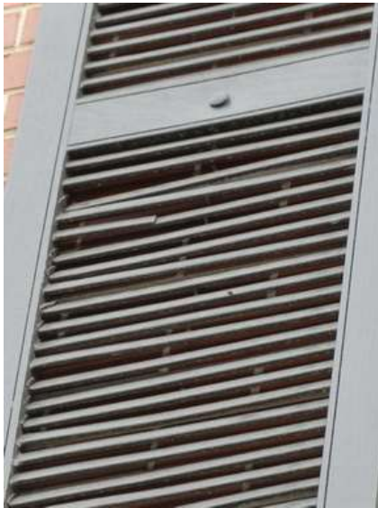
307. Building 14. Fractures in a plastic shutter from hail.
