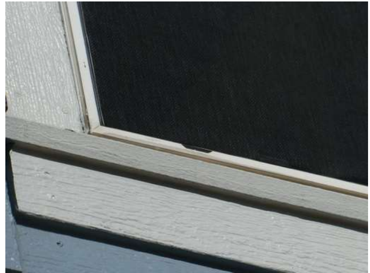
420. Building 19. Fractured window frame.
