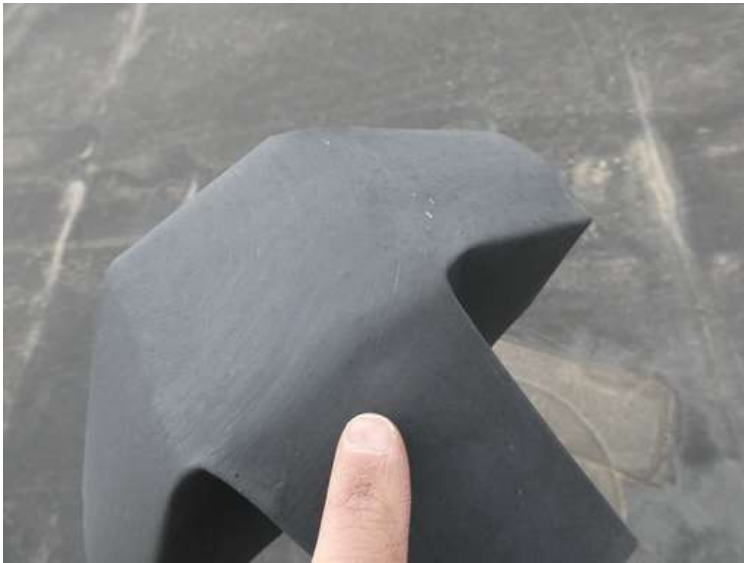
55. Building 02. Dent in a flue cap from hail.
