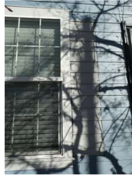
506. Building 22. Missing shutter.
