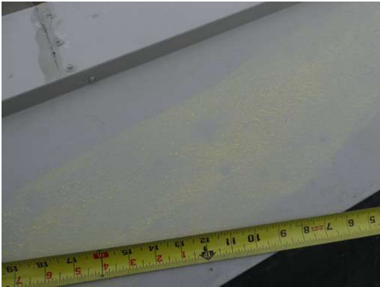
149. Building 06. Dents in coping from hail.
