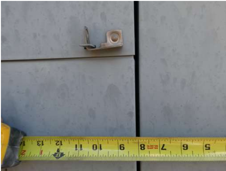
453. Building 20. Spatter marks on an electrical box.
