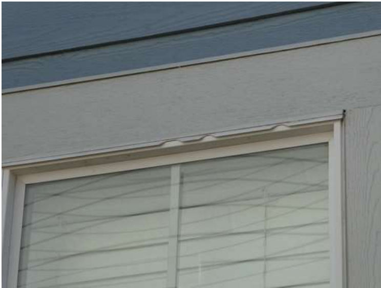
515. Building 22. Fractures in a plastic window frame from hail.
