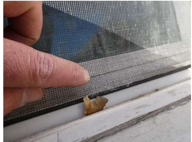
572. Building 24. Tear in a screen.
