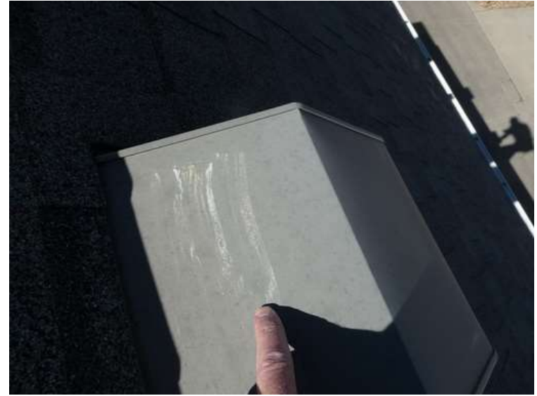
458. Building 20. Dents in an attic vent from hail.
