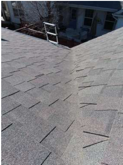
303. Building 13. Shingles draped over a valley were not bruised by hail.
