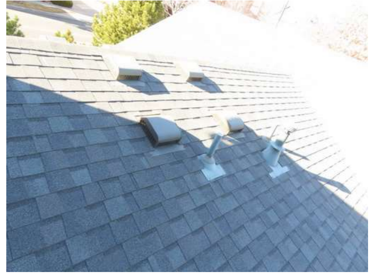
394. Building 17. East test area. No shingles within the test area were bruised by hail.
