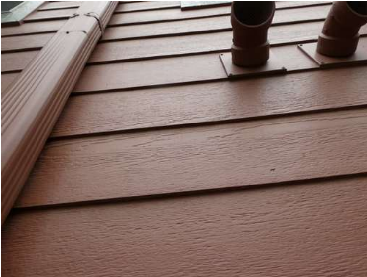
99. Building 04. Paint finishes on fiber cement siding were not chipped by hail.
