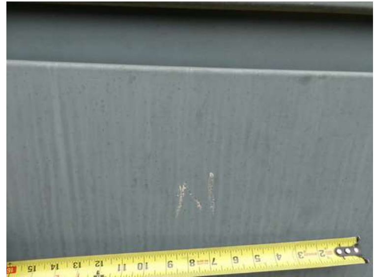
48. Building 02. Faint spatter marks on the north side of a transformer cabinet.
