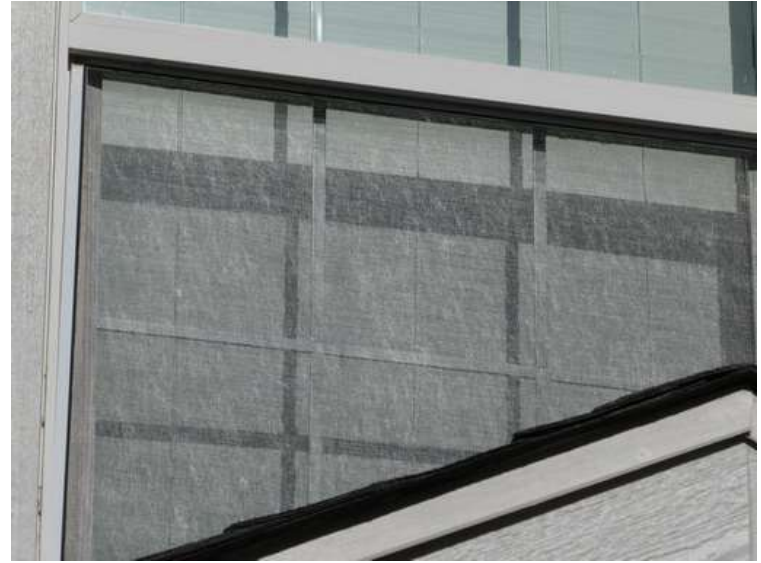
418. Building 19. Tears in a screen.
