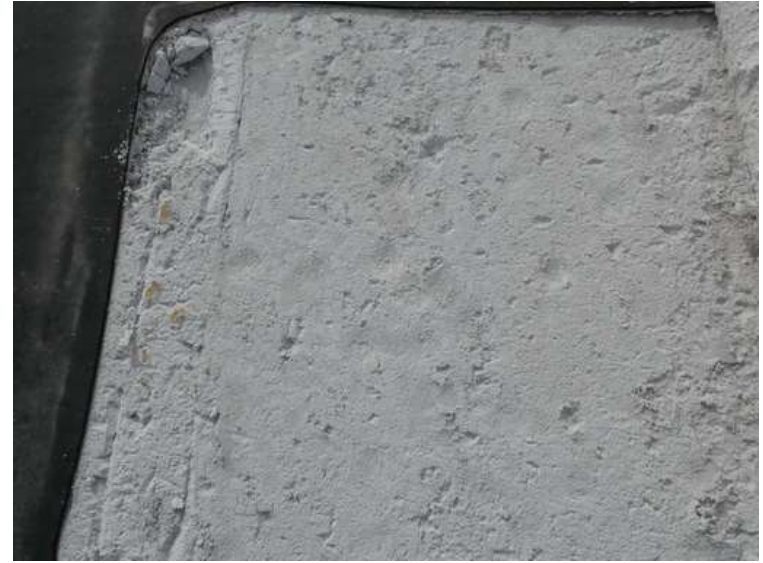
330. Building 14. Dents in the gypsum from hail. The gypsum was powdery.
