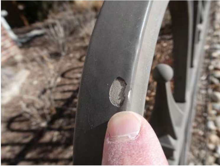
473. Building 21. Mechanical chip in paint.
