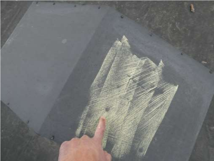
77. Building 03. Dents in an exhaust hood from hail.
