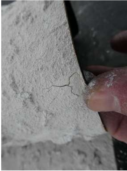
161. Building 06. Tear in the facer sheet from hail.
