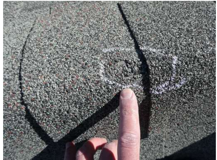
500. Building 21. Bruise in a ridge shingle.
