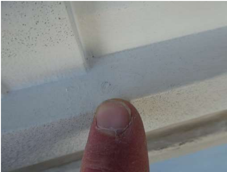
231. Building 09. Chips in paint.
