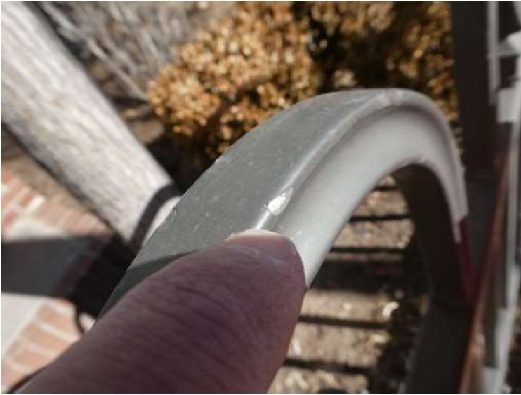
445. Building 20. Scrape in paint on an iron fence.
