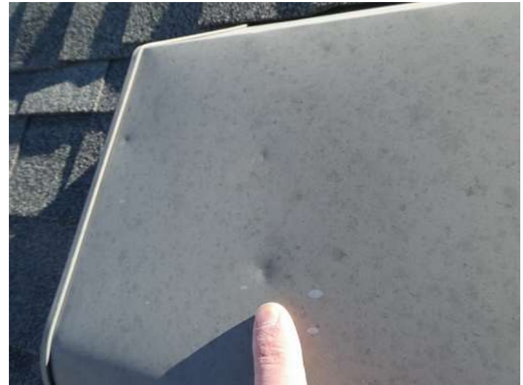
532. Building 22. Dent in an attic vent from hail.
