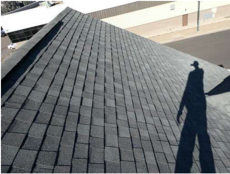
253. Building 10. East test area. No shingles within the test area were bruised by hail.
