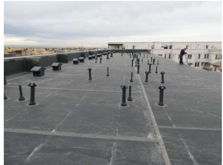
106. Building 04. View looking north. The roof was covered with an adhered EPDM membrane.
