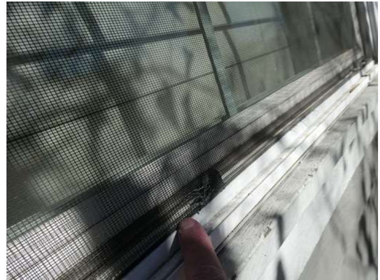
444. Building 20. Tear in a screen.
