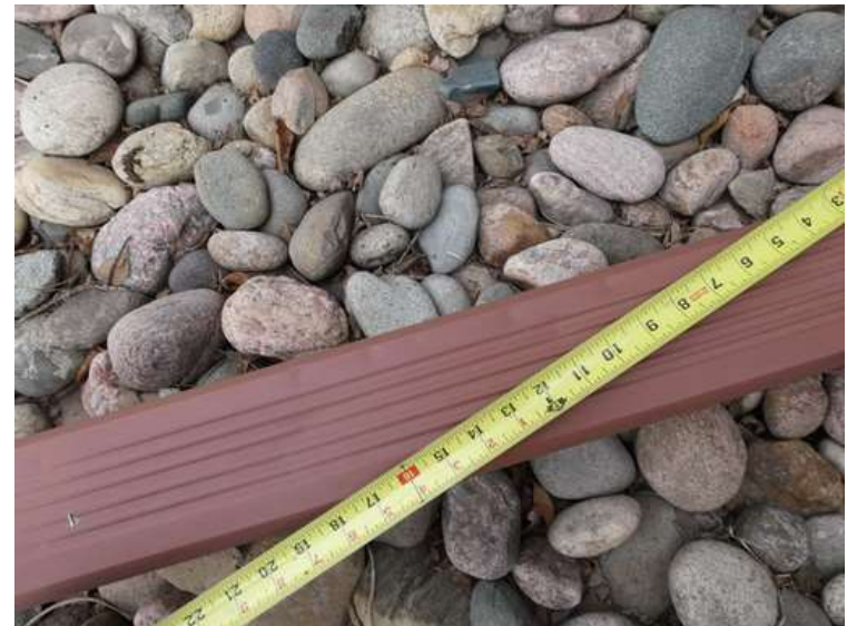
344. Building 15. Dents in a downspout extension from hail.
