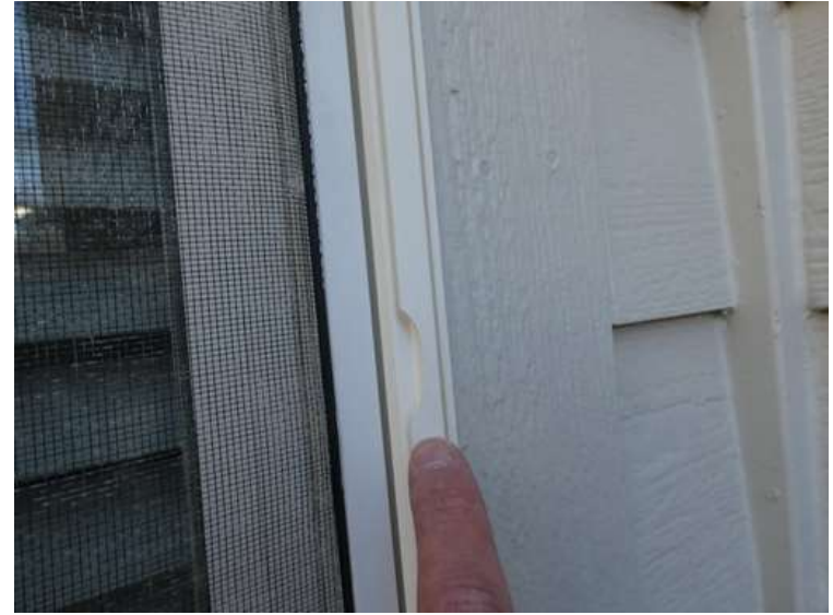
482. Building 21. Fracture in the frame from hail.
