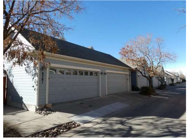
510. Building 22. North elevation. The garage doors were not dented by hail.
