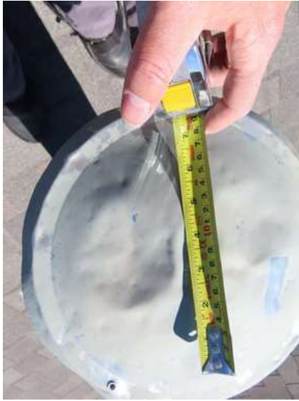
289. Building 12. Dents from hail.
