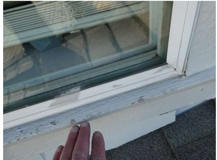
552. Building 23. Chips in paint from hail.
