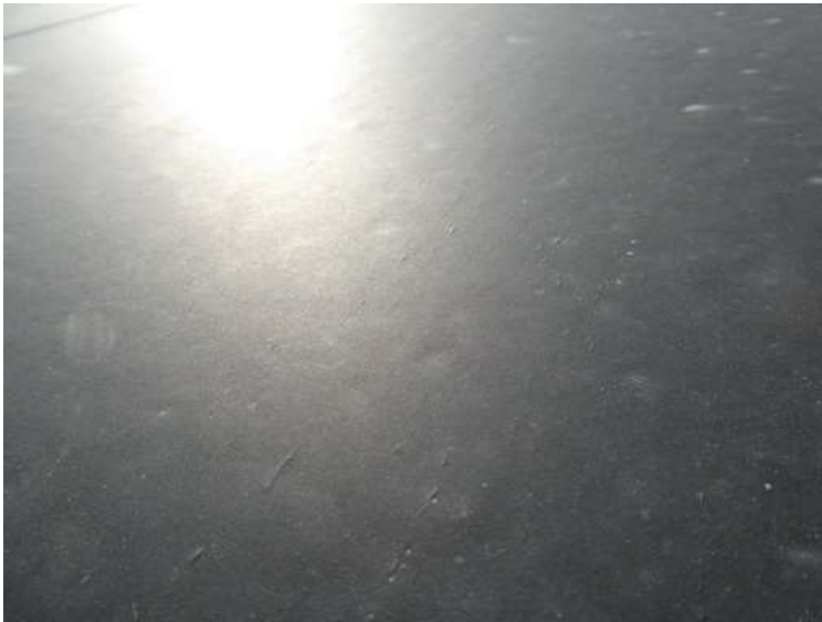
621. Building 25. Dent in the roof surface.
