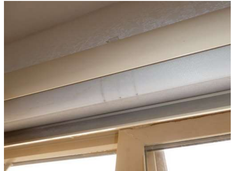
84. Building 03. Water stains.
