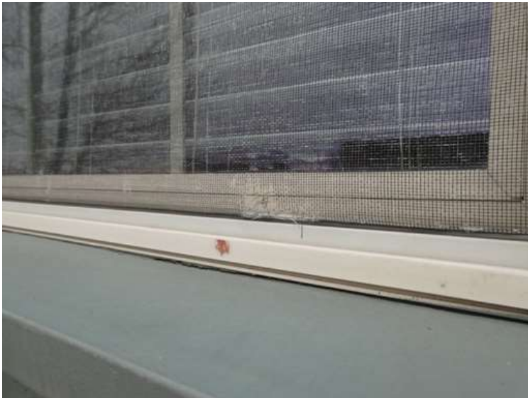
95. Building 04. Tears in a screen.
