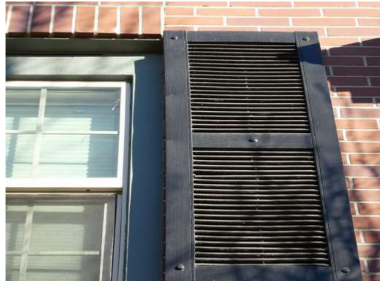
604. Building 25. Fractured shutter.
