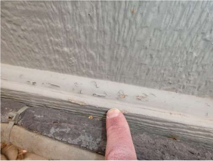
41. Building 02. Chips in paint on a south elevation.
