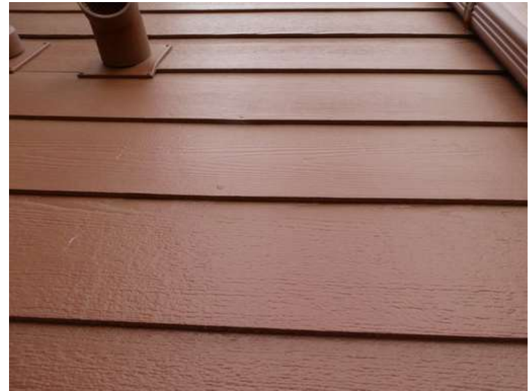
372. Building 16. Paint finishes on fiber cement siding was not fractured by hail.
