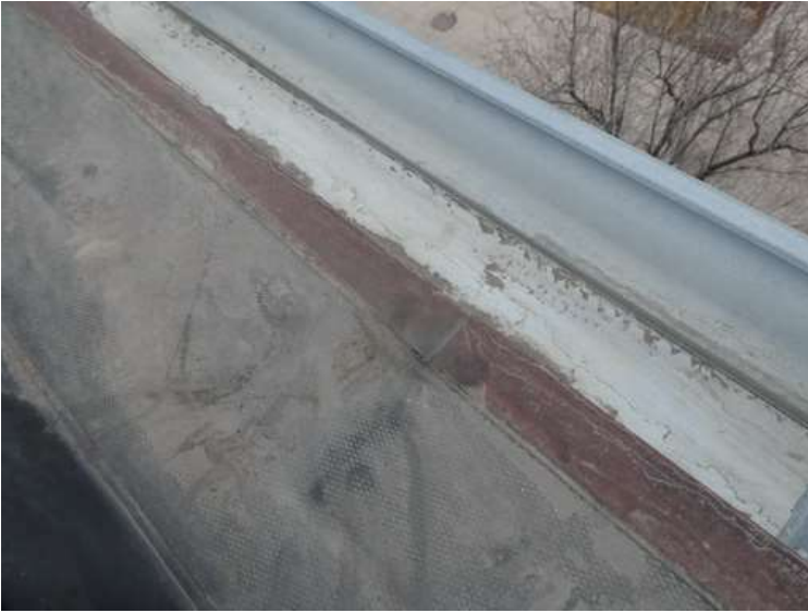
89. Building 03. Joint in edge metal. Edge metal was rusted where water pooled at the perimeter of the roof.
