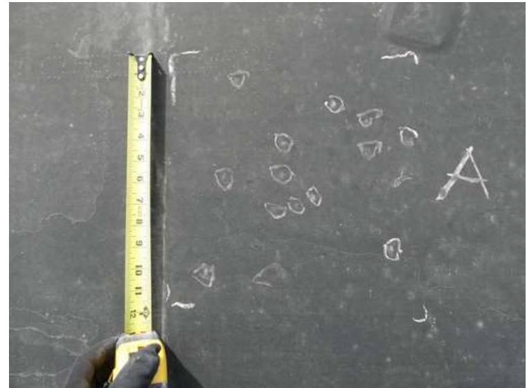
328. Building 14. Membrane area marked for sampling. Circular chalk marks denote dents in the substrate.
