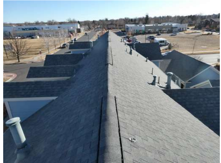
174. Building 07. View looking south. The roof was covered with IR shingles from CertainTeed.
