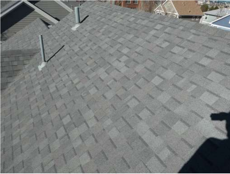
497. Building 21. South test area. Two shingles within the test area were bruised at wrinkles by hail.
