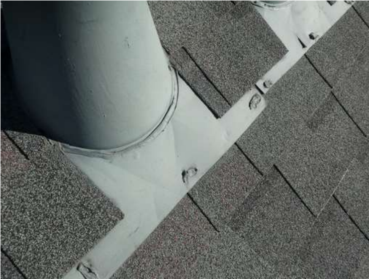
177. Building 07. Re-used base flashing.
