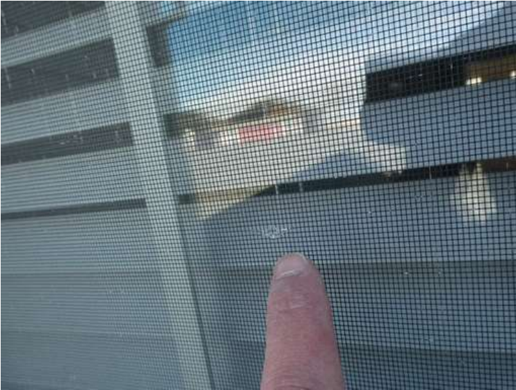
489. Building 21. Tear in a window screen.
