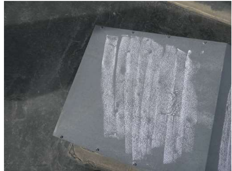
326. Building 14. Dents in a vent hood from hail.
