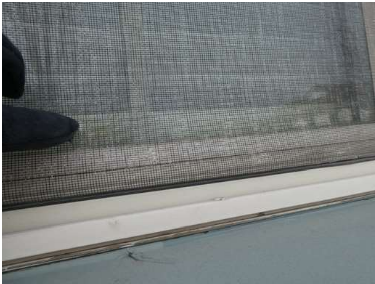
311. Building 14. Tears in a screen from hail.
