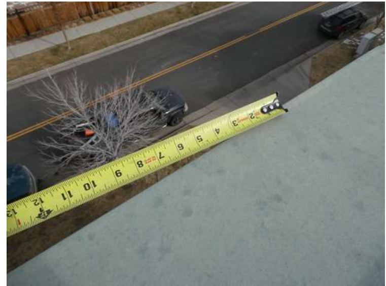
322. Building 14. Spatter marks on coping from recent hail.
