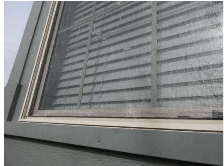
374. Building 16. Tears in a screen from hail.
