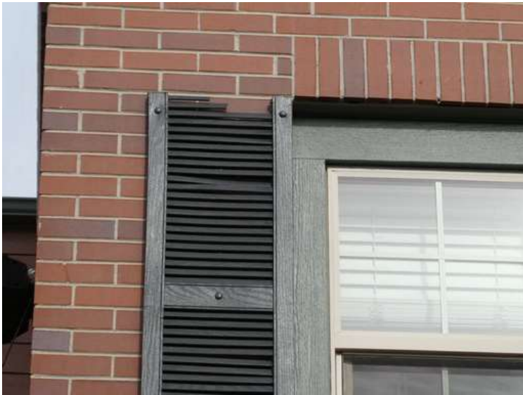
349. Building 15. Fractures in a plastic shutter.
