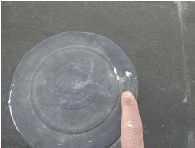
131. Building 05. Dents in a flue cap from hail.
