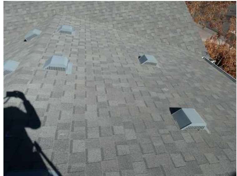
520. Building 22. East test area. Two shingles within the test area were bruised by hail at wrinkles.
