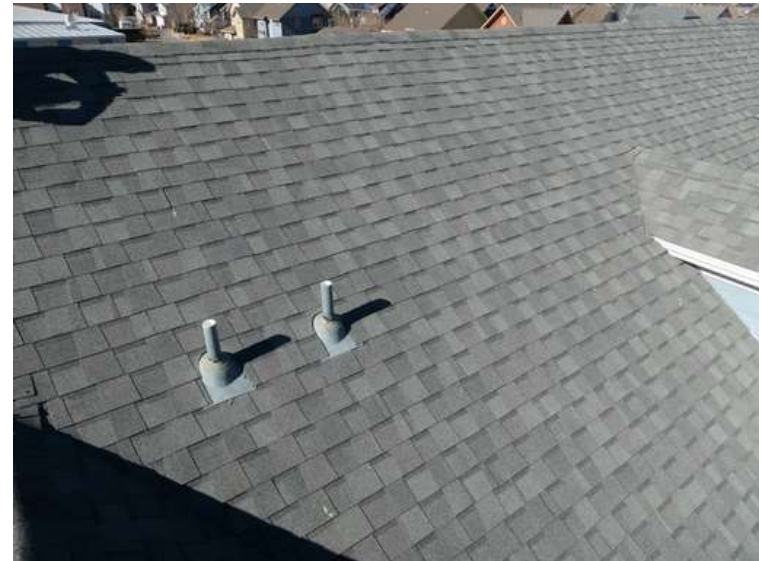
596. Building 24. East test area. No shingles within the test area were bruised by hail.
