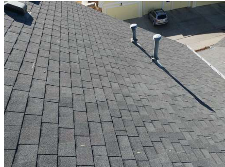
564. Building 23. West test area. No shingles within the test area were bruised by hail.
