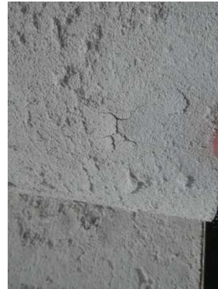
332. Building 14. Tear in the facer sheet adhered to the membrane from hail.
