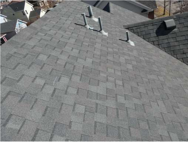
465. Building 20. South test area. No shingles within the test area were bruised by hail.
