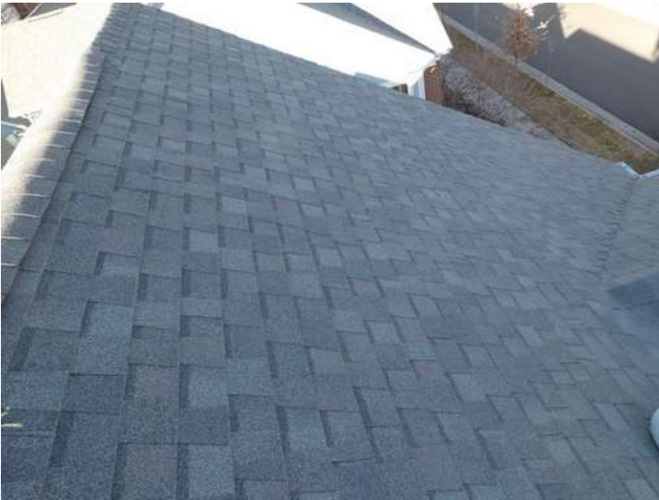
211. Building 08. East test area. No shingles within the test area were bruised by hail.
