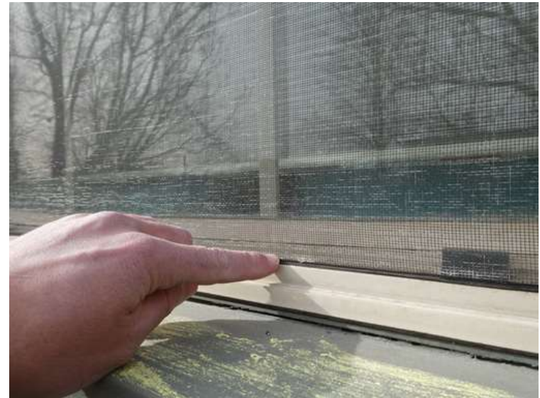
336. Building 15. Small tear in a screen.
