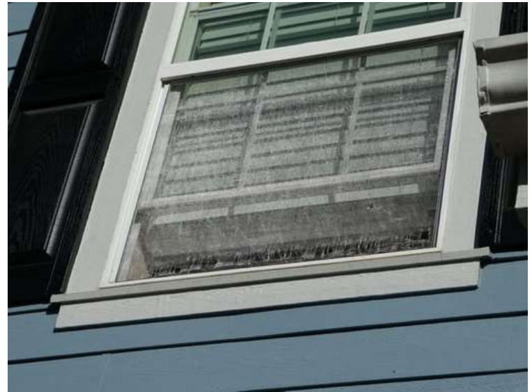
504. Building 22. Tears in a screen from hail.
