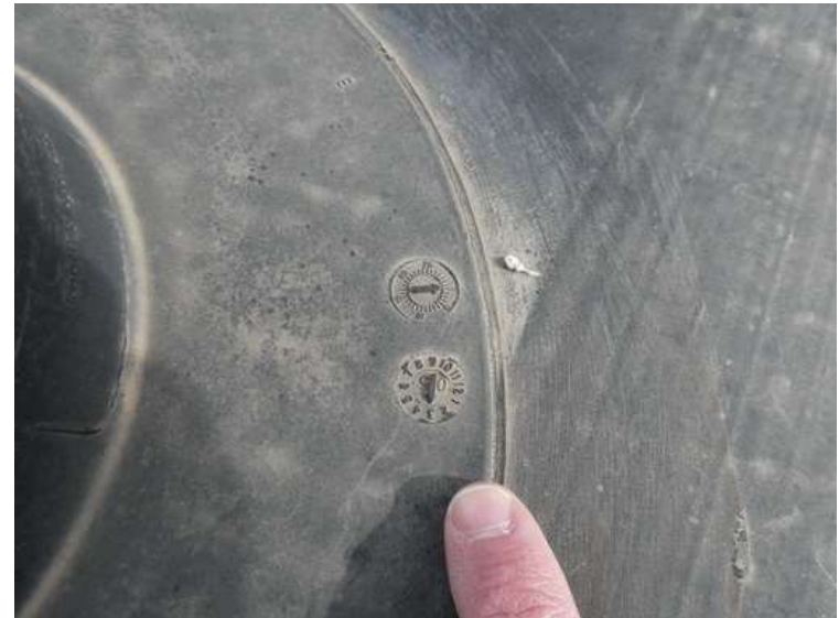
352. Building 15. Flashing boot dated, '05'.
