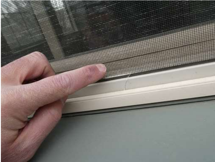
37. Building 02. Tear in a screen from hail.
