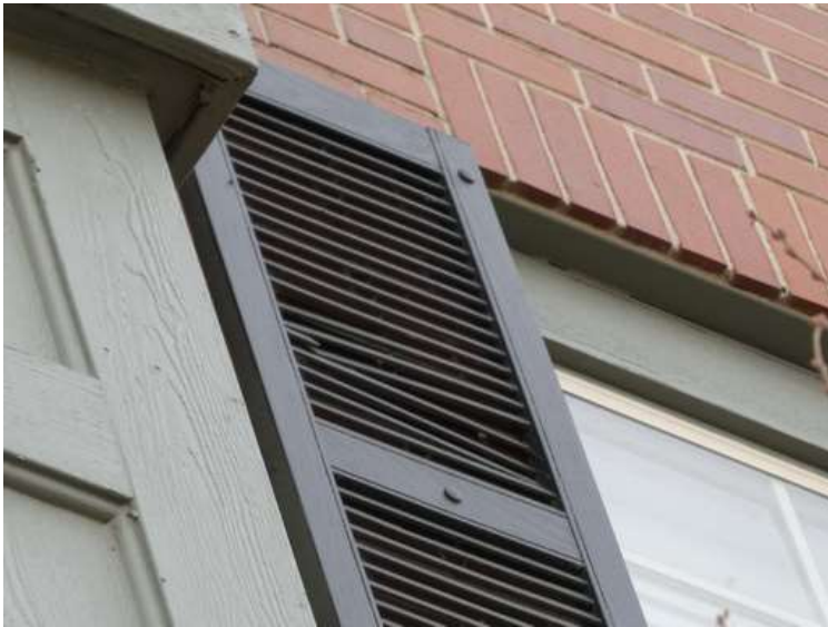
339. Building 15. Fractures in a shutter.
