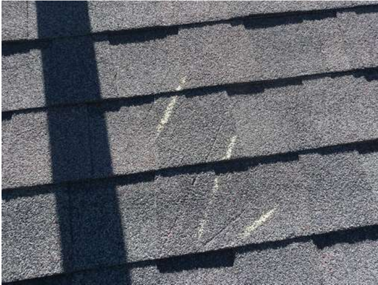
593. Building 24. Knife cuts.
