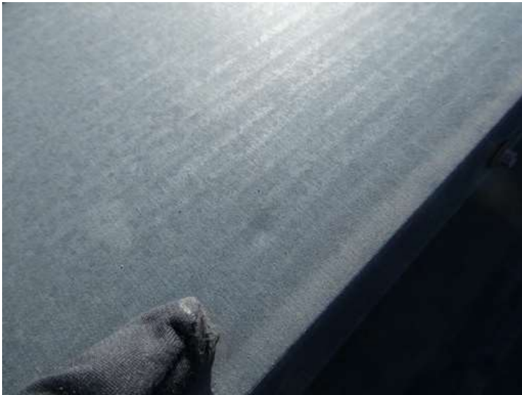
619. Building 25. Dent in coping from hail.
