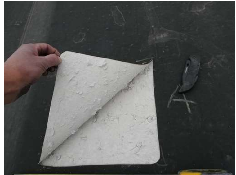
154. Building 06. The substrate provided little resistance to uplift.
