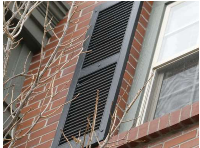
64. Building 03. Fractured shutter.
