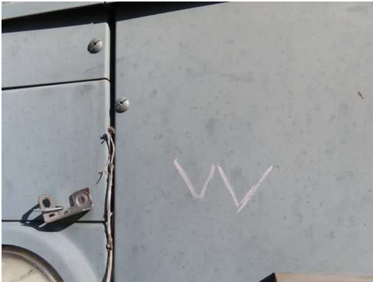
389. Building 17. Spatter marks on an electrical box.
