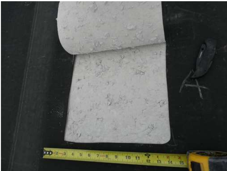
155. Building 06. Gypsum substrate was soft and deteriorated.
