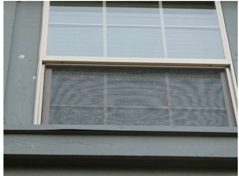
368. Building 16. Tears in a screen from hail.
