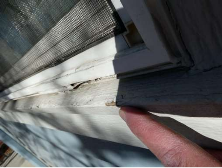
505. Building 22. Chip in paint from hail.
