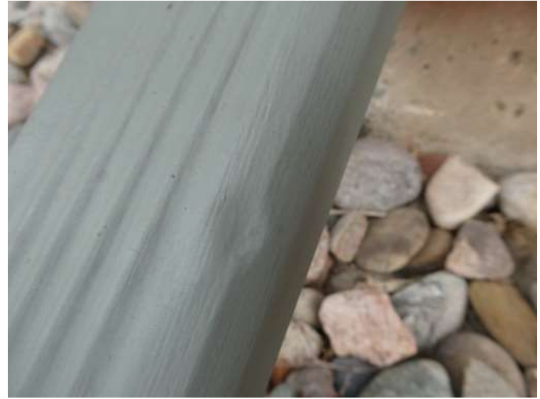
10. Building 01. Dent in a downspout extension from hail.
