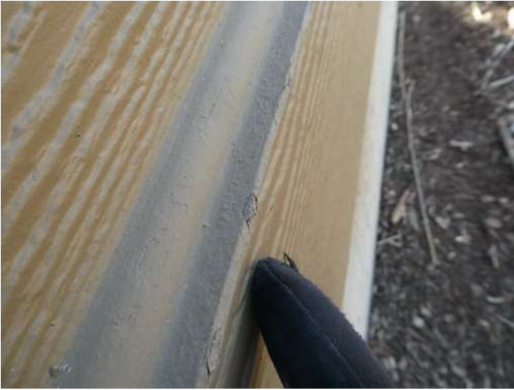
637. Building 26. Chips in paint from hail.
