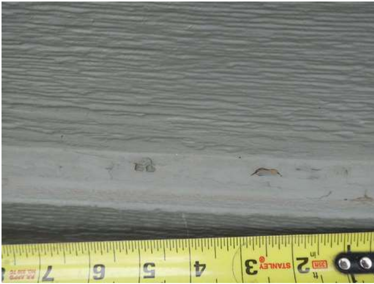
13. Building 01. Chips in paint from hail.
