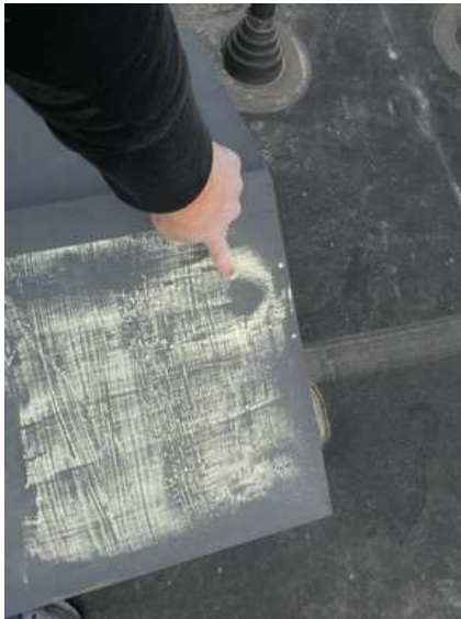
379. Building 16. Dent in an exhaust hood from hail.
