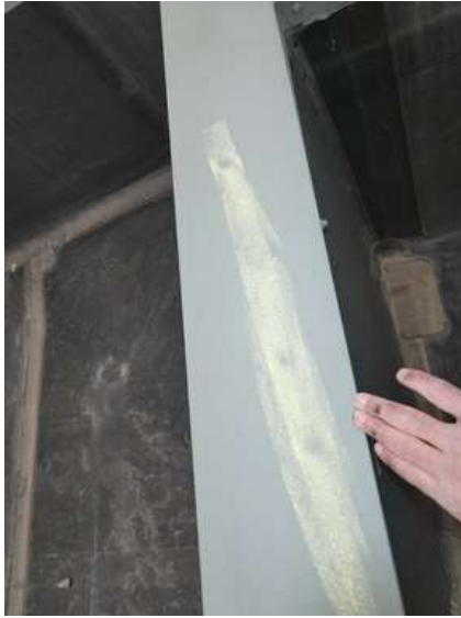
53. Building 02. Dents in a metal cap.
