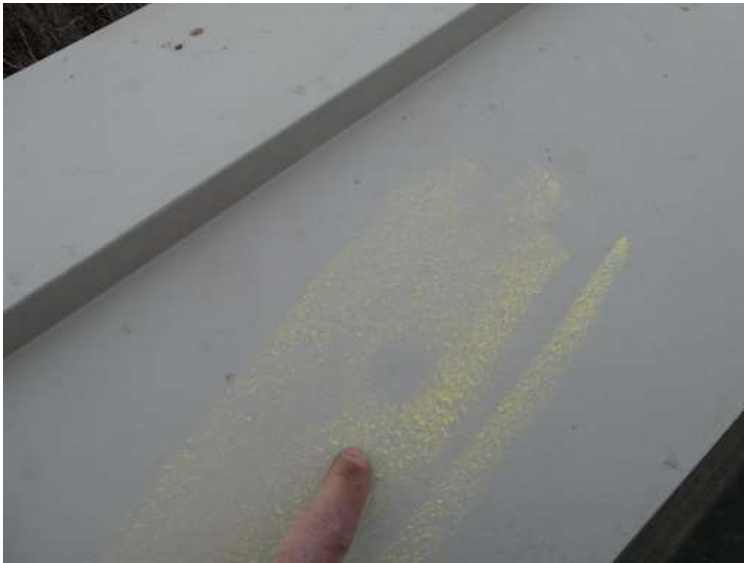
129. Building 05. Dent in coping from hail.
