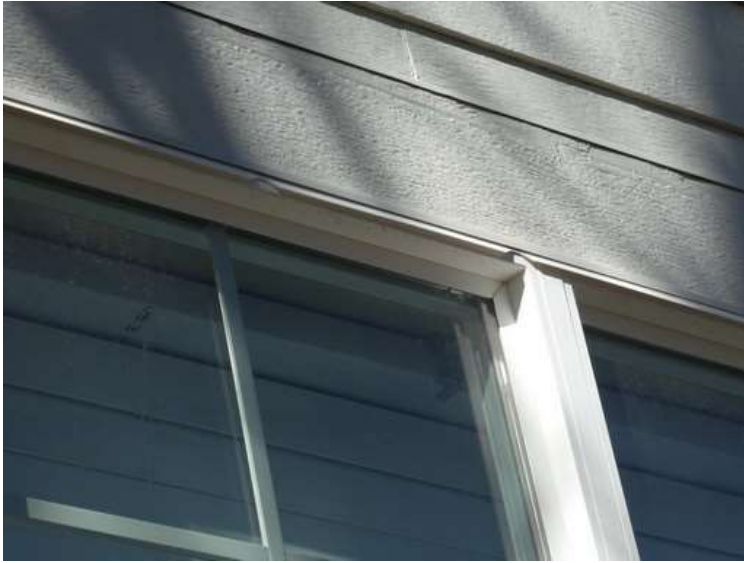
485. Building 21. Fractures in the vinyl frame from hail.
