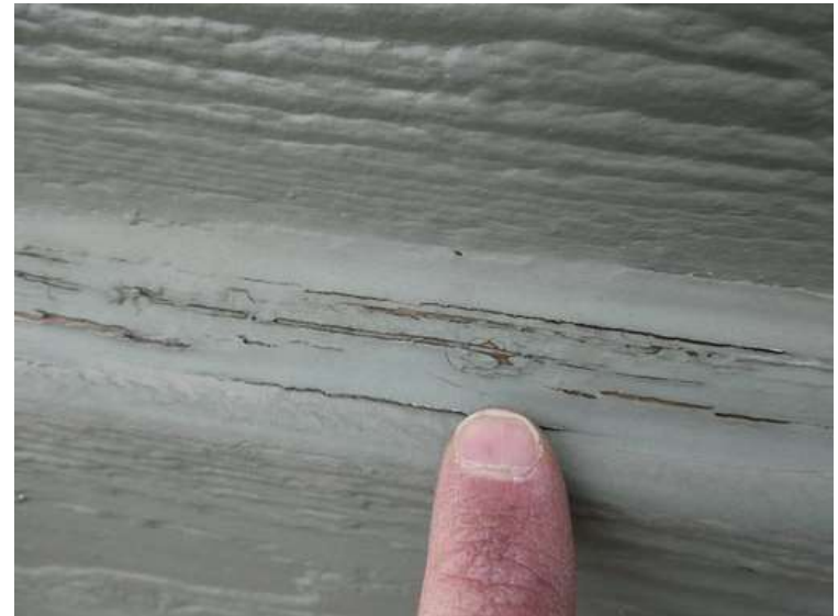
104. Building 04. Chips in paint from hail.
