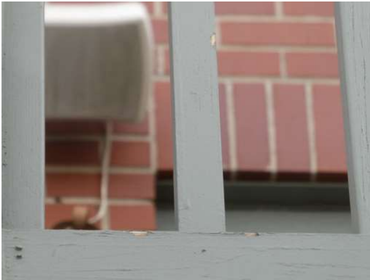
341. Building 15. Chips in paint on a railing.
