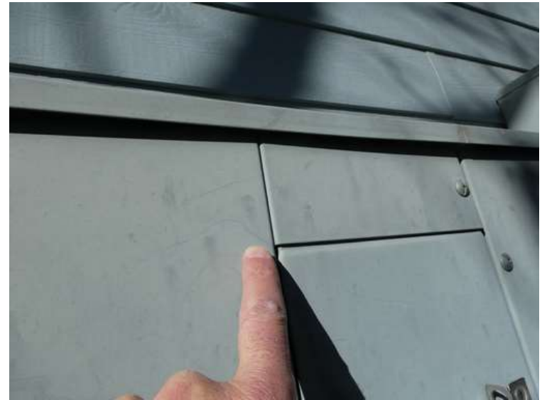
508. Building 22. Spatter marks on an electrical box from hail.
