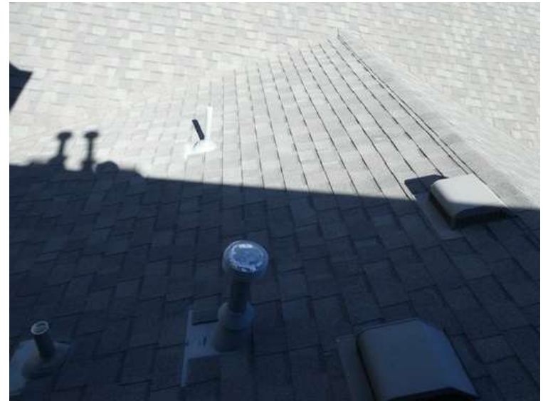
460. Building 20. West test area. No shingles within the test area were bruised by hail.
