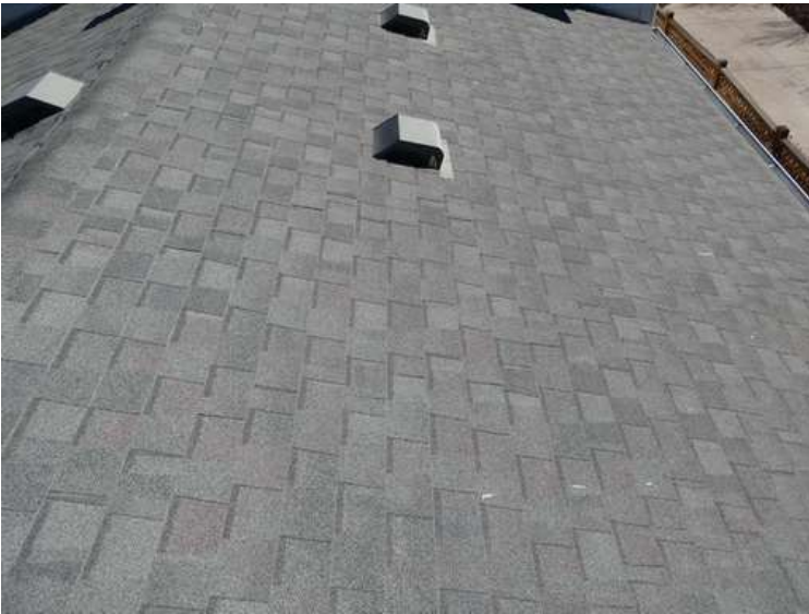
567. Building 23. South test area. No shingles within the test area were bruised by hail.
