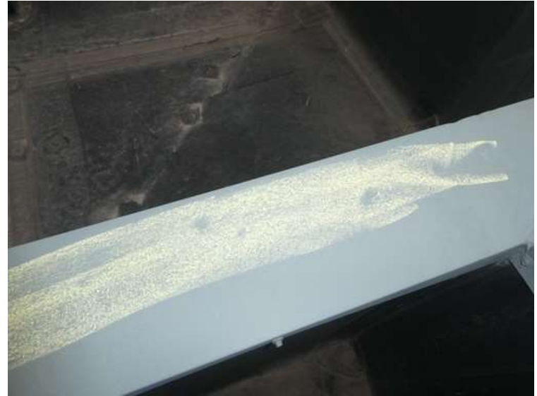
20. Building 01. Dents in a steel cap from hail.
