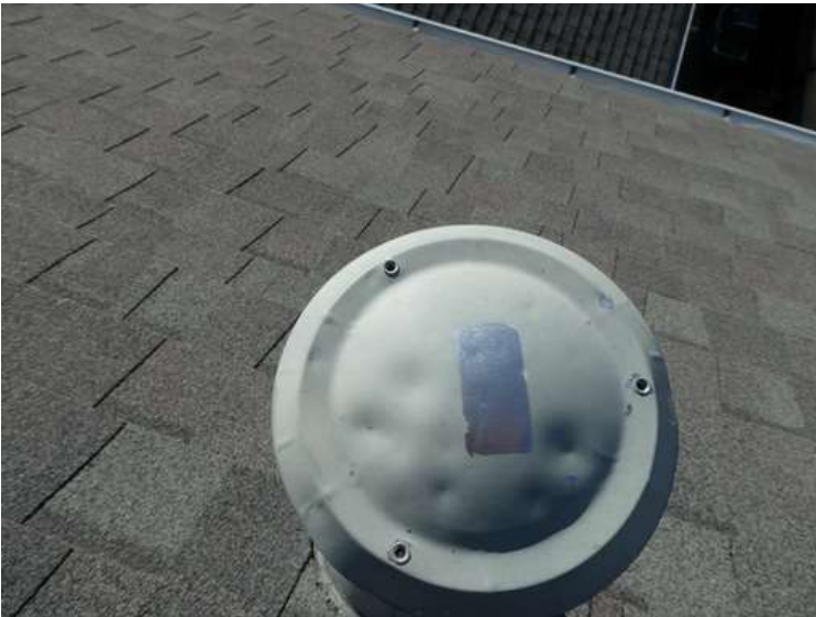
175. Building 07. Dents in a flue cap from hail.
