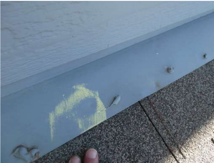
587. Building 24. Dent in headwall flashing.
