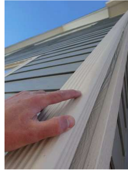
514. Building 22. Dent in a downspout.
