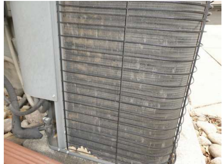
44. Building 02. Dents in condenser fins from hail.
