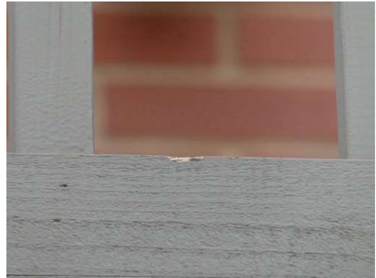
6. Building 01. Chip in paint on a railing.
