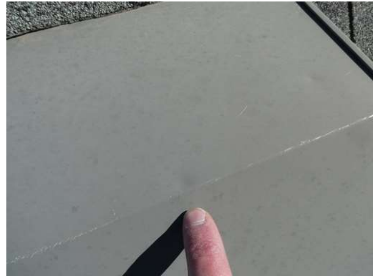
600. Building 24. Dent from hail.
