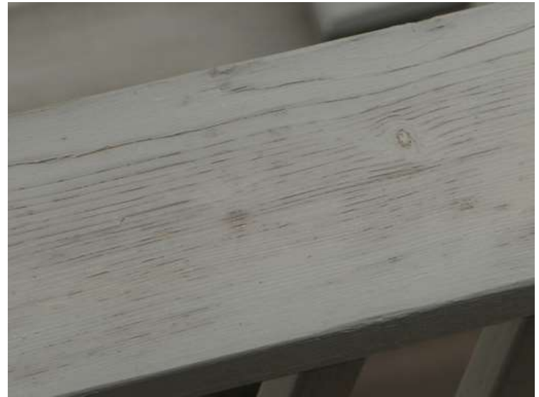
60. Building 02. Scuffs in paint on a railing from hail.
