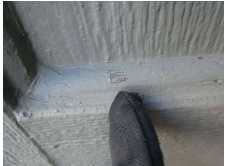
612. Building 25. Chip in paint on a west elevation.
