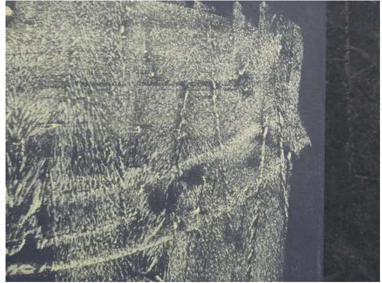
18. Building 01. Dents in an exhaust hood from hail.
