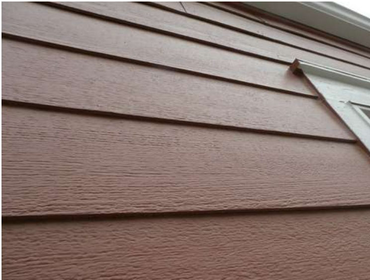
119. Building 05. Paint on fiber cement siding was not chipped by hail.
