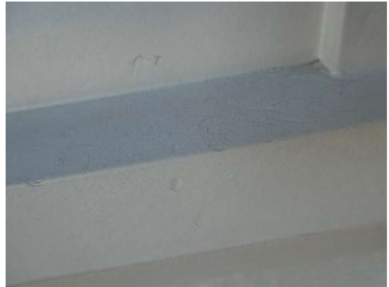
208. Building 08. Chip in paint from hail.
