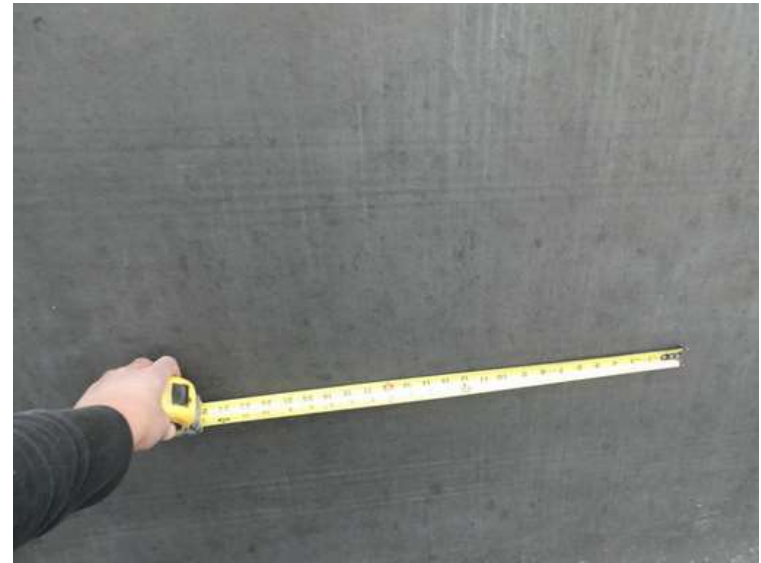
128. Building 05. Spatter marks on membrane turned up a parapet.
