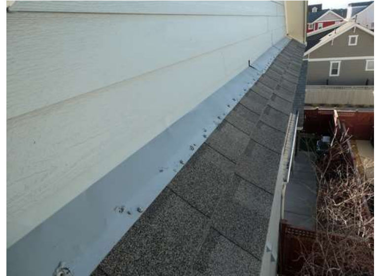
178. Building 07. Re-used headwall flashing.
