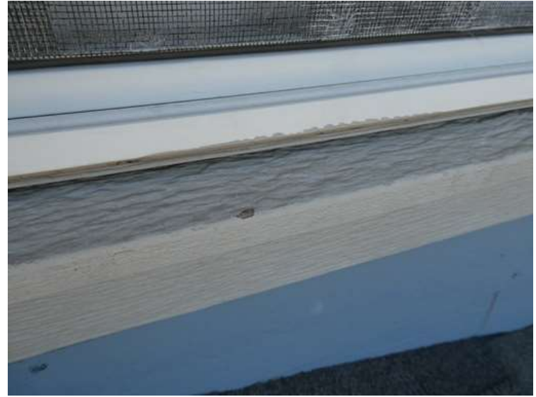
222. Building 09. Chip in paint on a sill.
