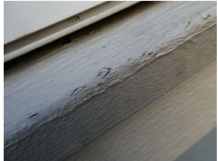
168. Building 07. Chip in paint finish on a windowsill.
