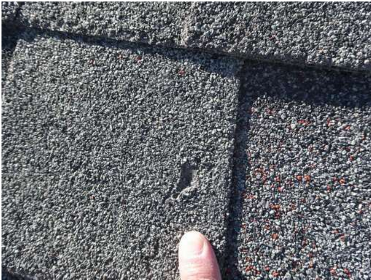
255. Building 10. Mechanical gouge.
