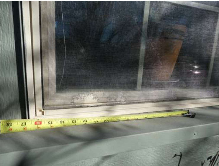
603. Building 25. Tears in a screen.
