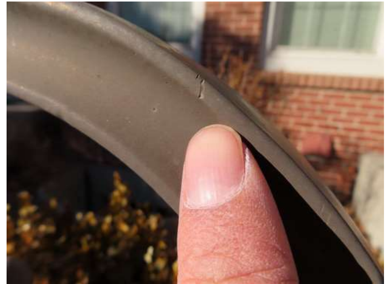
404. Building 18. Scrape in paint on an iron fence.
