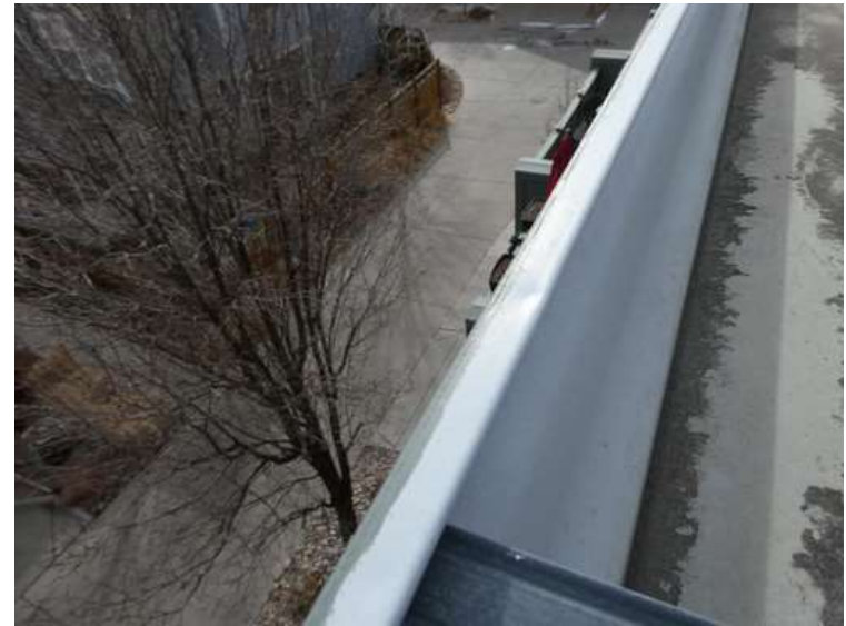
324. Building 14. Dent in a gutter from hail.
