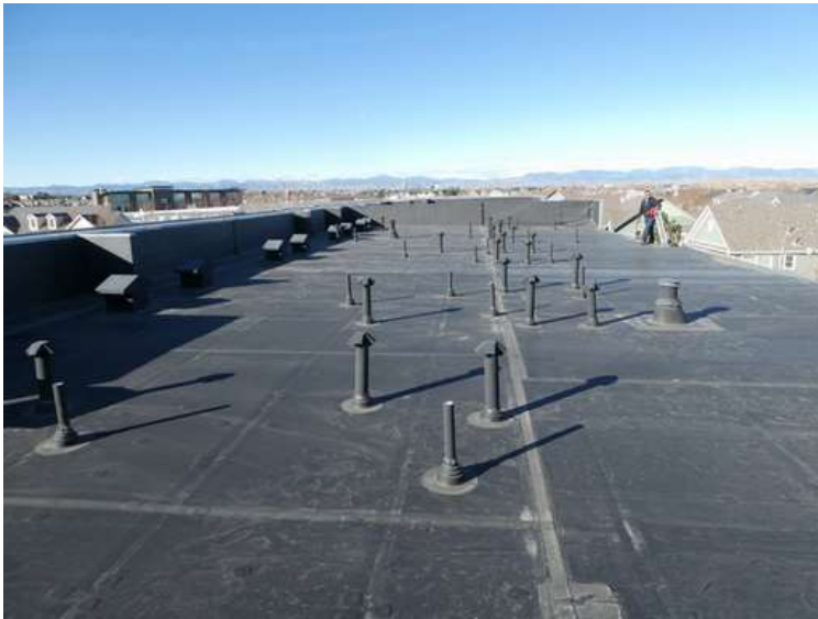
615. Building 25. View looking west. The roof was covered with an adhered EPDM membrane.
