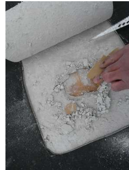
32. Building 01. The roof consisted of a plywood or OSB deck, a layer of gypsum board, and the adhered EPDM membrane.
