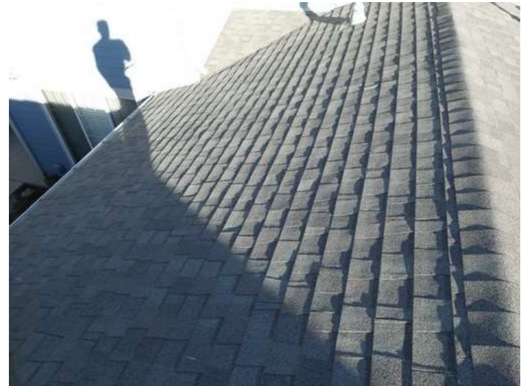
184. Building 07. North test area. No shingles within the test area were bruised by hail.
