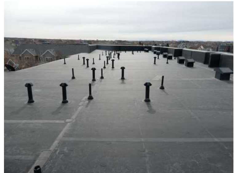
376. Building 16. View looking south. The roof was covered with an adhered EPDM membrane.
