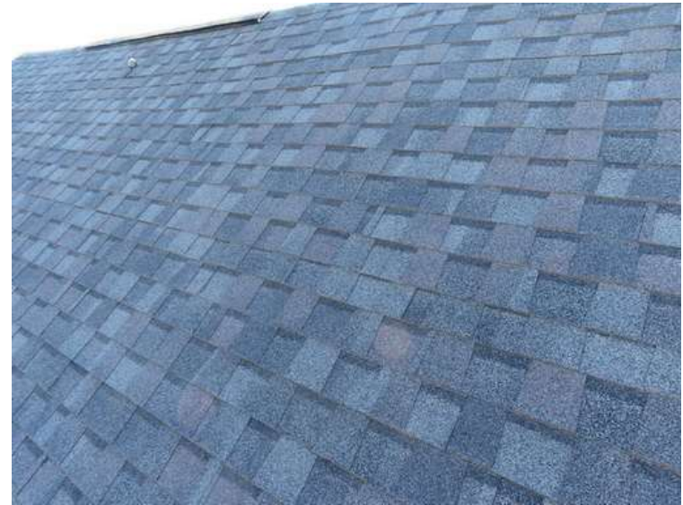
300. Building 13. North test area. No shingles within the test area were bruised by hail.
