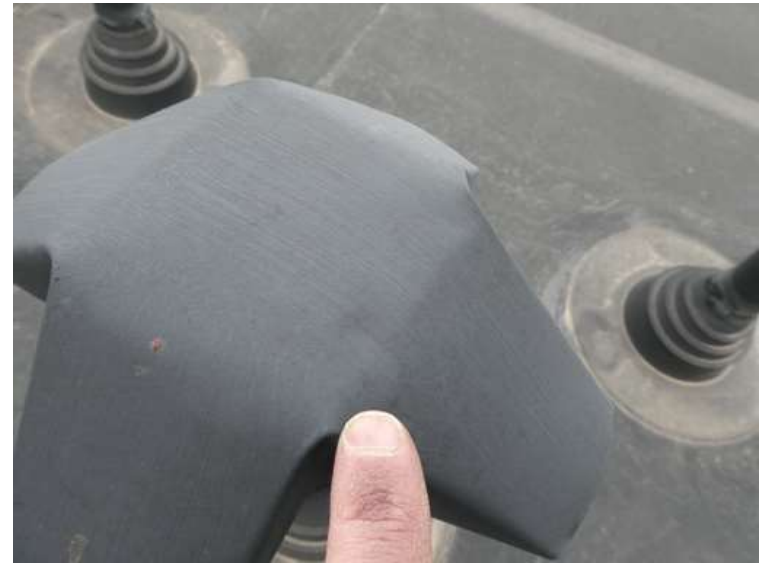
132. Building 05. Dent in a flue cap from hail.
