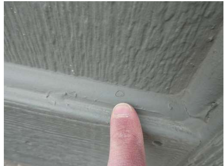
8. Building 01. Chip in paint from hail.
