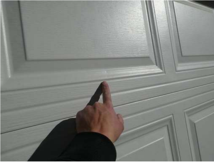
193. Building 08. Dent in a garage door from hail.
