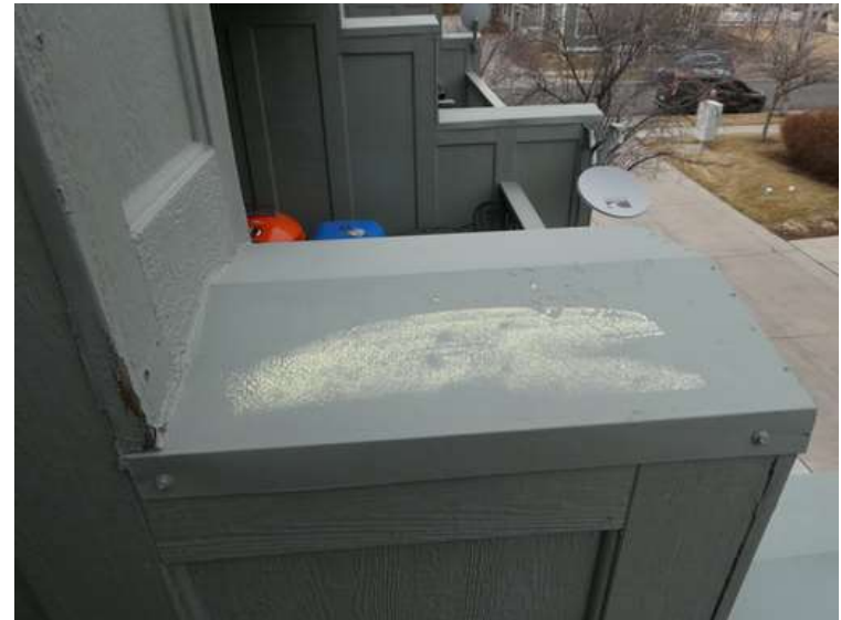
72. Building 03. Dents in a painted steel cap from hail.
