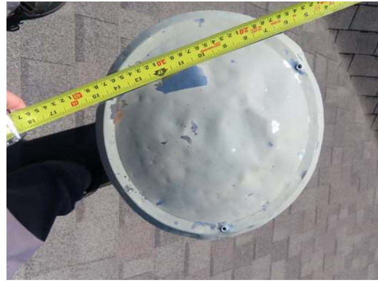
270. Building 11. Dents in a flue cap from hail.
