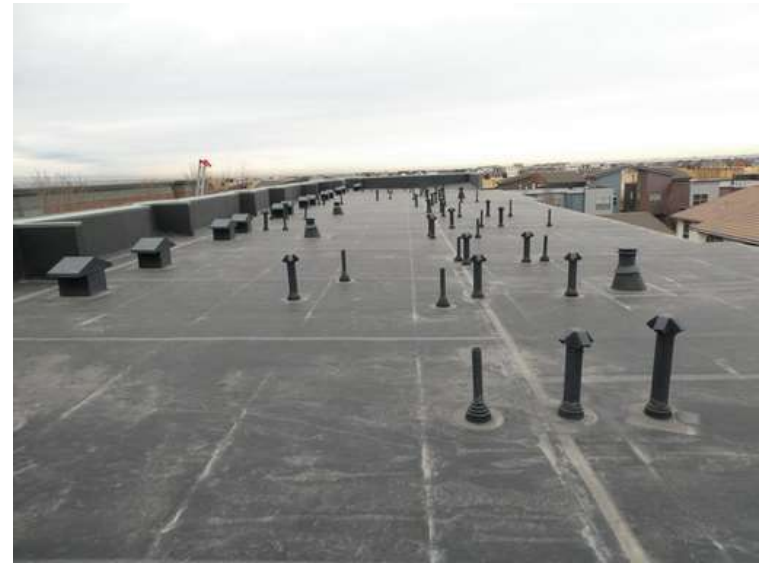
50. Building 02. View looking north. The roof was covered with an adhered EPDM membrane.
