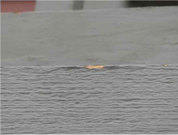
9. Building 01. Chip in paint from hail.
