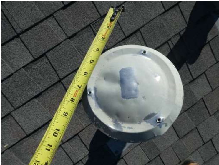
563. Building 23. Dents in a flue cap from hail.
