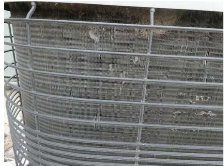
100. Building 04. Small dents in condenser fins.
