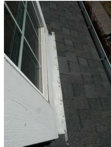
496. Building 21. Re-used headwall flashing.
