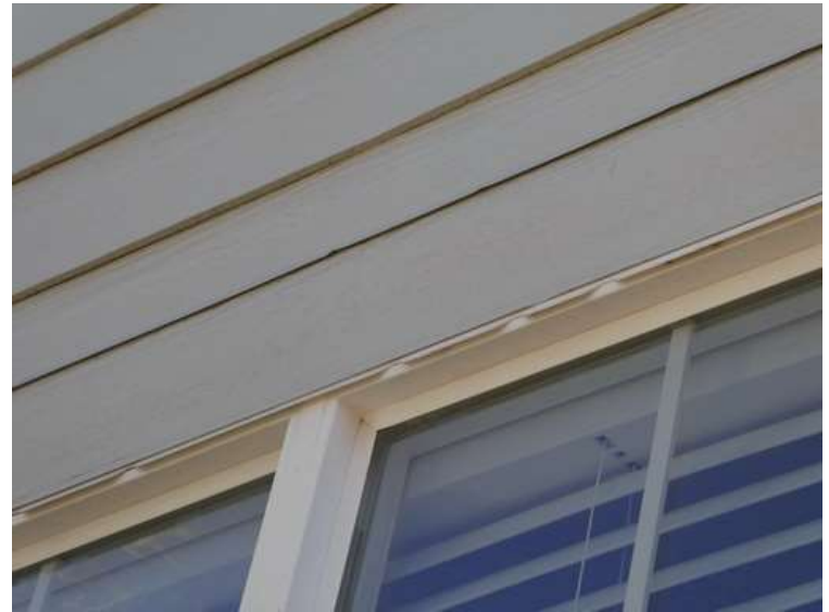
476. Building 21. Fractures in a vinyl window frame from hail.
