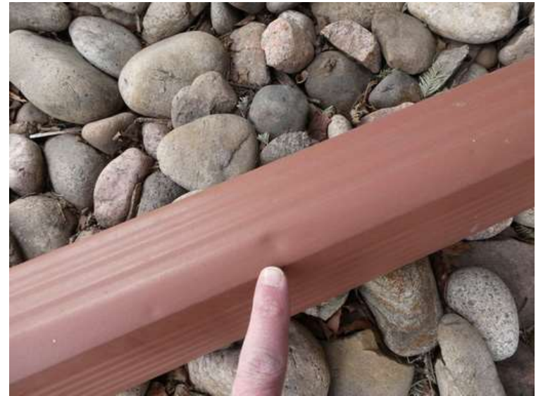
370. Building 16. Dent in a downspout extension from hail.
