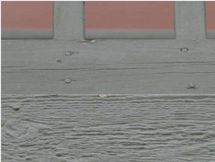
67. Building 03. Chips in paint from hail.
