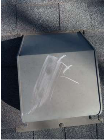
413. Building 18. Dents in an attic vent from hail.
