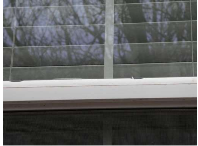
142. Building 06. Beading fractured by hail.
