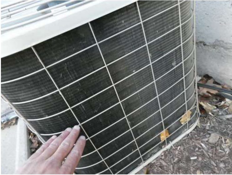
577. Building 24. Small dents in condenser fins from hail.
