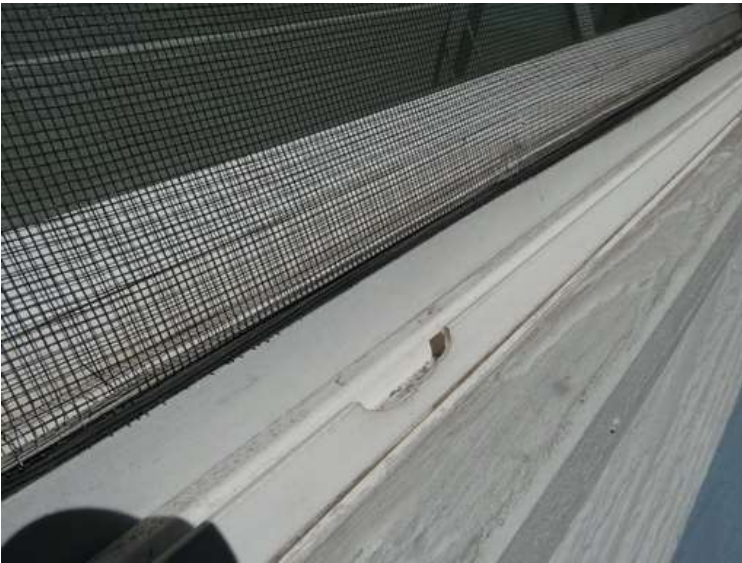
419. Building 19. Fractured frame.
