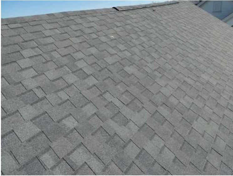
233. Building 09. West test area. No shingles within the test area were bruised by hail.
