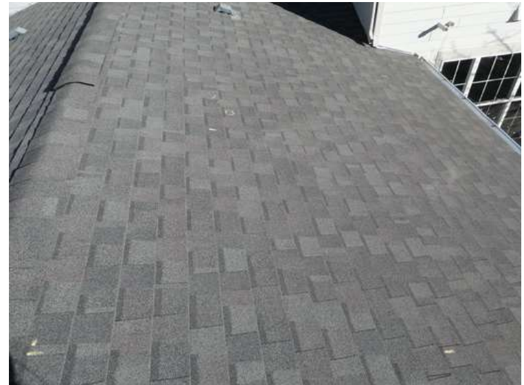
200. Building 08. South test area. One shingle within the test area was bruised by hail.
