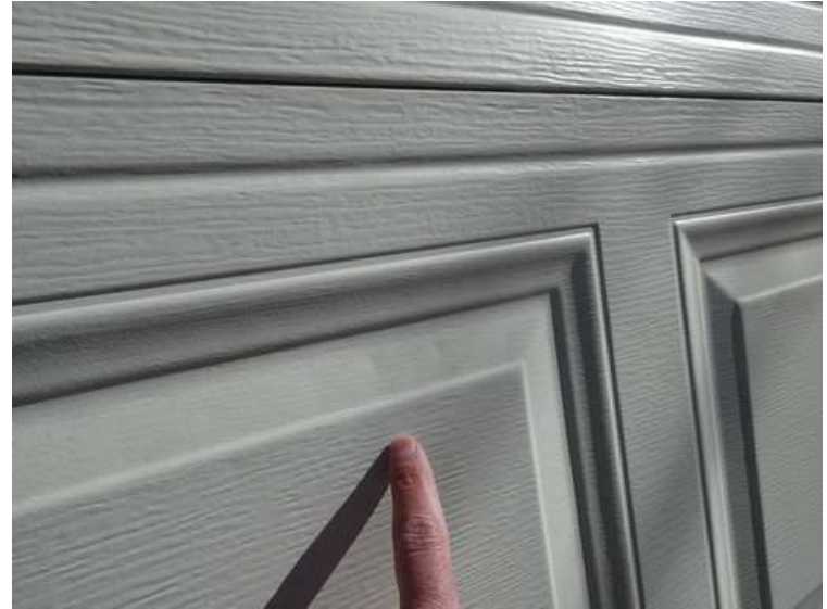
242. Building 10. Dents in a garage door.
