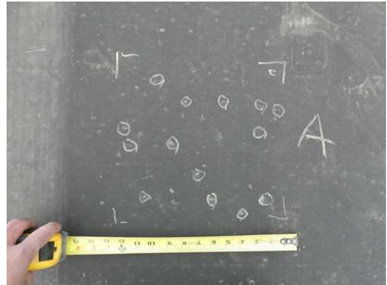
152. Building 06. Test area. Circular chalk marks denote dents in the substrate.
