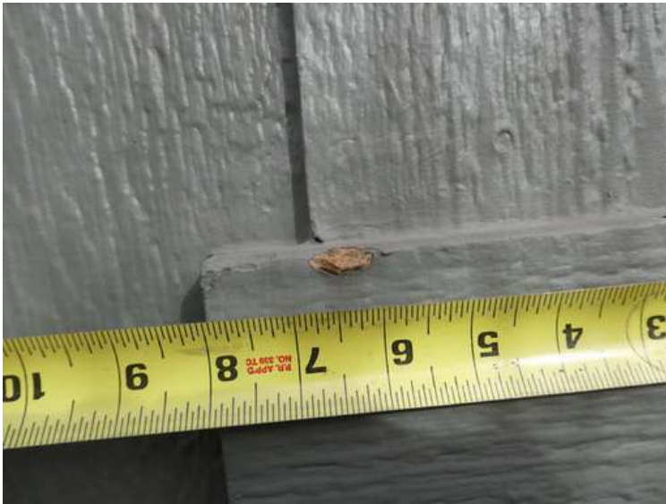
317. Building 14. Chip in paint from hail.
