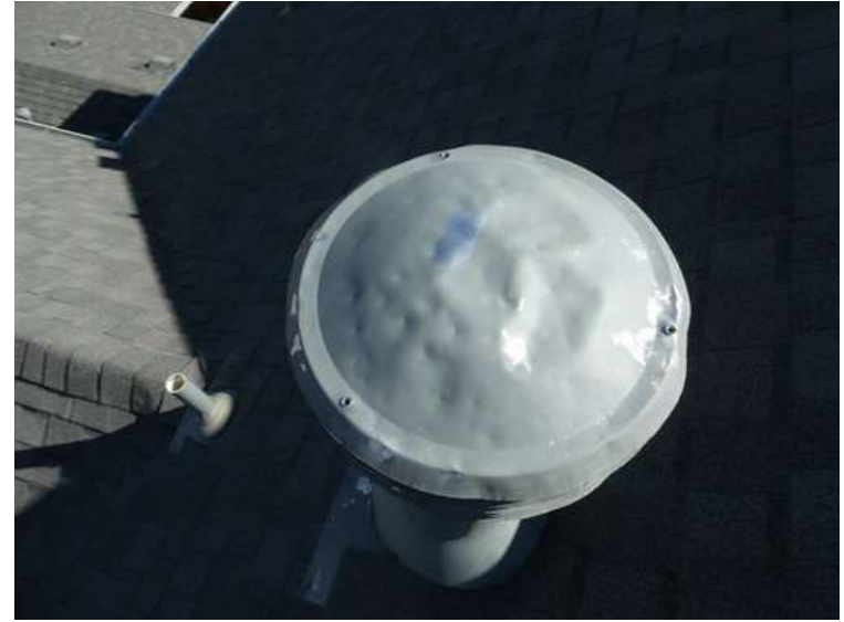
494. Building 21. Dents from hail.
