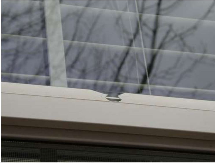
141. Building 06. Beading fractured by hail.
