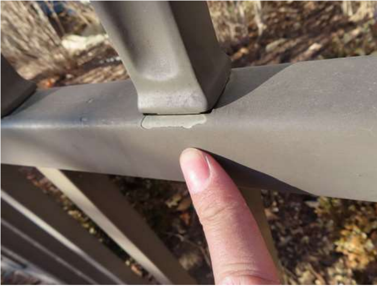
405. Building 18. Chip from thermal strains.
