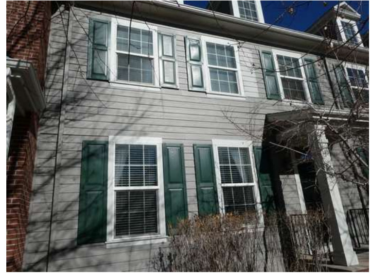
442. Building 20. Paint finishes on fiber cement siding were not chipped by hail.
