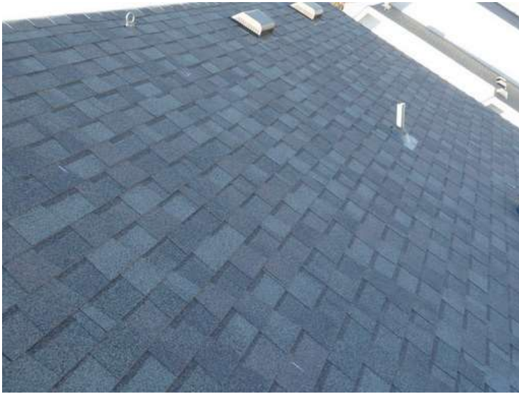
529. Building 22. North test area. No shingles within the test area were bruised by hail.
