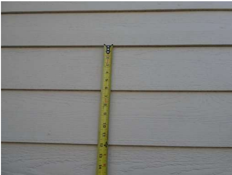
479. Building 21. Paint finish on fiber cement siding was not fractured by hail.
