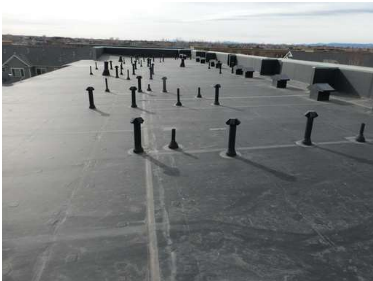
319. Building 14. View looking south. The roof was covered with an adhered EPDM membrane.
