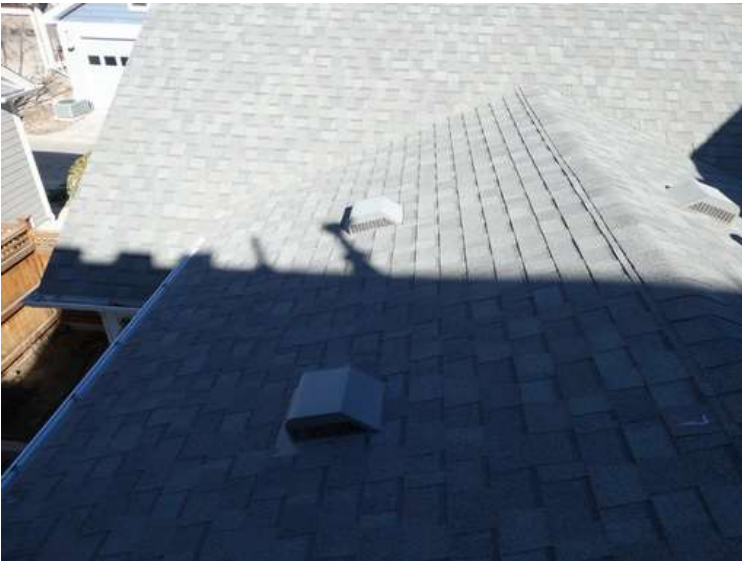
491. Building 21. West test area. No shingles within the test area were bruised by hail.
