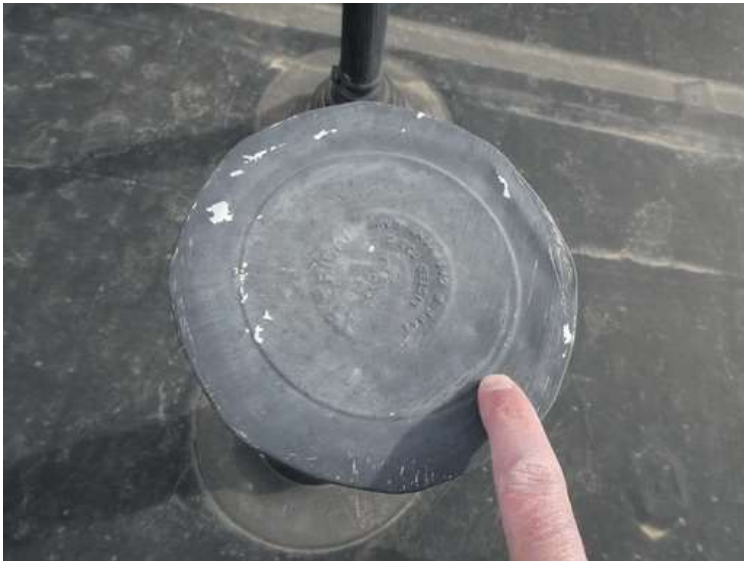
327. Building 14. Dents in a flue cap from hail.
