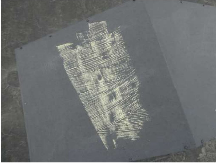
109. Building 04. Dents in an exhaust hood from hail.
