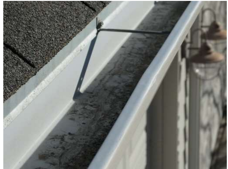
196. Building 08. Dent in a gutter.
