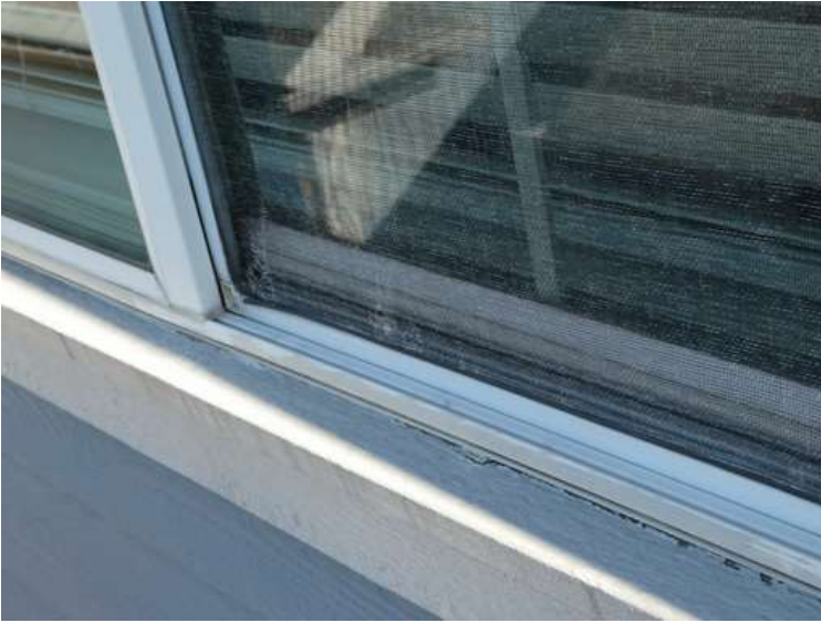
585. Building 24. Tears from hail.
