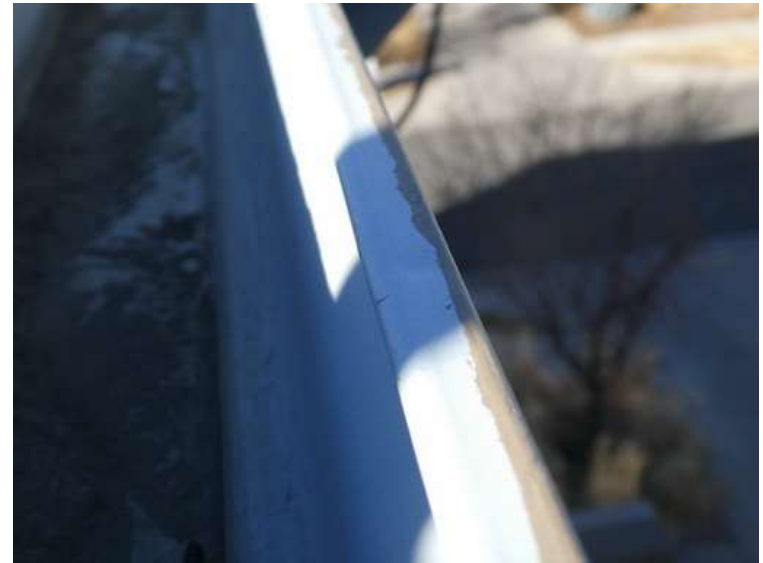
640. Building 26. Dent in a gutter.
