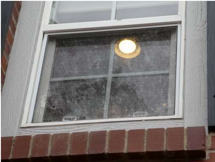
145. Building 06. Tears in a screen from hail.
