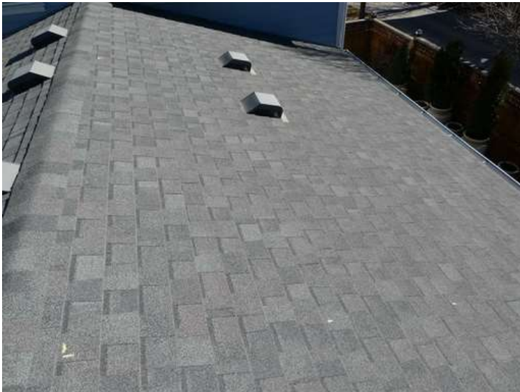
595. Building 24. South test area. No shingles within the test area were bruised by hail.
