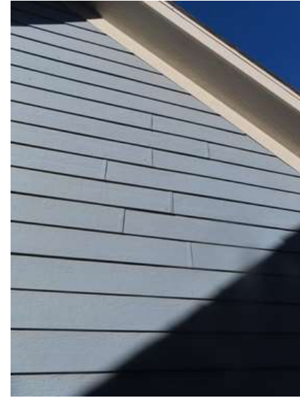
266. Building 11. Paint was not chipped from fiber cement siding.
