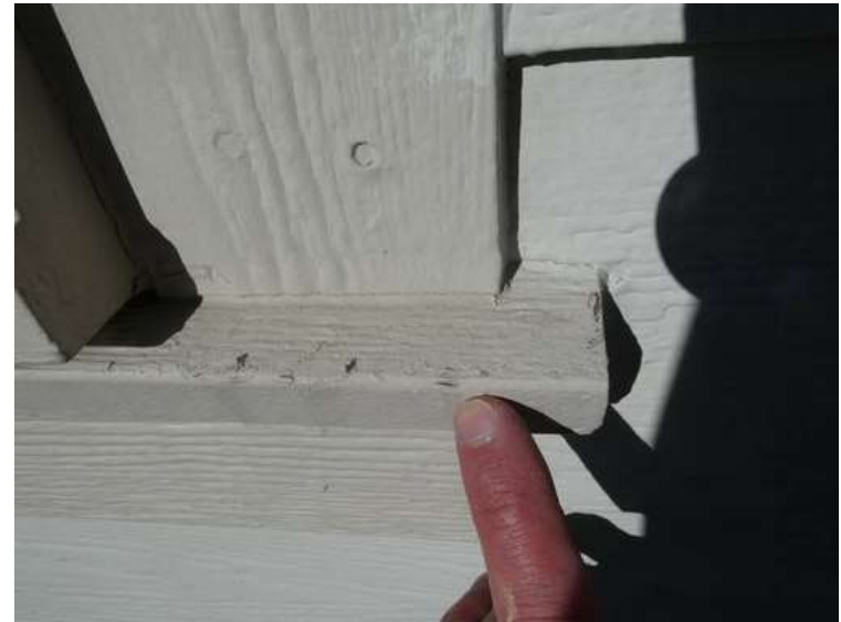
258. Building 10. Paint chips on a sill.
