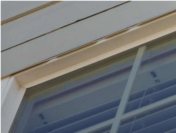
477. Building 21. Fractures in another vinyl window frame.
