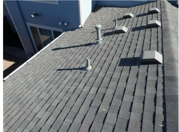
594. Building 24. North test area. No shingles within the test area were bruised by hail.
