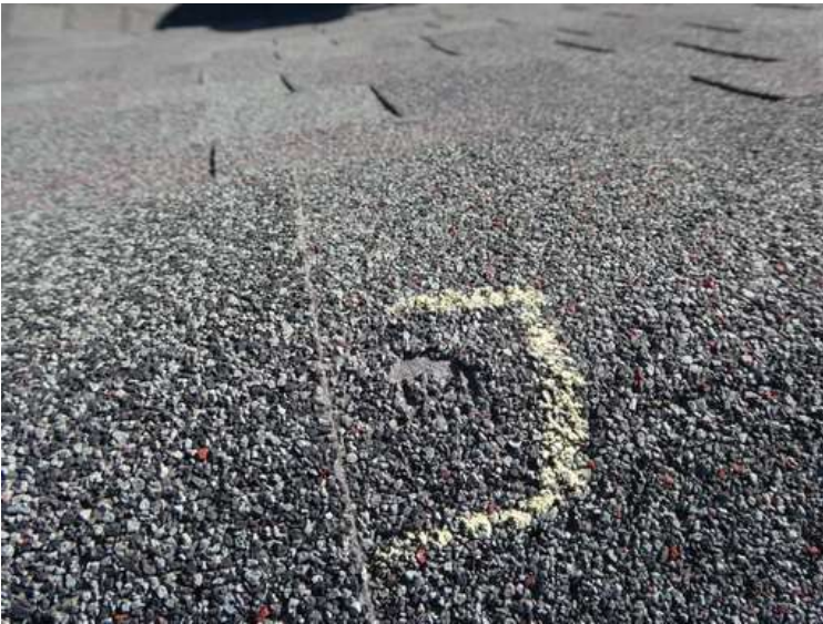
555. Building 23. Bruise in a ridge shingle from hail.
