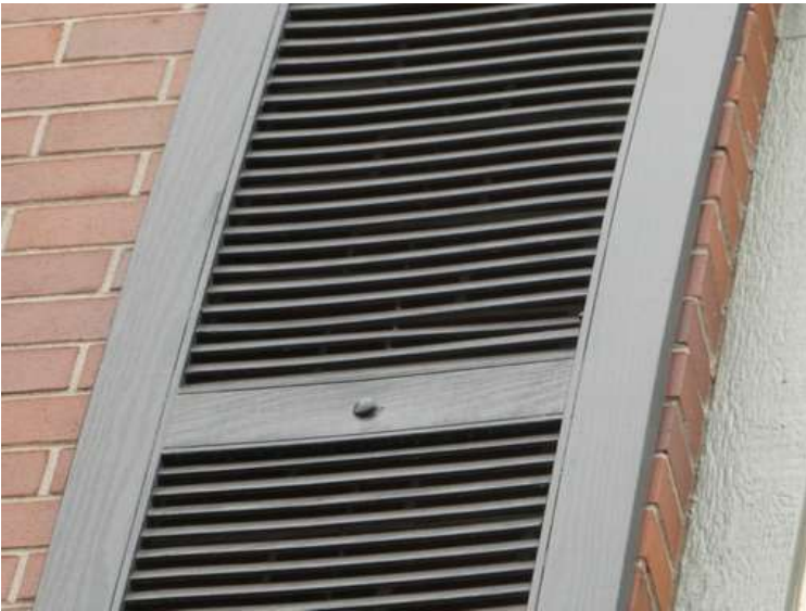
35. Building 02. Fracture in a shutter.
