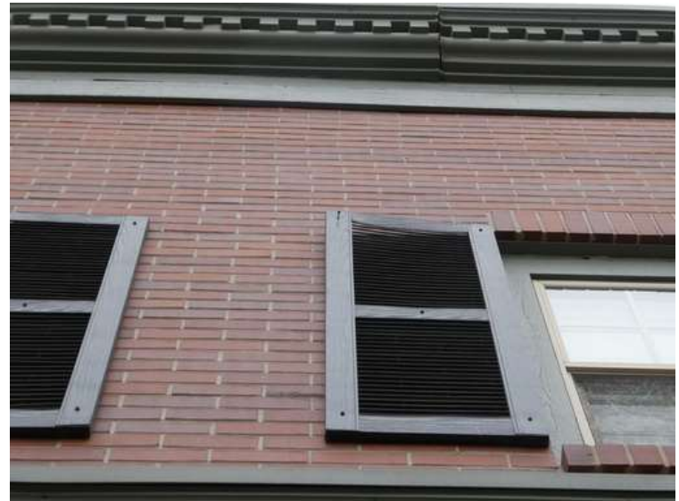
96. Building 04. Warped shutter.
