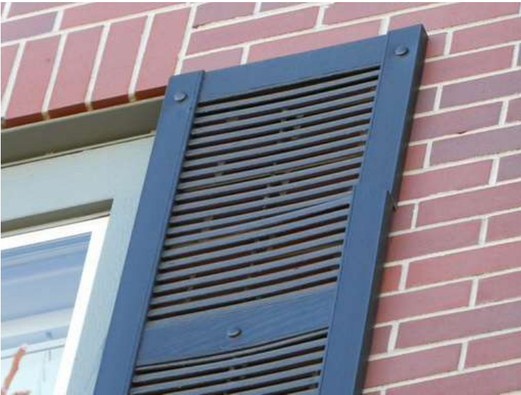
611. Building 25. Fractured shutter.
