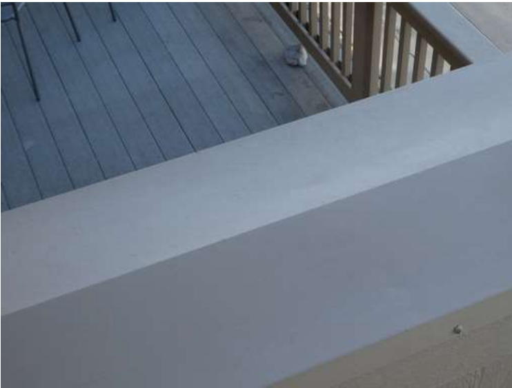
639. Building 26. Dents in a steel cap from hail.
