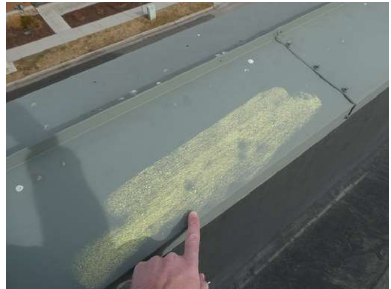
356. Building 15. Dents in coping from hail.
