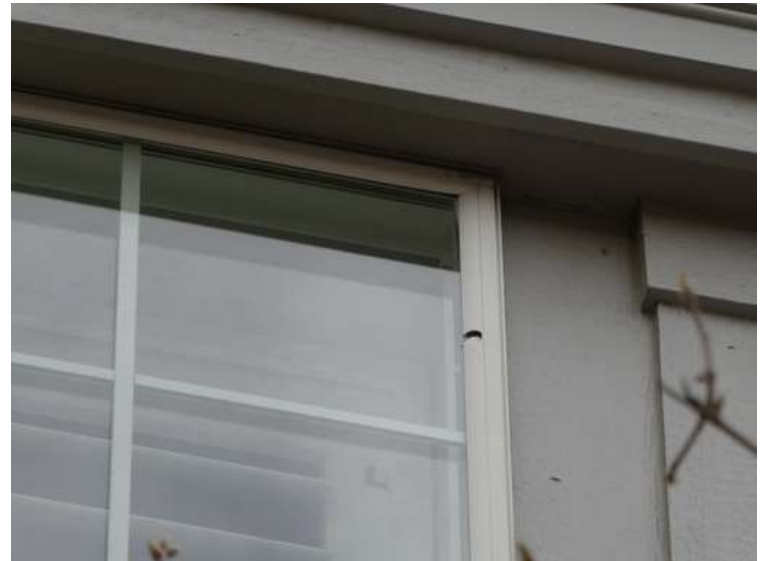
124. Building 05. Fracture in vinyl glazing bead.
