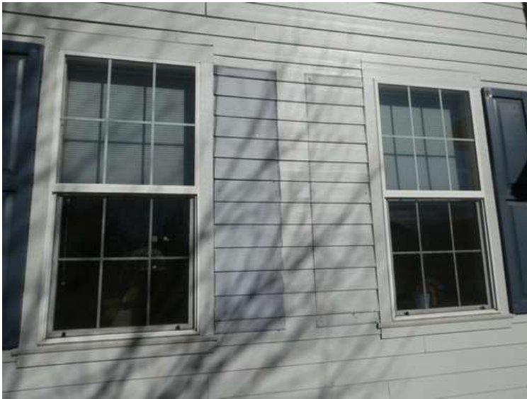
471. Building 21. Windows missing shutters.
