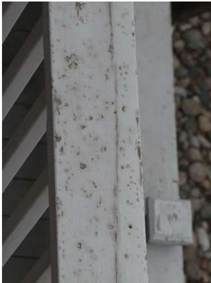
163. Building 06. Chips in paint on a hand railing from hail.
