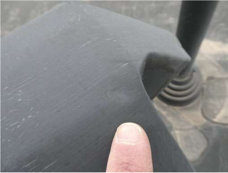
21. Building 01. Dent in a flue cap from hail.
