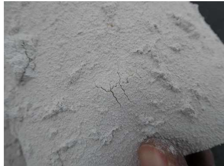
160. Building 06. Tear in the facer sheet adhered to the EPDM membrane from hail.
