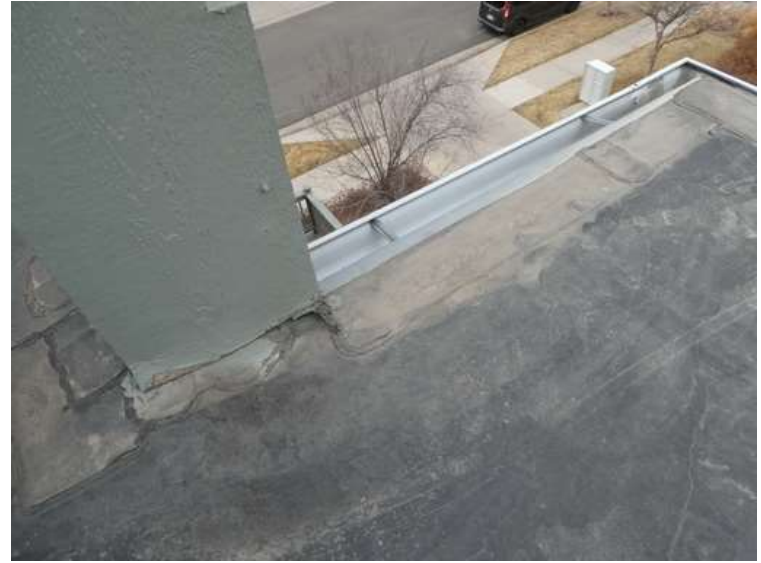
90. Building 03. Membrane tied into a parapet above Unit 2955. The deck was soft.
