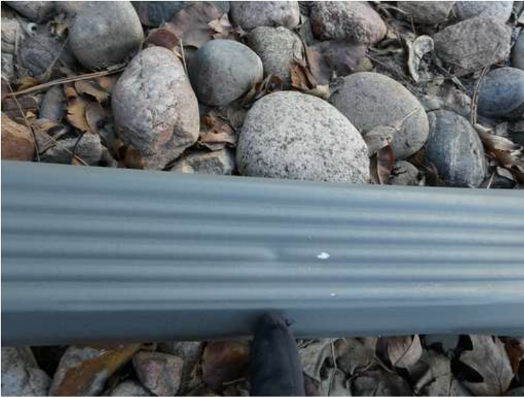
609. Building 25. Dent in a downspout extension from hail.
