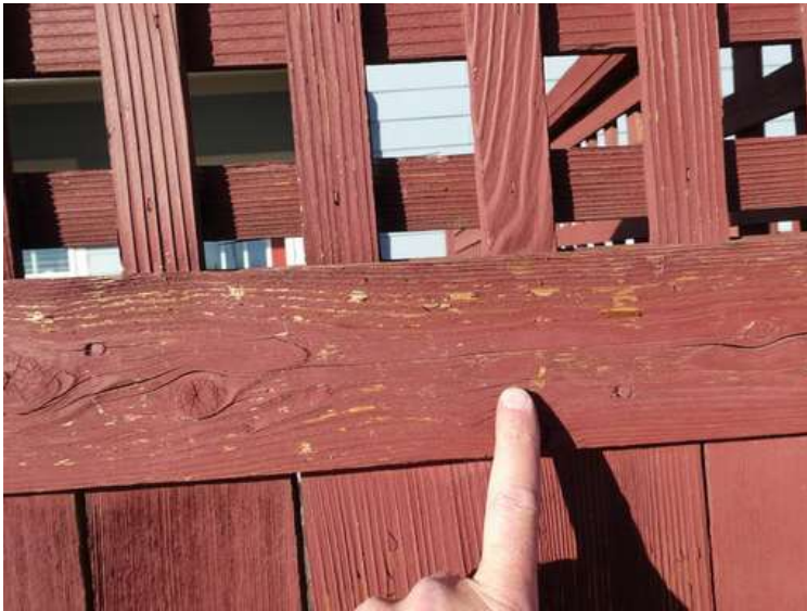
171. Building 07. Scuffs in stain from hail.
