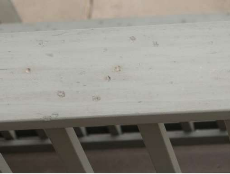
385. Building 16. Chips in paint finish on a hand railing from hail.
