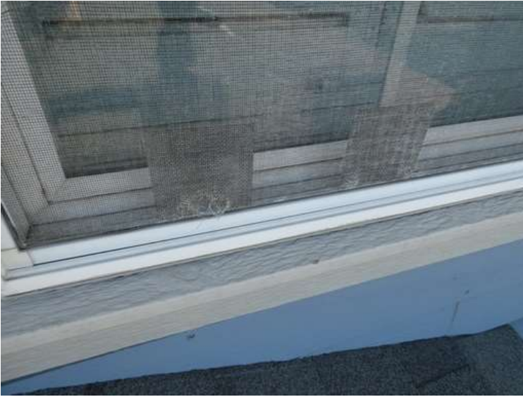
221. Building 09. Tears in a screen.
