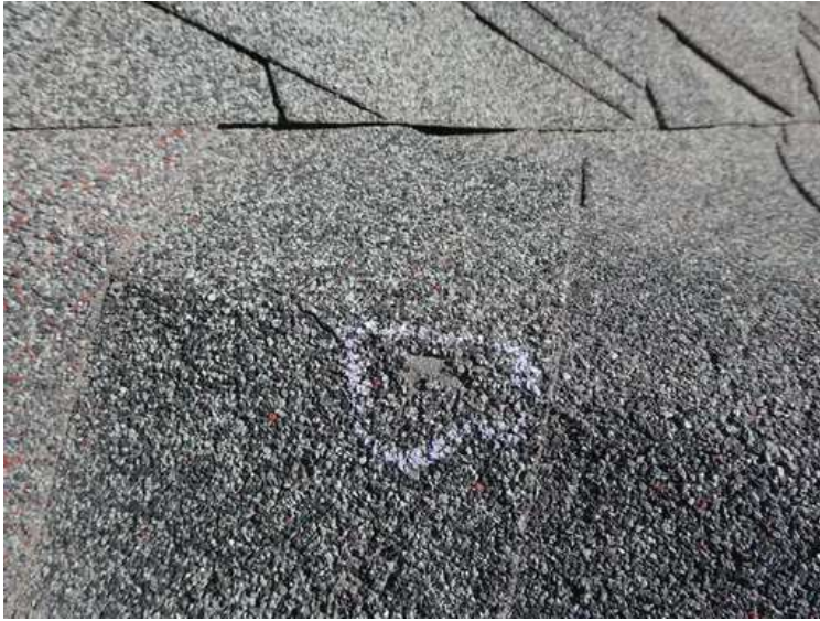
501. Building 21. Bruise in a ridge shingle.
