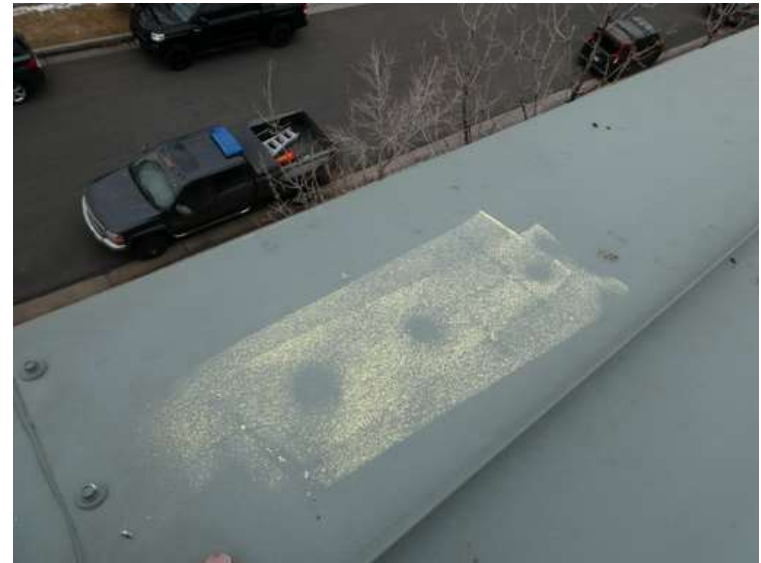
76. Building 03. Dents in coping from hail.
