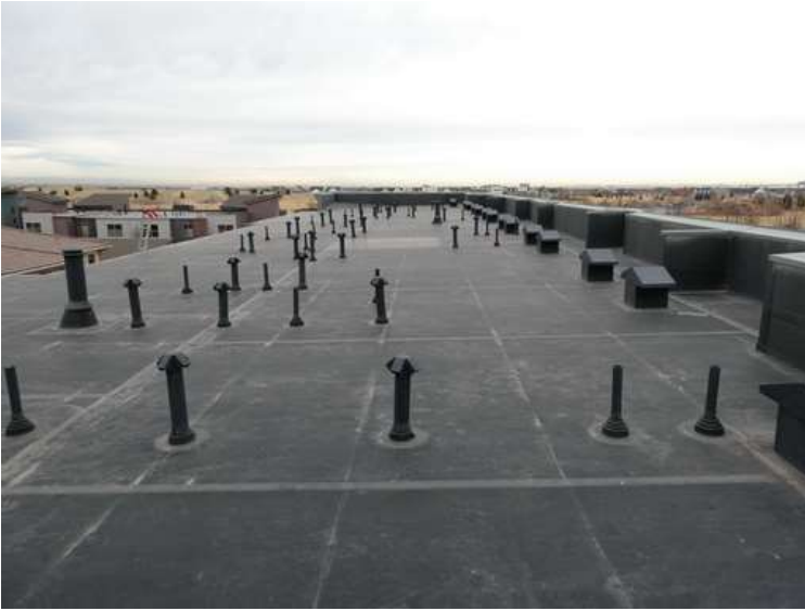
73. Building 03. View looking north. The roof was covered with an adhered EPDM membrane.
