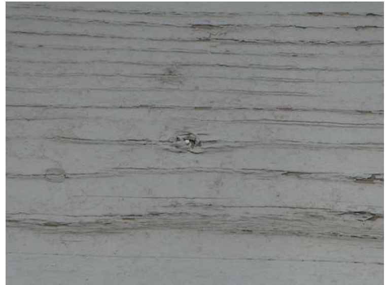
136. Building 05. Chips in paint on a railing from hail.
