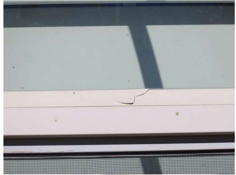
262. Building 11. Fracture in glazing bead from hail.
