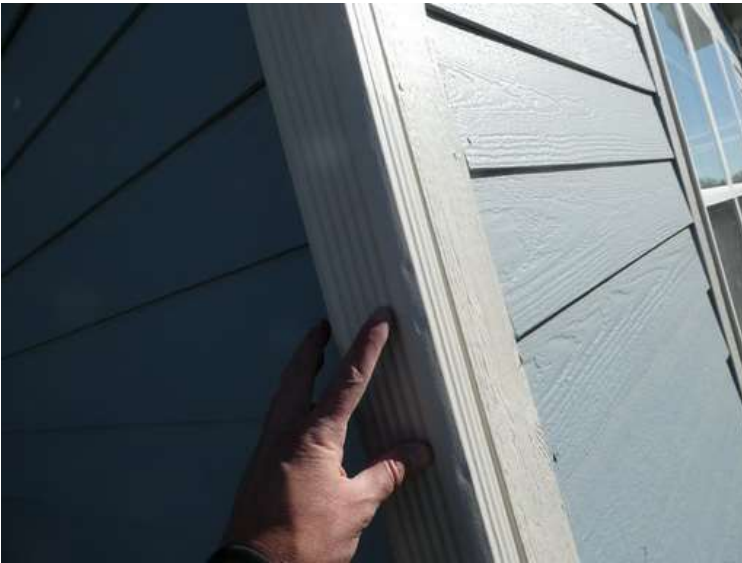
223. Building 09. Dents in a downspout.
