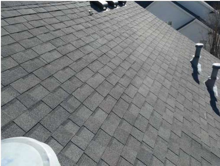
599. Building 24. West test area. No shingles within the test area were bruised by hail.
