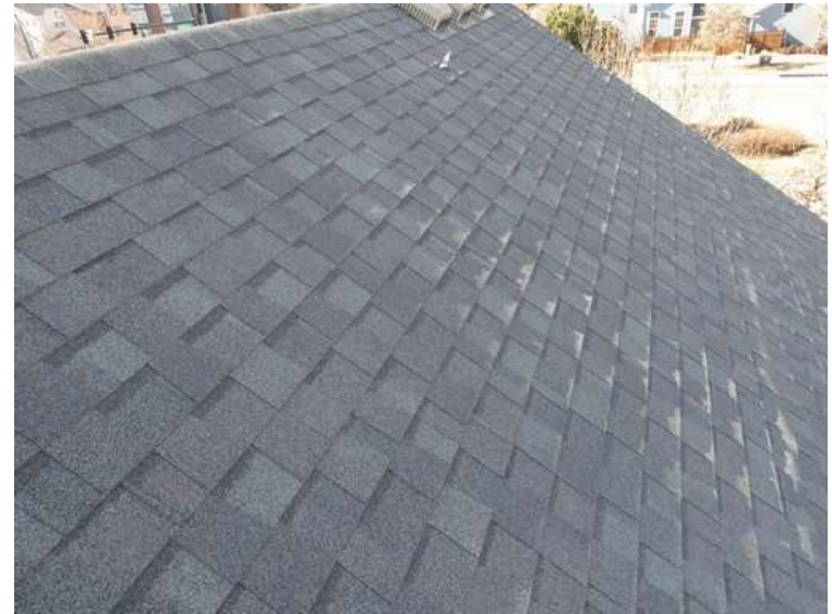
468. Building 20. North test area. No shingles within the test area were bruised by hail.
