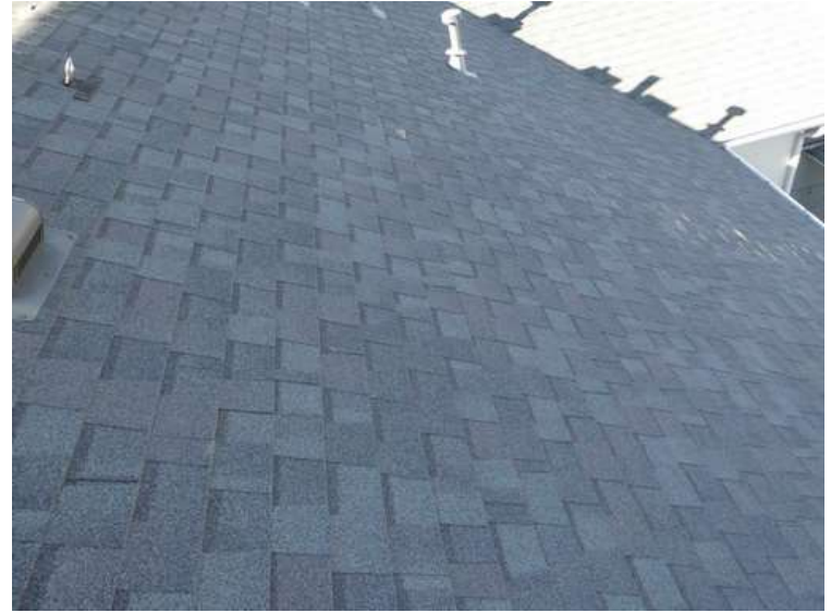
502. Building 21. North test area. No shingles within the test area were bruised by hail.
