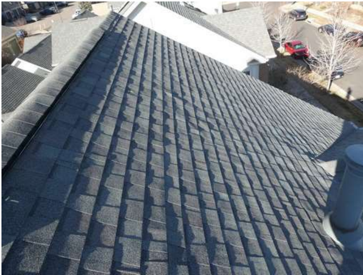
235. Building 09. East test area. No shingles within the test area were bruised by hail.
