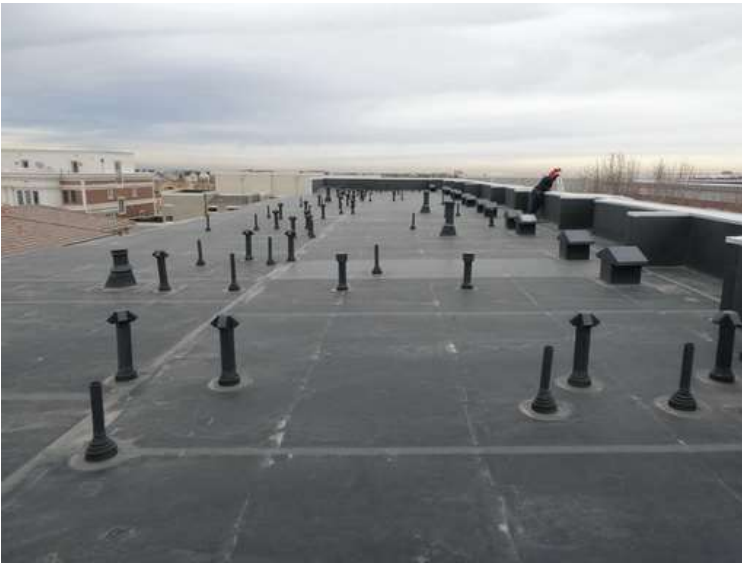
125. Building 05. View looking north. The roof was covered with an adhered EPDM membrane.
