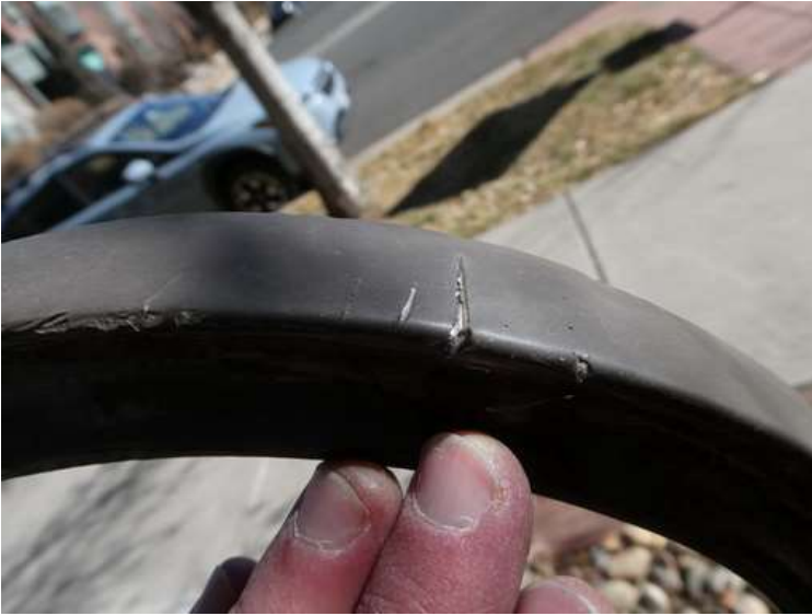
573. Building 24. Mechanical scuffs.
