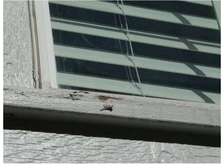
582. Building 24. Chip in paint from hail.
