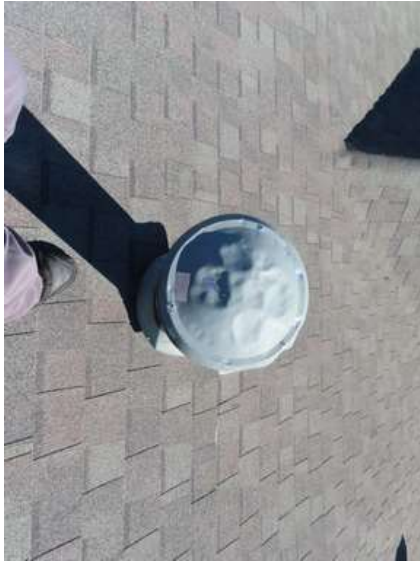
429. Building 19. Dents from hail.
