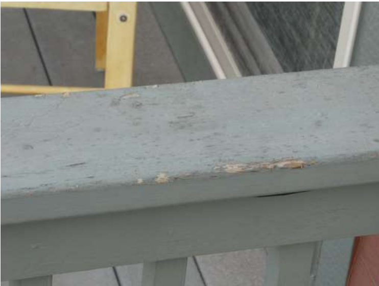
347. Building 15. Fractures in paint finishes on railings from hail.
