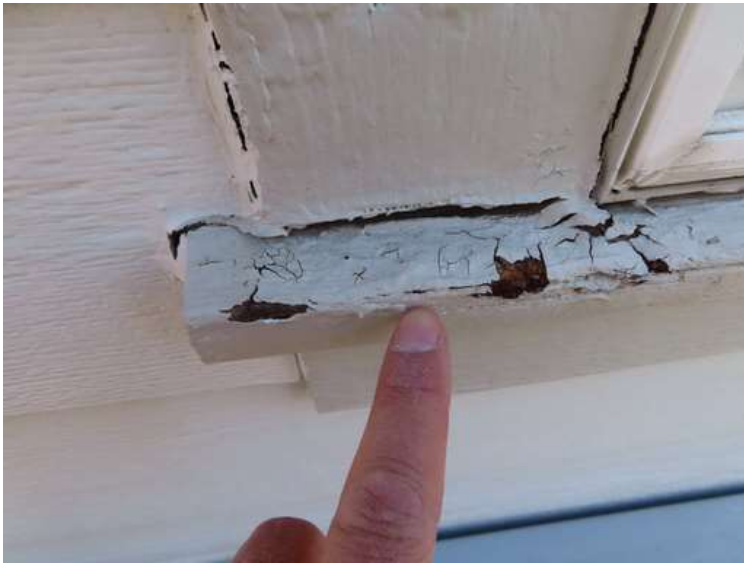
281. Building 12. Chips in paint on a rotted sill.
