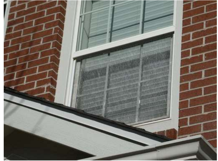
470. Building 21. Tears in a screen from hail.
