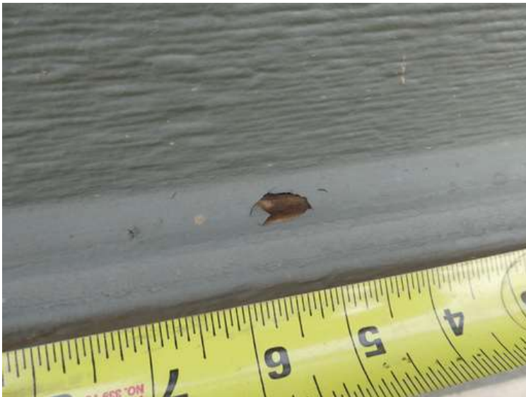
375. Building 16. Chip in paint from hail.
