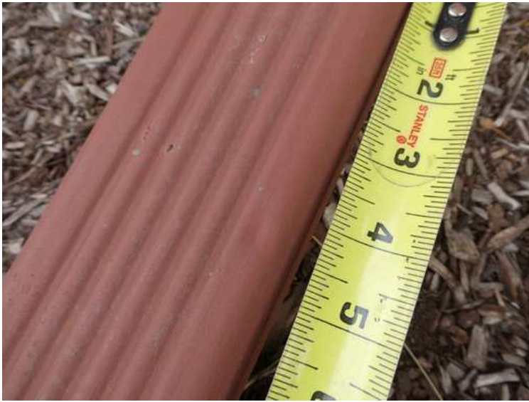
309. Building 14. Dent in a downspout extension from hail.
