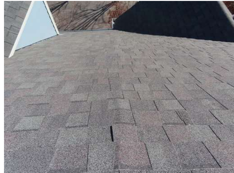
432. Building 19. Wrinkle from decking movement.
