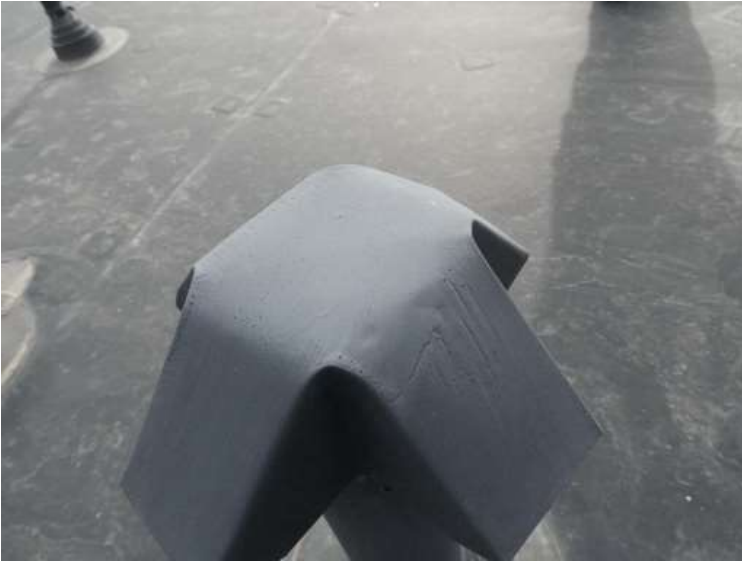
357. Building 15. Dent in a flue cap from hail.
