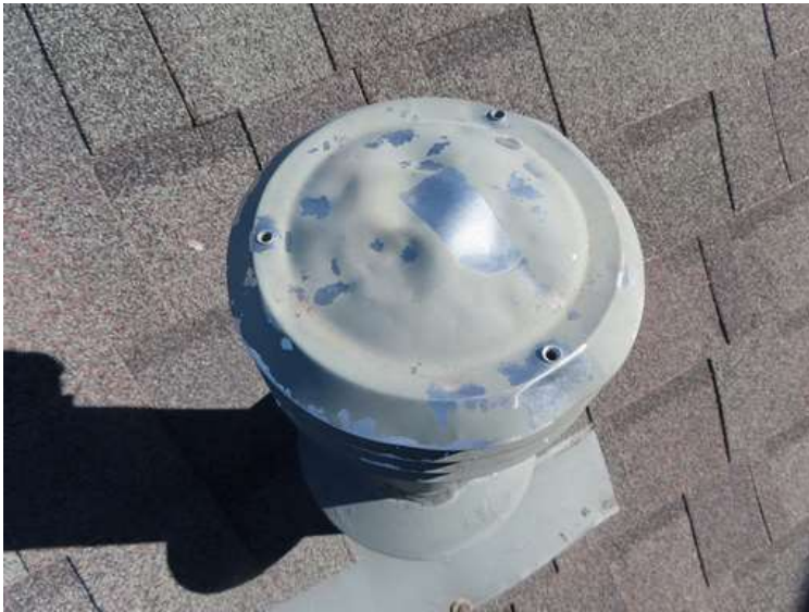
297. Building 13. Dents from hail.
