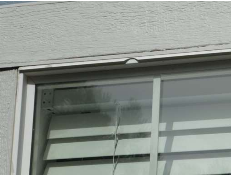
575. Building 24. Fracture in a vinyl window frame from hail.
