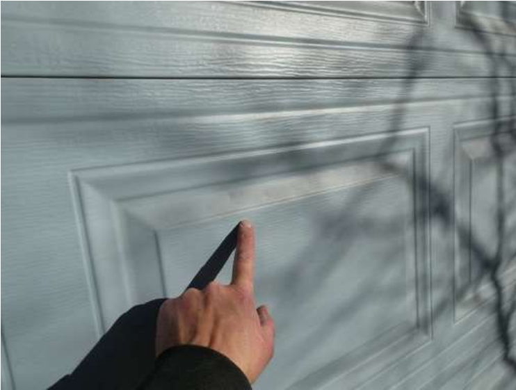
173. Building 07. Dents in a garage door from hail.
