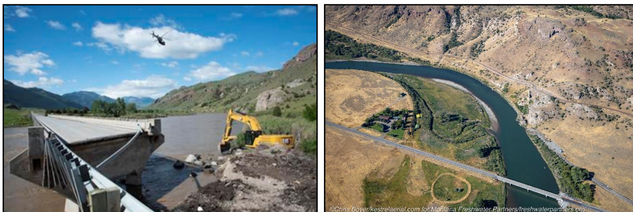
Figure 30 Point of Rocks Bridge after 2022 flood (left), and after the emergency repair (right). Photo on the right is by Chris Boyer.
