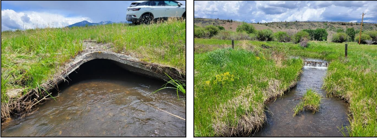
Figure 35 Fridley Creek culvert inlet (left) and beaver dam against a fence upstream of culvert (right).
