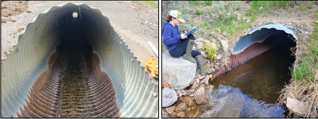
Figure 26 Bassett Creek culvert inlet (left) showing steep portion of culvert with shallow, fast flows; and outlet (right) showing the lower gradient portion of the culvert with deep, slow flows.
