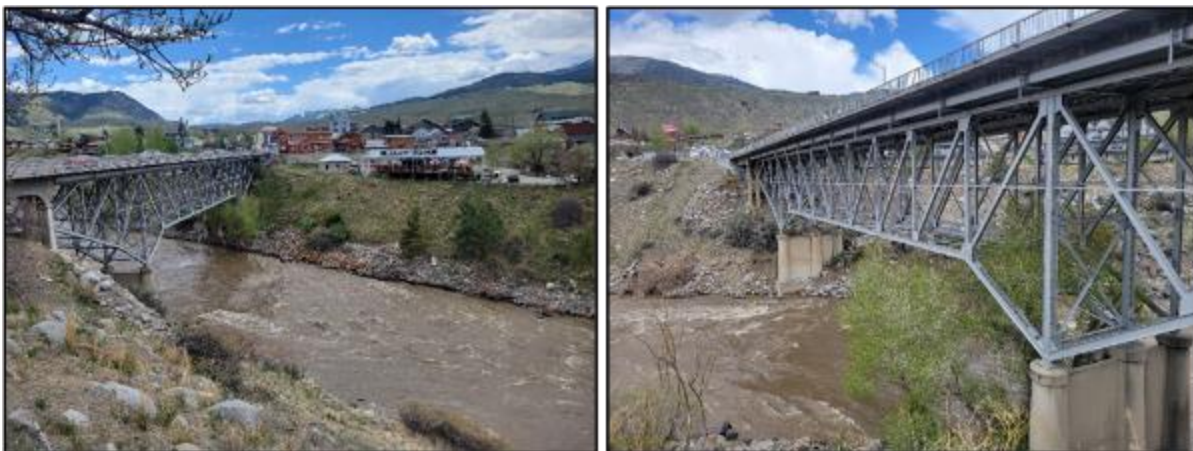
Figure 24 Gardiner bridge from river left looking towards river right (left) and from river right looking towards river left (right).
