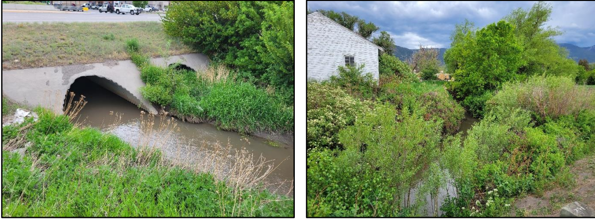
Figure 38 Billman Creek culvert outlet (left) and Billman Creek upstream of US 89 crossing showing incision.
