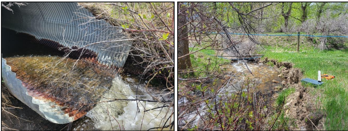
Figure 25 Little Trail Creek outlet structure (left) and looking downstream from outlet structure (right).
