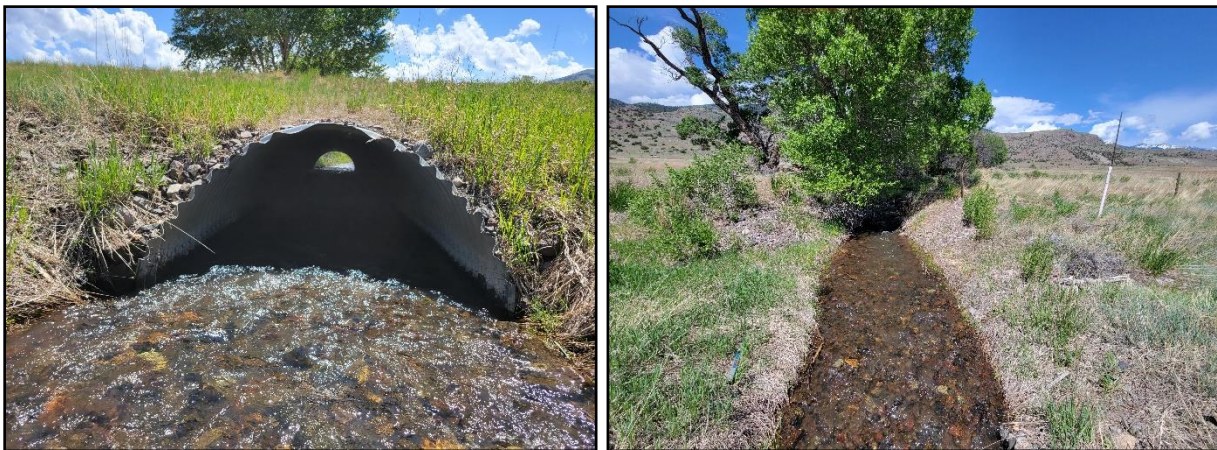
Figure 31 Donahue Creek culvert outlet (left) and Donahue Creek downstream of culvert (right).
