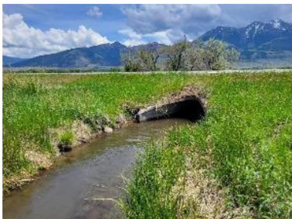
Figure 34 Ditch that captures water from Goldmeyer Creek where it flows under US 89.
