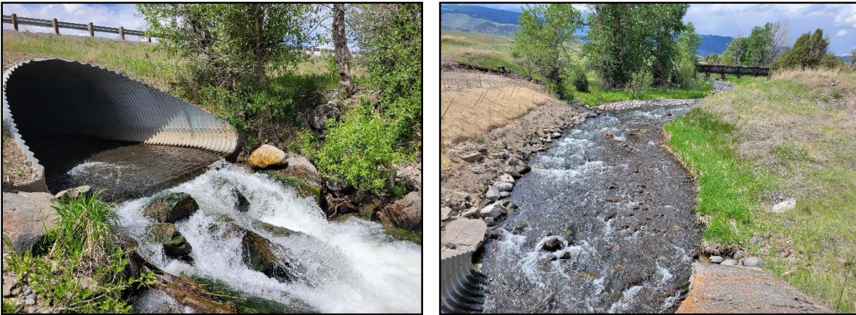
Figure 36 Eightmile Creek culvert outlet (left) and Eightmile Creek upstream of US 89 crossing (right).
