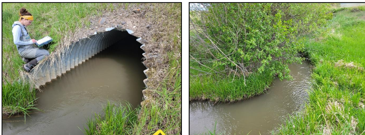
Figure 37 Trail Creek/ Ditch crossing under US 89 (left) and ditch upstream of culvert (right).
