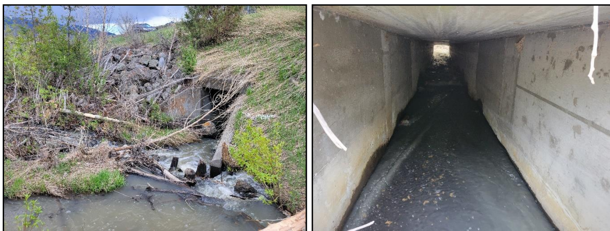
Figure 28 Slip and Slide Creek culvert inlet (left) showing extensive beaver activity and erosion around the culvert wingwall on river right. The image on the right is through the culvert from upstream to downstream, showing the slope break midway through.
