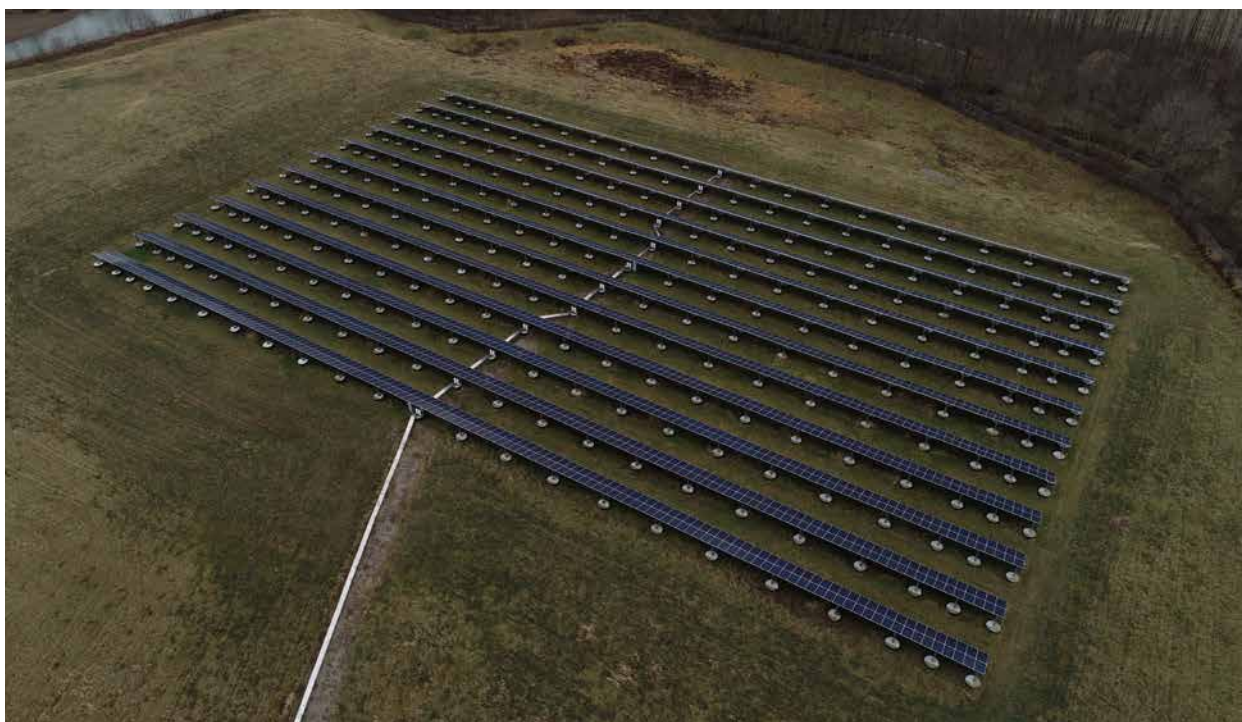
In Newark, Ohio a 6,000-panel solar project provides 25% of the energy needed for the city's wastewater treatment plant. The solar array was constructed on a vacant brownfield that the city was not utilizing.
