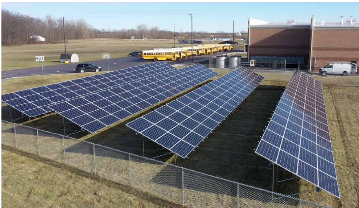
A student-led initiative brought solar energy to Graham Local Schools in Champaign County, Ohio. The solar arrays are able to produce approximately 136,000 kilowatts of energy per year, which measures to be about 78% of the school district's energy usage. Photo: The Nature Conservancy
