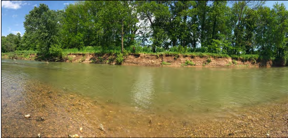
Illinois River 2 FID 75, (2019) Critical Bank View.
