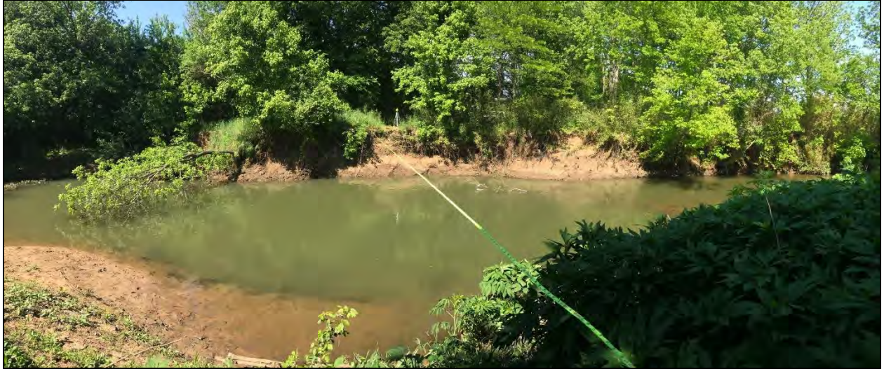
Muddy Fork 1 FID 172 (2019) Critical Bank View
