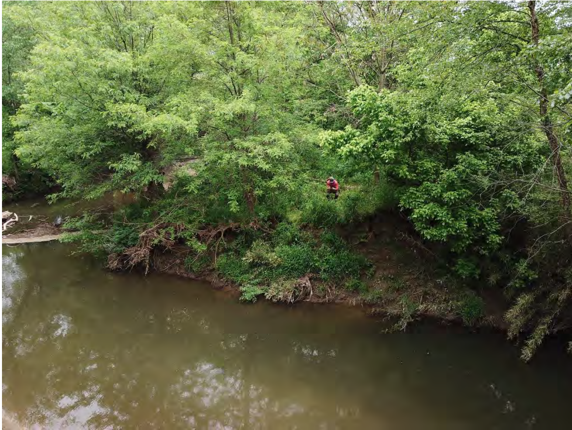
Moore's Creek 3 FID 43 (2019) Cross Section View looking back at the very stable study bank.
