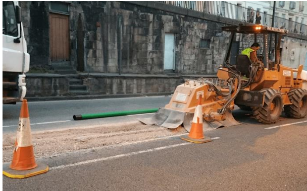
It is possible to cut one tram-track at a time for minimal traffic disrupting and no diversion of services. Photo: pipe-laying in Bath
