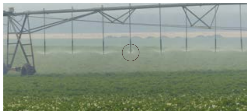
Figure 4. A faulty sprinkler head; for this crop, which was grown during hot weather, reduced irrigation limited growth and caused an estimated 10% drop in yield.
