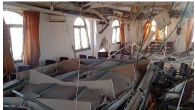
Bomb damage to Gaza Baptist Church Dec. 26, 2023 Credit: Word & Way. More in article by Brian Kaylor.
