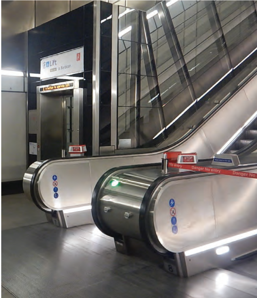
Accessible route on the Elizabeth Line at Barbican Station where the lift tracks the escalator. Photo: Jos Boys.
