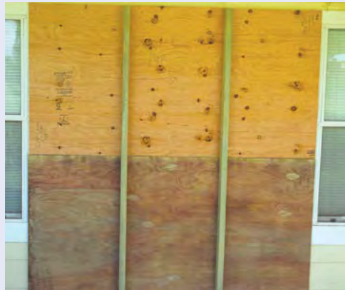
Figure 4-54. For larger windows, such as this sliding glass door, two 2 by 4's face outside and are oriented with the narrow end against the plywood . The fastening screws attach from the plywood into the 2 by 4 (see Figure 4-55).
