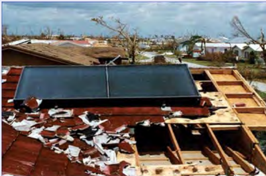
Figure 4-71. House with solar panels hit by hurricane winds. Note the major damage along the rakes of the roof. As noted in Figures 4-58 to 4-60, pressure is greatest along the edges and can lead to loss of shingles and eventually the roof decking (plywood sheathing). Thus the best practices shown in Figures 4-61 to 4-64. The solar panels remained on the roof, held by the lag bolts attaching the panel system to the roof rafters or truss. Photo courtesy of One Block Off the Grid.
