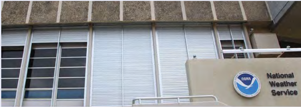
Figure 4-35. Roll-down shutters can provide significant protection against hurricane winds. The NOAA National Weather Service facility is protected with these shutters; here, the shutters are fully deployed over the two middle windows, and partially deployed at the sides. The shutters are made from heavy duty aluminum slats.
