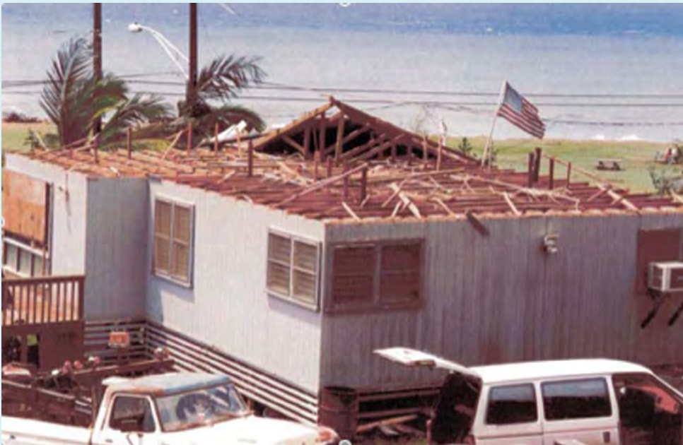
Figure 2-5. A common site on Kauai after Hurricane Iniki. Many roofs were blown off due to a lack of proper connection. Photo courtesy of Department of Commerce and Consumer Affairs Insurance Division.
