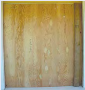
Figure 4-53. If the joint between the plywood is short, for example, 4' to 5' in length, a 2 by 4 (really 1 ½" by 3 ½") can be used with the wide end on the outside against the plywood . Both ends of the 2 by 4 are then attached with screws through the plywood and into the window frame. This will require two 4 or 4 ½" lag screws, which may require pre-drilling or similar Simpson Strong-Tie self driving screws (SDS).
