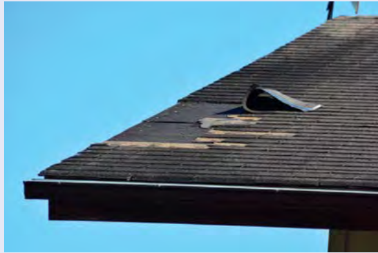
Figure 4-60. At less than hurricane strength winds, Iselle initiated the peeling off of asphalt shingles along the rakes (edge) of this roof, as expected (see Figure 4-58). This problem would have been much worse with a hurricane, as forces on building structures do not double with the doubling of wind speed but quadruple. Progressive failure with wind speed increase could include peeling off all the shingles, then the sheathing and then the entire roof.
