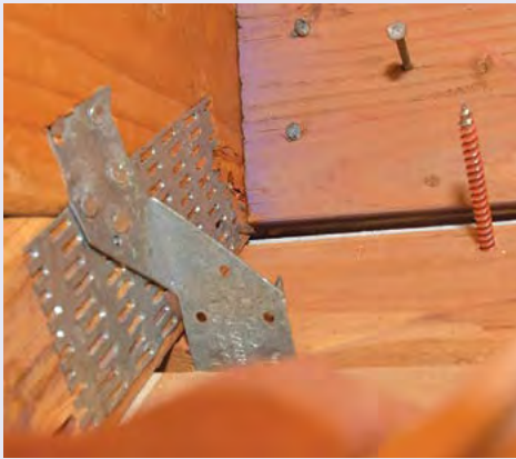
Figure 4-21. For this double-wall house, the H2.5 hurricane clip (see Figure 4-2), ties the truss to the double-top plate. Ideally, 5 nails should be in the top tab and 5 on the bottom. This clip was installed in 1992 as a building code requirement at the time of construction from the interior of the house before any walls were installed. To the right is the orange SDWC, drilled from the outside of the house through the siding in 2018. It purposely missed the truss for illustration purposes. Moving the screw to the left by 6 inches would serve the same function as the H2.5 and tie the double-top plate and truss. Thus, it is possible to install the SDWC even if there are existing hurricane ties such as the H2.5. This can serve to strengthen the connection when there are no hurricane clips, clips that are poorly installed, or even clips that are properly installed but of less capacity.
