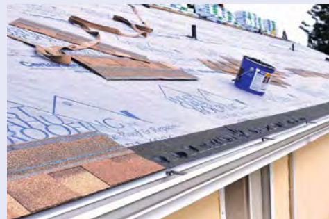
Figure 4-64. To address the increased wind pressure on the corners and edges of the roof from hurricane winds (see Figures 4-58 to 4-60), one inch dabs of asphalt roof cement are placed between the starter shingles (black) and first course of roof shingles (brown) for the eaves. With this technique, the especially vulnerable corners and edges of the house are protected with shingles that are attached with six nails and nine dabs of asphalt roof cement. For exact placement of the shingles and cement for the eaves, rakes, hips, or ridges of the roof, see Technical Fact Sheet 7.3. This method takes time, but is stronger at the vulnerable parts of the house (see Figures 4-58 to 4-60).
