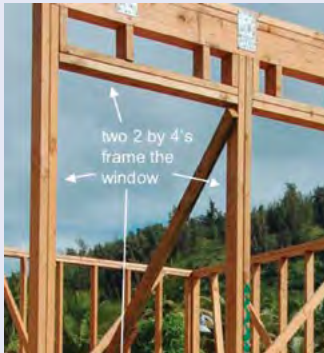
Figure 4-47. For this double-wall house under construction, two 2 by 4's frame the window. When attaching the plywood to the window, the fasteners should go into the 2 by 4's, not the siding. It is always useful to know how your house was built. Take pictures during construction (if possible), review your blueprints, drill small test holes if you have to, or ask your architect or home builder for the details on your window.
