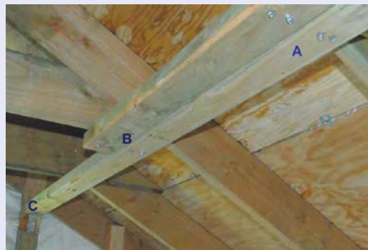
Figure 4-68. In this application of lateral bracing, the 2 by 4's are 18 inches from the ridge and connect to horizontal members that attach the opposing trusses. Not all roofs will have the horizontal members. The 2 by 4's are connected with two #14 3-inch screws (A) and overlap over two trusses (A and B). The end is connected to the gable end with an angle or L bracket (C).
