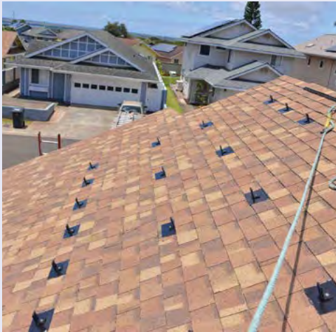
Figure 4-73. Fasteners used to attach the racking system and solar panels are shown. The fasteners represent parts A, B, and C of Figure 4-72. Where it was necessary to go near the rakes or edge of the roof, or the corner near the ridge, extra fasteners were provided, a change from every 4', or every other rafter, to every 2' but only for the areas near the higher wind roof zones. Extra fasteners were $85 each. Federal and state tax credits pay for a portion of the increased cost. Check with a contractor whether extra fasteners are needed given the wind loads on the installed panels for the area and the uplift resistance per-fastener (Endnote 35). Another alternative to extra fasteners are wider and/or longer lag bolts into the roof rafters.
