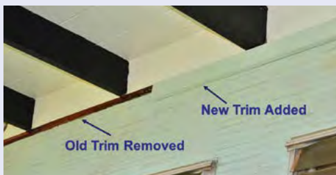
Figure 4-11. The old trim has been pulled. The new trim is 1 inch x 4 inch exterior wood, treated for termites, painted with primer and two coats of paint that color match the wall. Color matching can be done by taking a small sample to your local hardware store.
