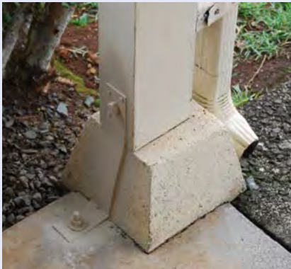
Figure 4-6. In some retrofit examples, it is possible to tie a portion of the house to the foundation. Here, a metal strap connects the vertical post to the foundation, which attempts to finish the continuous load path connection from the roof to the foundation. Photo courtesy of Hurricane Protection Services.
