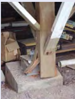
Figure 4-15. Damage after the October 15, 2006 Kiholo Bay Earthquake (see Figure 2-10). This post was shaken off the termite pan and tofu block (Reference Link 43). While the major emphasis for an earthquake is horizontal or lateral loads from shaking of the ground, often a retrofit for lateral loads, such as anchorage of the foundation posts will also be effective in resisting lateral and vertical loads caused by hurricane strength winds. Once anchorage to the foundation posts is performed, the weight of the house itself will provide some vertical uplift protection. The key is to keep the foundation posts properly anchored.
