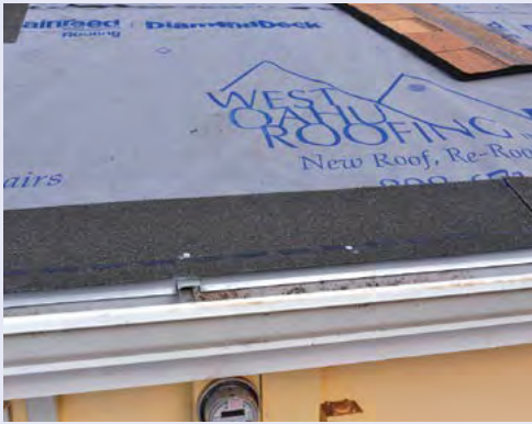
Figure 4-63. Roofing felt (grey) is then tacked onto the self-adhering modified bitumen layer. The FEMA guideline calls for the #15 felt, which is supposedly cheaper. In this instance, the #30 felt is stronger and about the same price (considering more expensive materials, but cheaper installation cost). Check with a licensed contractor. The purpose of the felt is to prevent the bonding of the overlying asphalt shingles with the underlying bitumen layer. If there is bonding, it would be difficult to remove the shingles at the end of their useful life. Bonding problems in the past have required complete removal of the plywood to remove the asphalt shingles.
