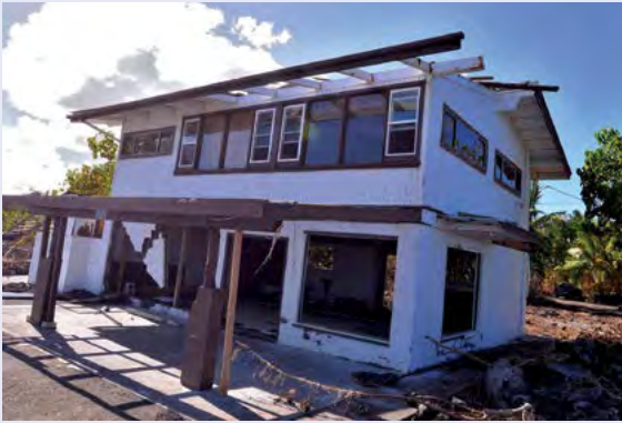
Figure 4-59. When Tropical Storm Iselle hit Hawai‘i County, this coastal house experienced wave inundation and roof damage. Although not an asphalt shingle roof, the damage was initiated at the corners, as expected, where uplift pressures were greatest (see Figure 4-58) even though the winds were less than hurricane strength. Better building practices could include fewer overhangs, overlap of roofing panels, and the use of ring shank nails.
