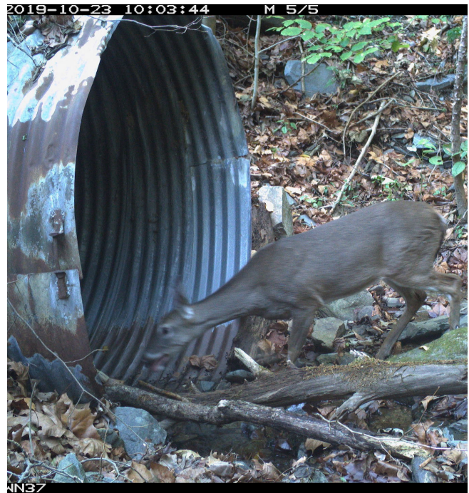
Although the culverts under I-40 were not designed with wildlife movement, some animals are already using them as safe routes to travel. Collecting this information is a key step in deciding where to add or enhance infrastructure to reduce collisions.
