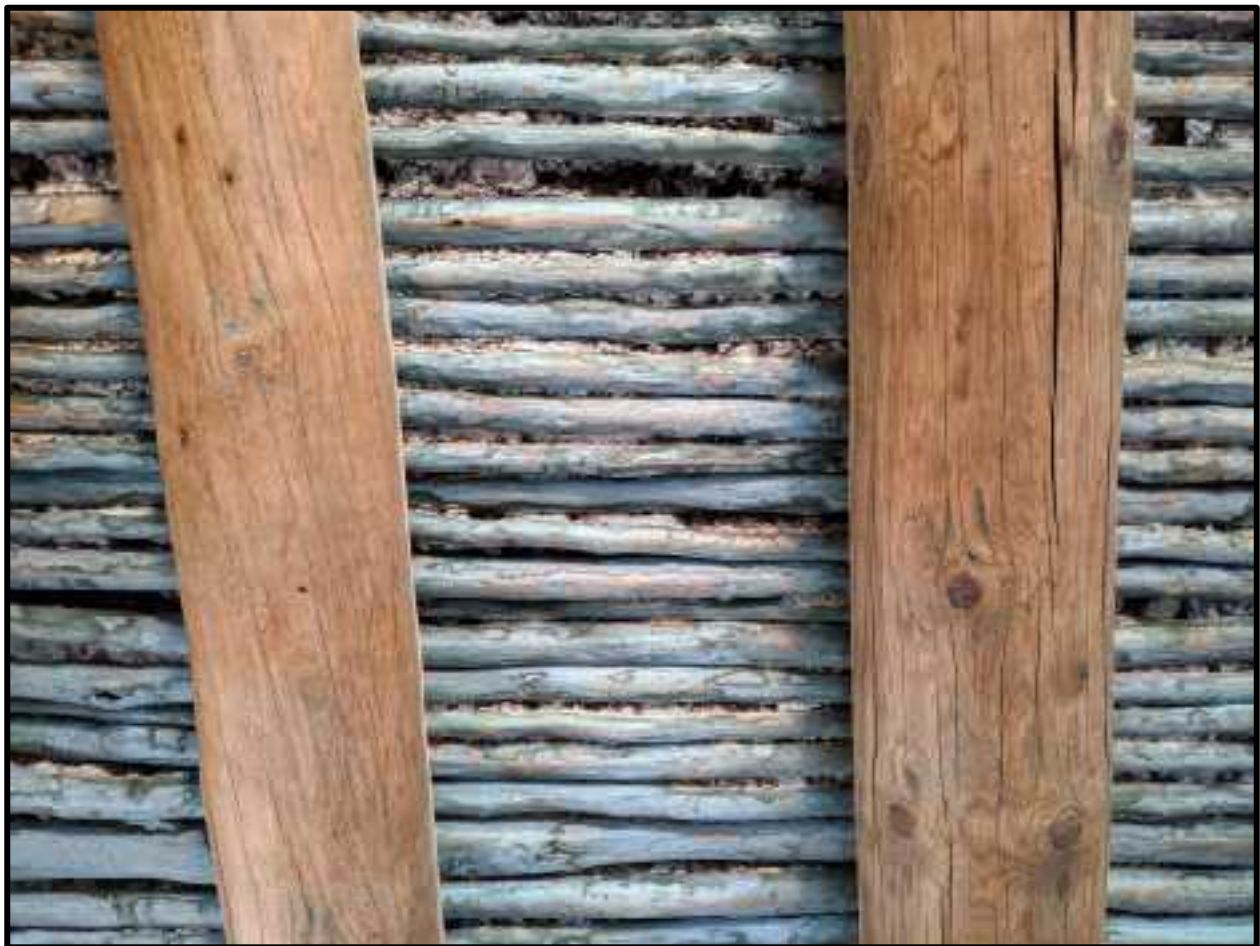
Vigas and latillas with mud roof in a house researched by Dr. Windes. These vigas are tree ring dated as having been cut 1824-1826. Latillas are “painted” with blue-tinted tierra blanca from La Cueva Blanca, south of Llano Quemado.
