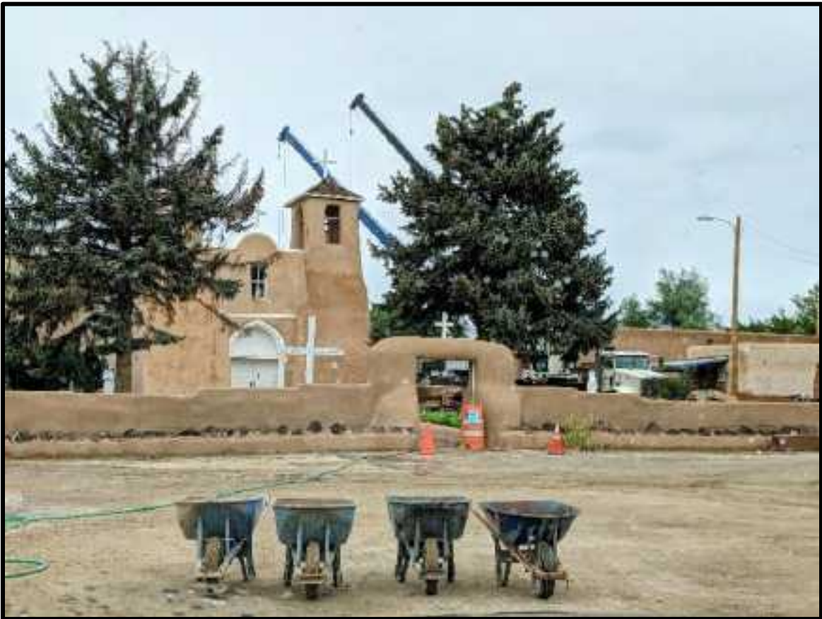
Replastering San Francisco de Asis, Ranchos de Taos Plaza, 1957-59? Replastering Lunch Break, 2021
