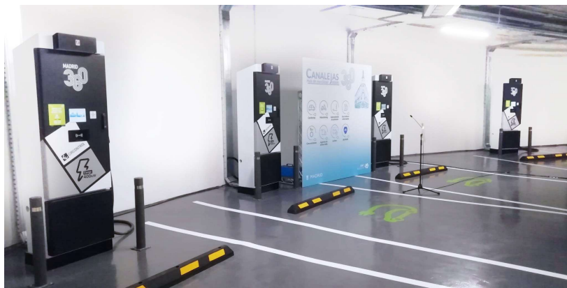
Figure 7 EV chargers at the hub "Canalejas 360"
