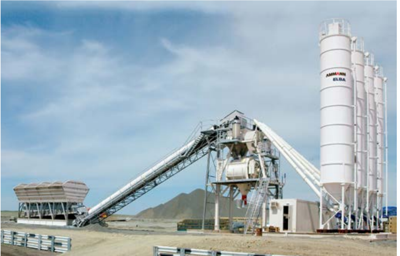
The CBS 180 TB Elba just before commissioning.
