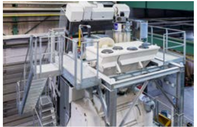
Good accessibility to the skip and weighing bin at the CBS 105 SL Elba
