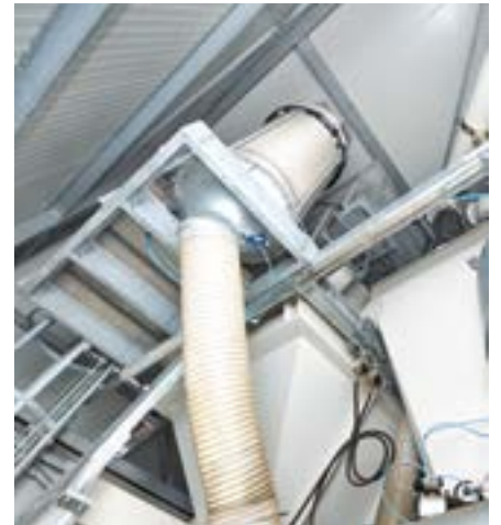
The central dedusting filter has a separate maintenance platform.
