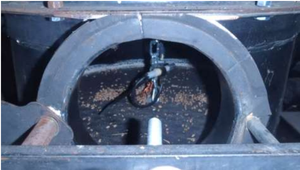
Figure 3-3. Plenum at bottom of bin.
