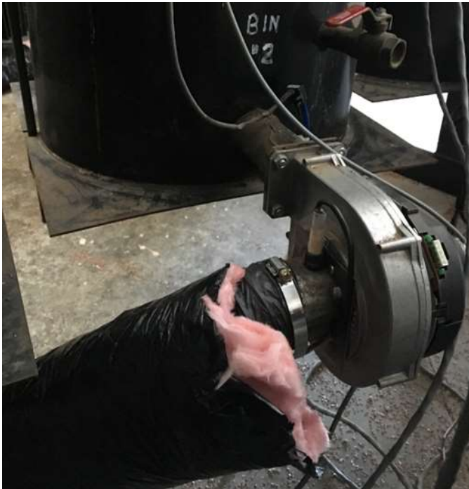
Figure 3-7. Insulated duct outlet connected to aeration fan inlet.
