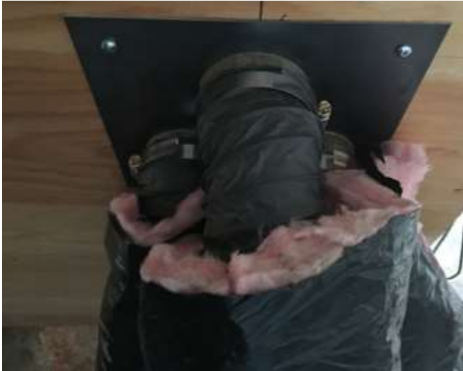
Figure 3-8. Insulated duct inlet connected to preheated chamber.
