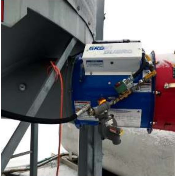
Figure 4-11. Downstream direct-fired heater.
