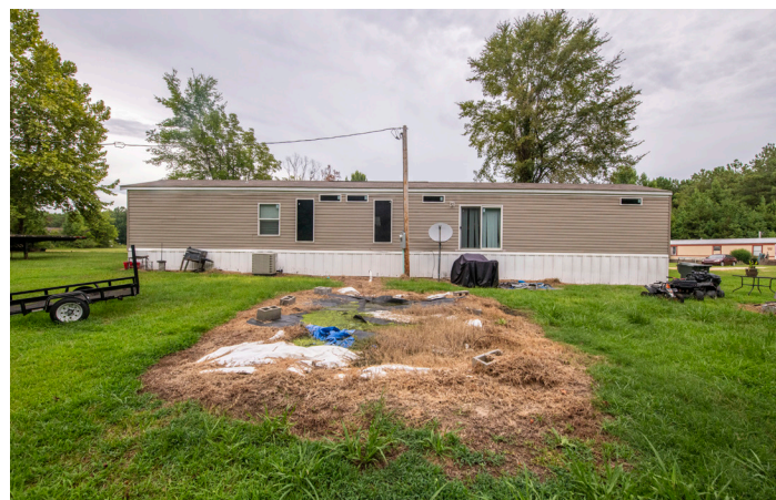
A home with a failing septic system resulting in a surface pool of sewage in Hayneville, Lowndes County, Alabama, on August 1, 2022.
