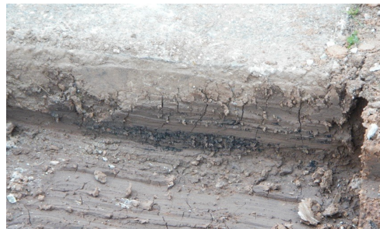
Potential Contamination Beneath Concrete in Parking Lot
