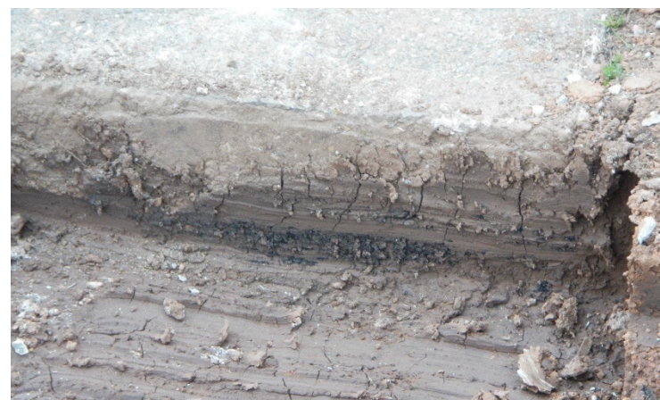
Potential Contamination Beneath Concrete in Parking Lot
