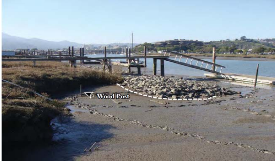
Figure 9. Photograph showing "outflanking", or erosion at the end of a marsh sill, which is typical of coastal structures over their design life (ESA 2017). The wood post shows the distance between the eroded marsh edge and landward side of the sill.
