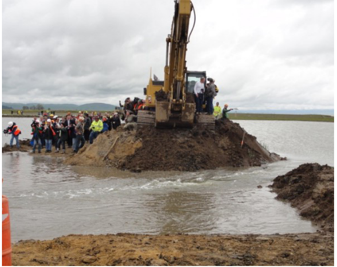
▲ Figure 32: Bayward levee was breached to restore site to full tidal action on April 25, 2014. Photo credit: USACE.
