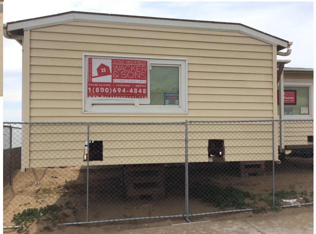
Building in process of being moved, Esplanade Ave, Pacifica, CA . Photos: Bob Battalio, May, 2016.
