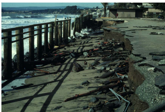
Figure 5. Failure of timber bulkhead at Seacliff State Beach due to wave and log impact.
