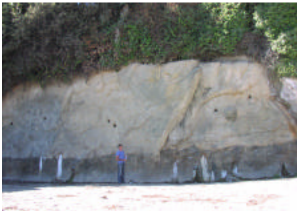
Figure 7. Cliff stabilization (soil nail wall) using concrete textured and colored to match existing cliff materials.
