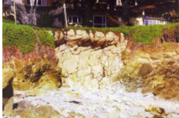
Figure 8. Soil nail wall in the Pebble Beach area designed to look like the adjacent granite.
