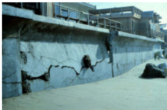
Figure 4. Failure of a seawall in northern Monterey Bay due to loss of supporting fill behind the wall.
