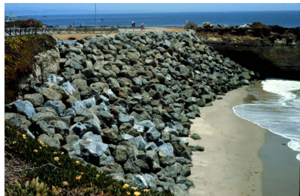
Figure 9. Emplacement of riprap impounds or covers significant beach area.
