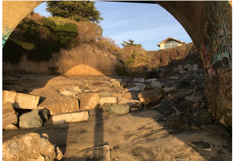
Figure 3 Concrete debris east of bridge.
