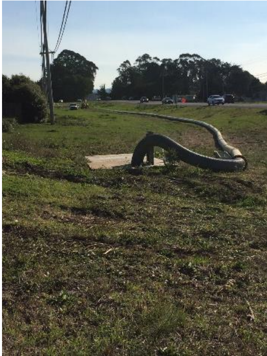
Bypass Valve Vault STA 39+00
