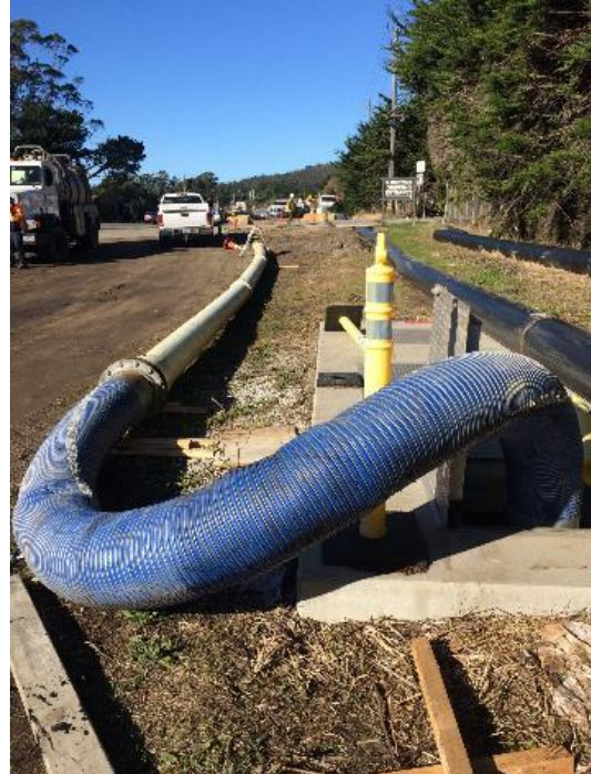
Bypass Valve Vault STA 74+00
